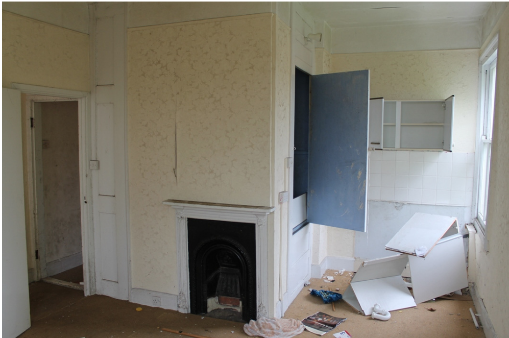
Plate 13 Living room, with the inserted stud wall to the left, the register grate and the cupboard above the stairs - view south-east
