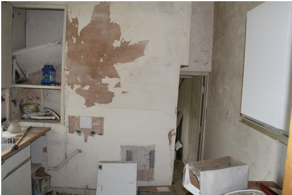
Plate 8 The service wing, showing the kitchen with its blocked fireplace and the inserted phase 3 doorway – view north-west
