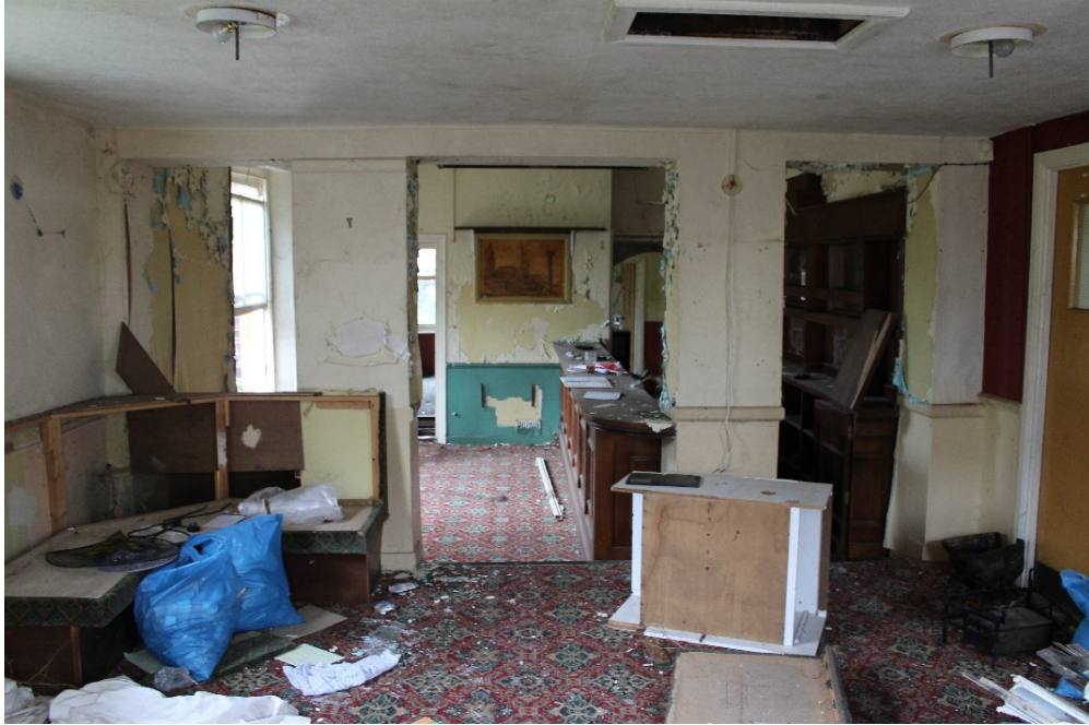
Plate 5 Interior of the bar, seen from the phase 2 extension looking into Wright Villa – view north-west
