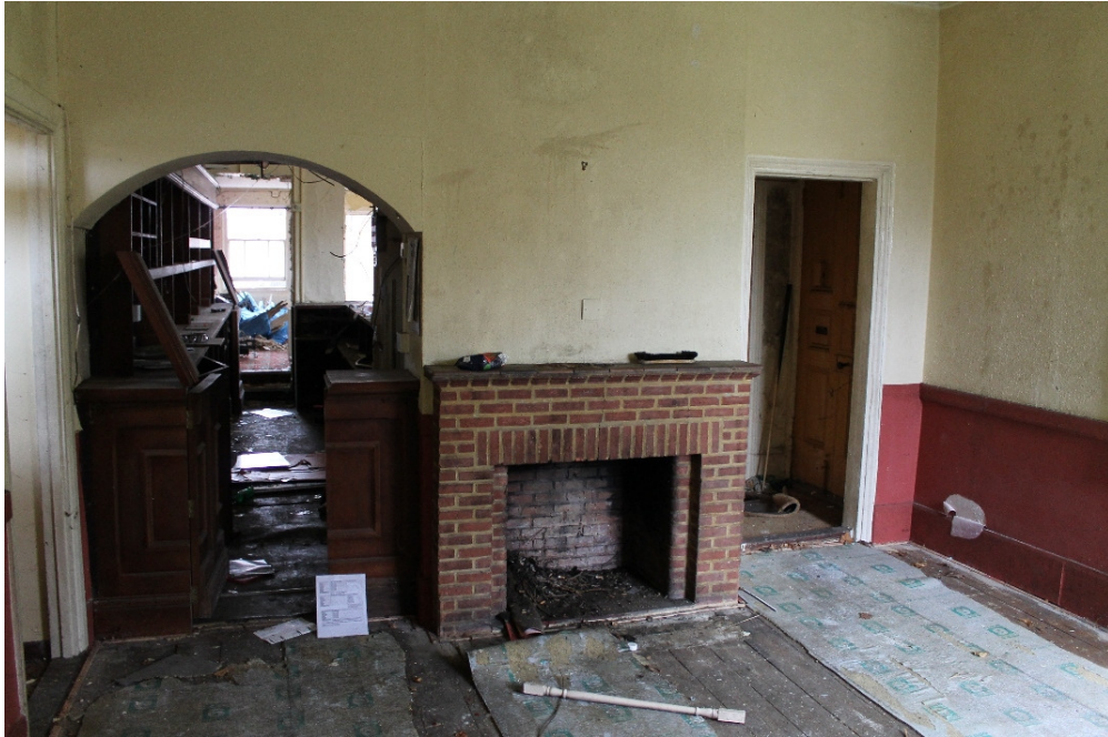
Plate 7 The back bar, with rebuilt fireplace and exposed original floorboards – view south
