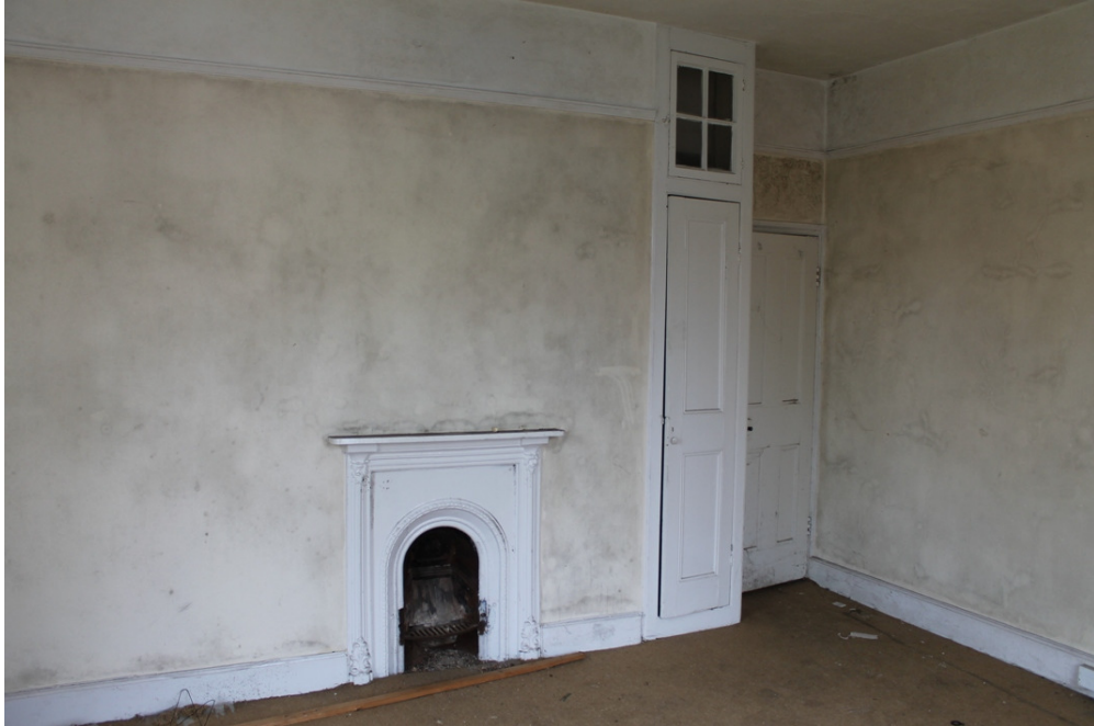
Plate 12 Bedroom with register grate, picture rail, later fitted cupboard and original door – view north-east
