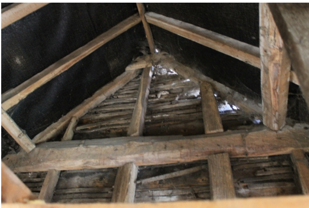
Plate 9 The interior of the north gable with original studs above and below a collar beam and the original purlins and rafters - view north
