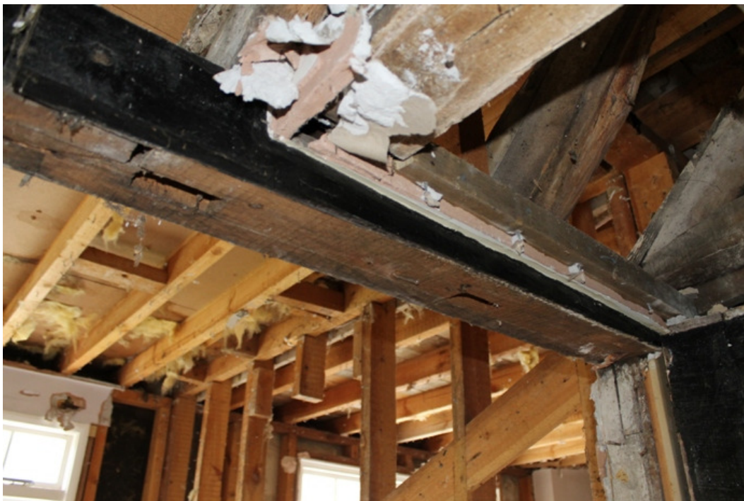
Plate 8 Mortices for removed studs in underside of wall plate with bladed scarf joint to the left – view south-east
