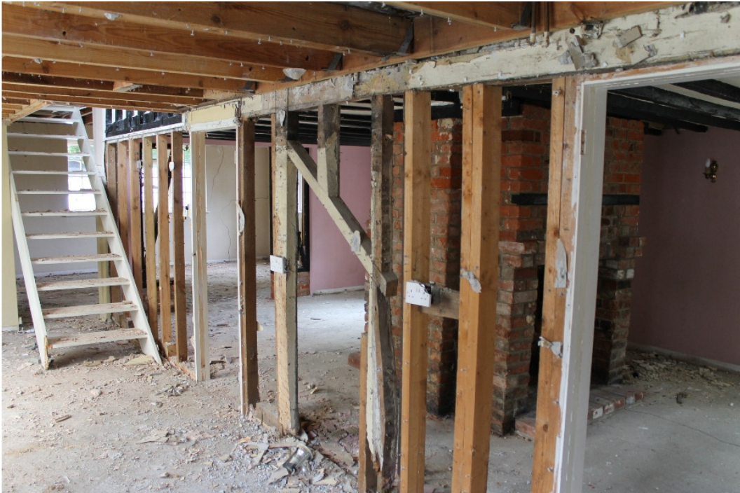
Plate 2 The exposed frame of the east wall, with the surviving girt, main post, studs and brace – view south-west
