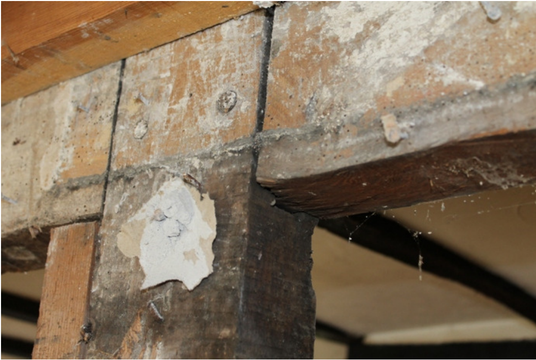
Plate 3 Girding beams single-pegged to main post, with carpenter's mark (II) at the top of the post – view south-west
