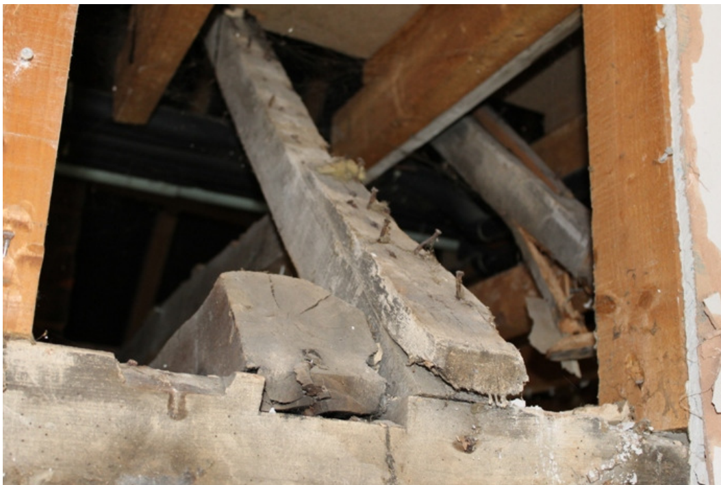
Plate 10 Original rafter with firing piece nailed to it and end of relocated tie beam – view north-west
