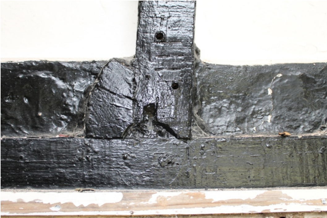
Plate 12 Example of a carpenter's mark (III) on the base of a stud in the east wall of the first floor frame, with the butt end of a floor joist carried on the girt - view west
