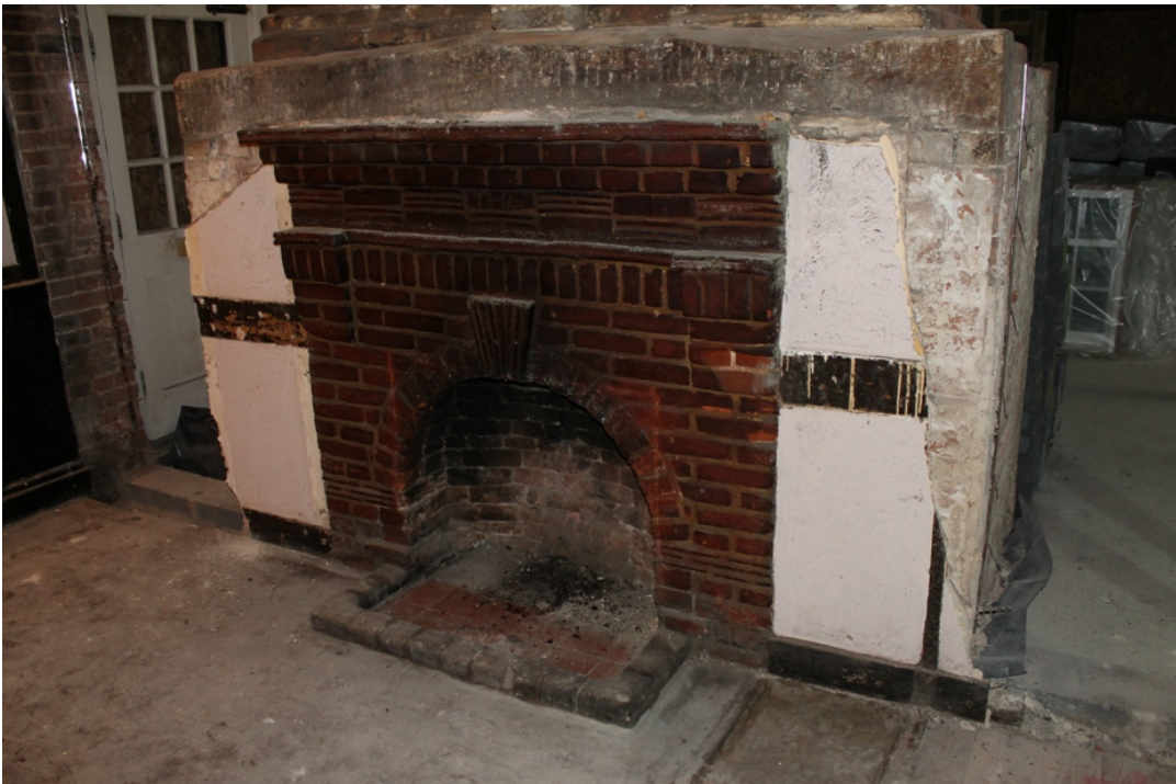
Plate 10 Art Deco fireplace inserted to the Phase 1 chimney, with Phase 5 render and mock timber framing – view south-west
