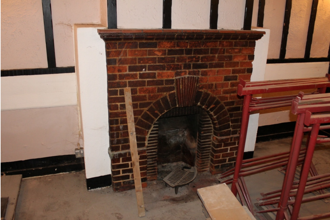
Plate 11 Art Deco fireplace on Phase 2 chimney breast at east end of the lounge – view south-east
