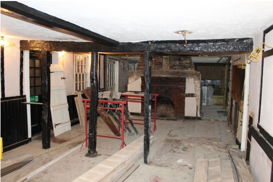
Plate 8 The bar viewed from the lounge, showing the large-section lateral bridging beam with re-used posts and one of the chamfered longitudinal bridging beams – view north-east
