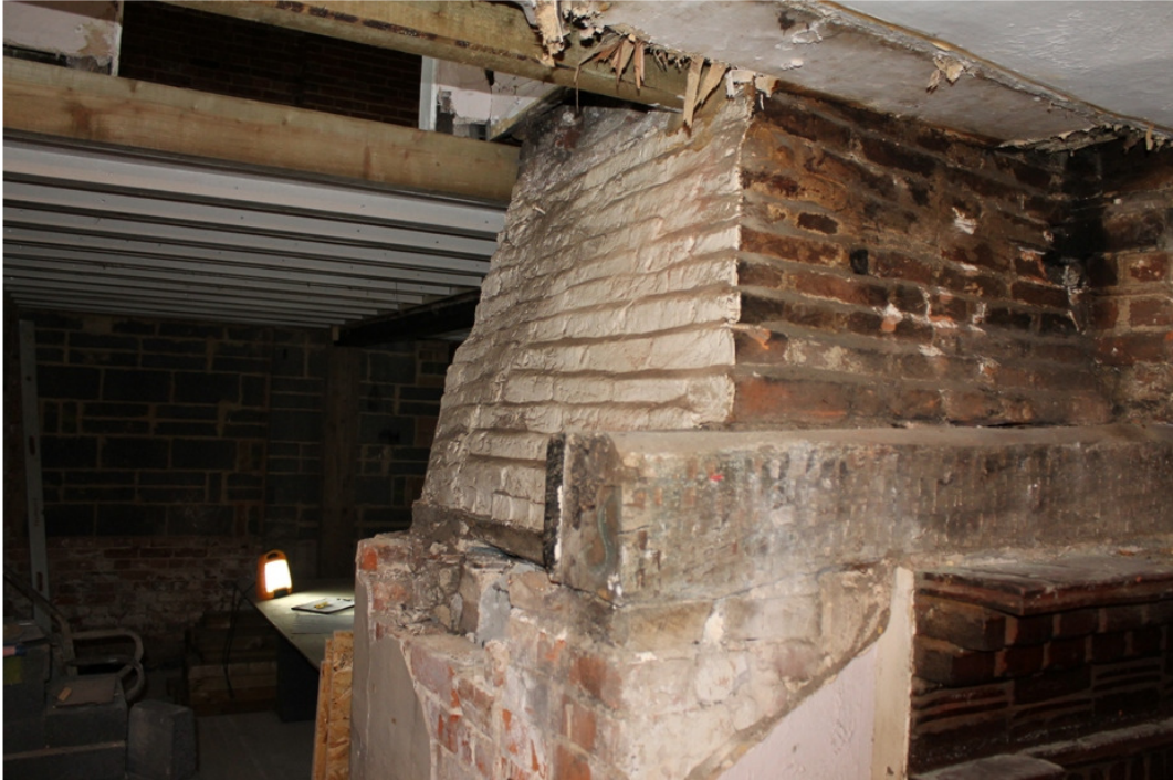
Plate 9 The original Phase 1 chimney between the dining area and the bar, with the stepped brickwork of the stack and the cambered timber mantel - view north-west.
