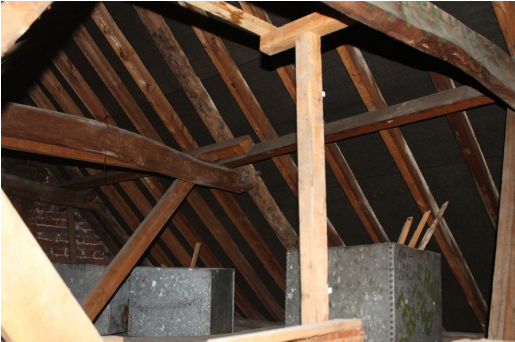
Plate 22 Detail of the roof timbers, showing original Phase 1 principal rafter and collar and modern inclined queen post, purlin and common rafters – view south-east
