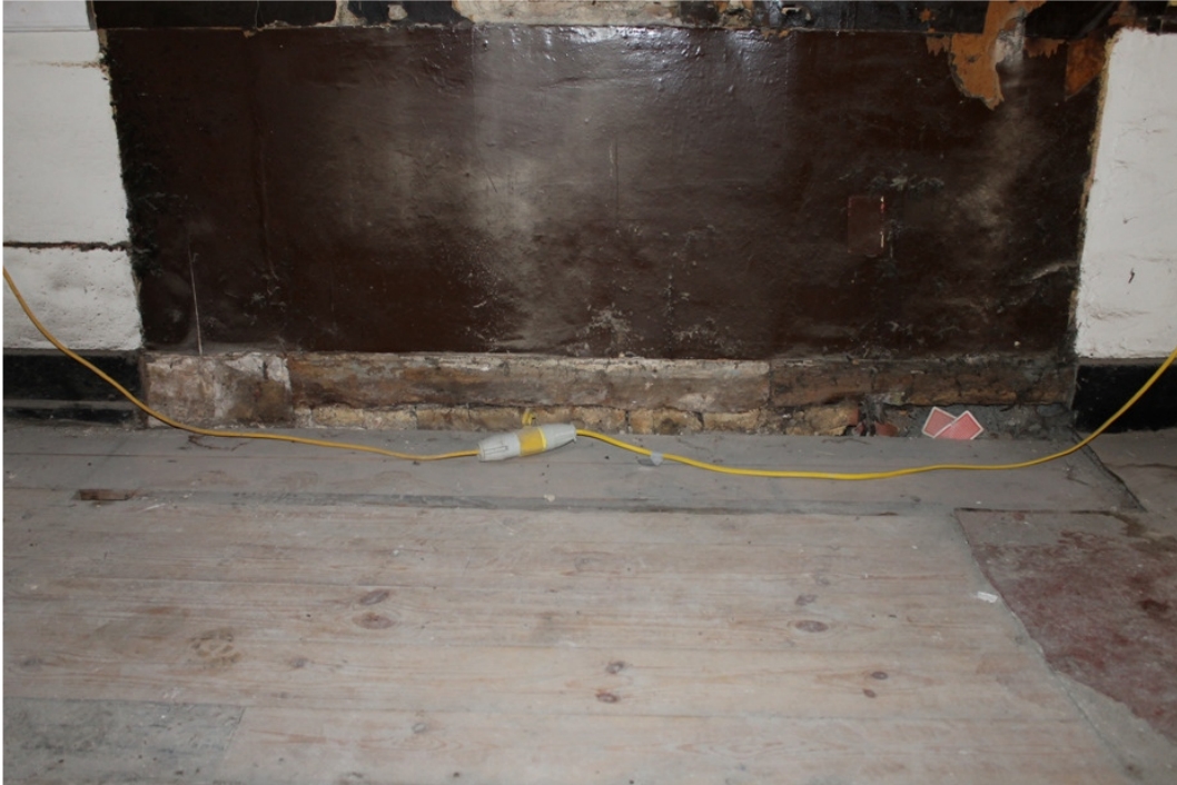
Plate 7 Phase 1 sill beam and brick plinth exposed in rear wall of bar - view north
