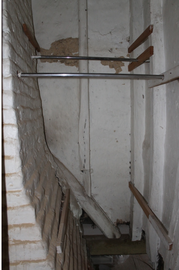
Plate 17 Cupboard formed from the space besides the Phase 1 chimney stack, exposing the original framing – view west
