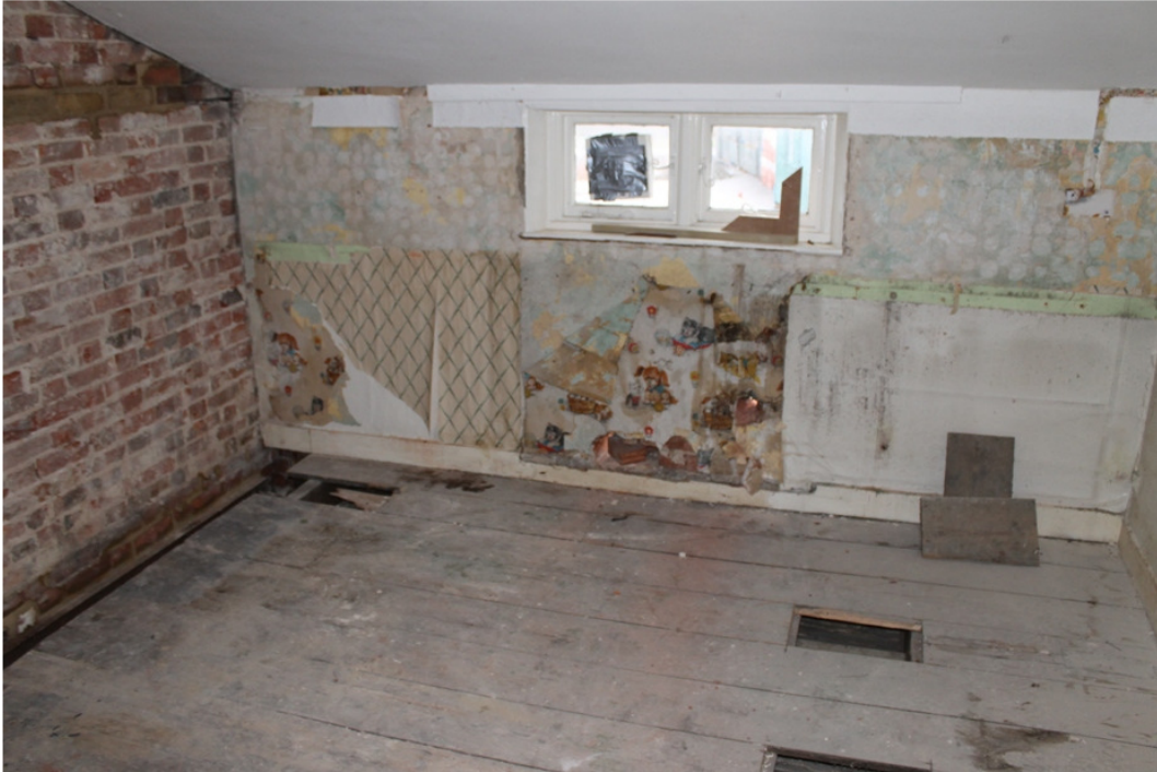
Plate 19 Bedroom 4, possibly intended as a nursery or child's room, with sloped ceiling and narrow wooden-framed casement windows – view north
