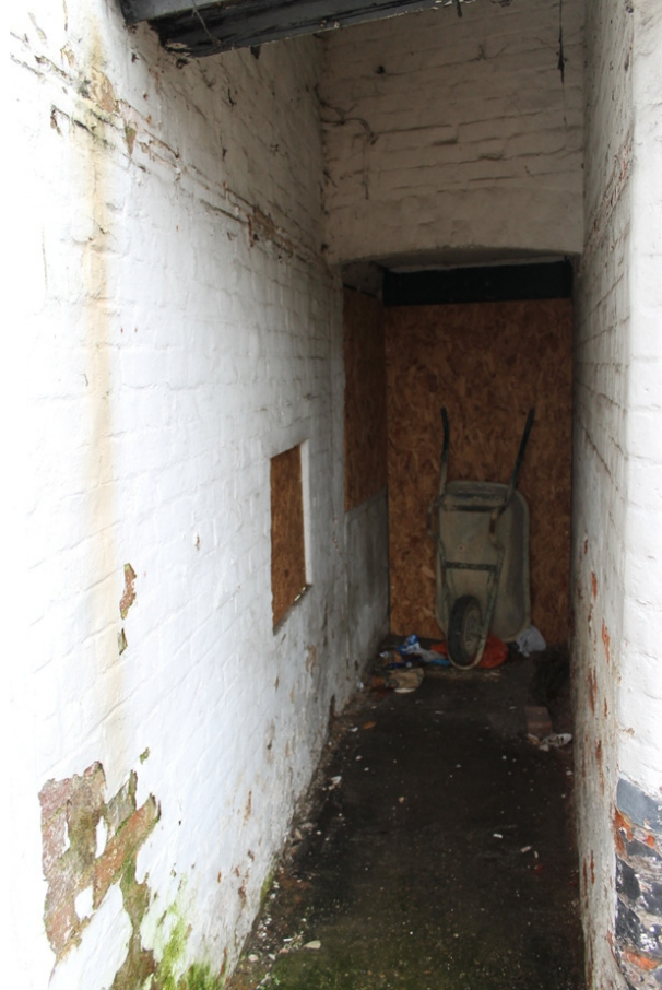
Plate 13 Phase 4 passage way leading from yard into Phase 3 extension, showing the arch for the original doorway to the extension – view south-east
