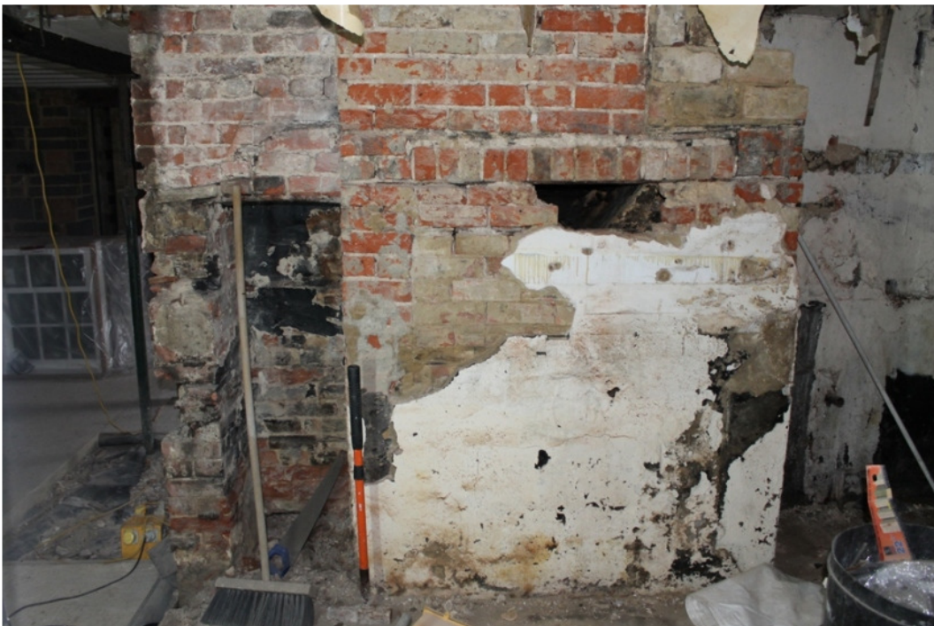
Plate 14 Phase 3 kitchen, showing blocked fireplace with warming oven to the left - view west
