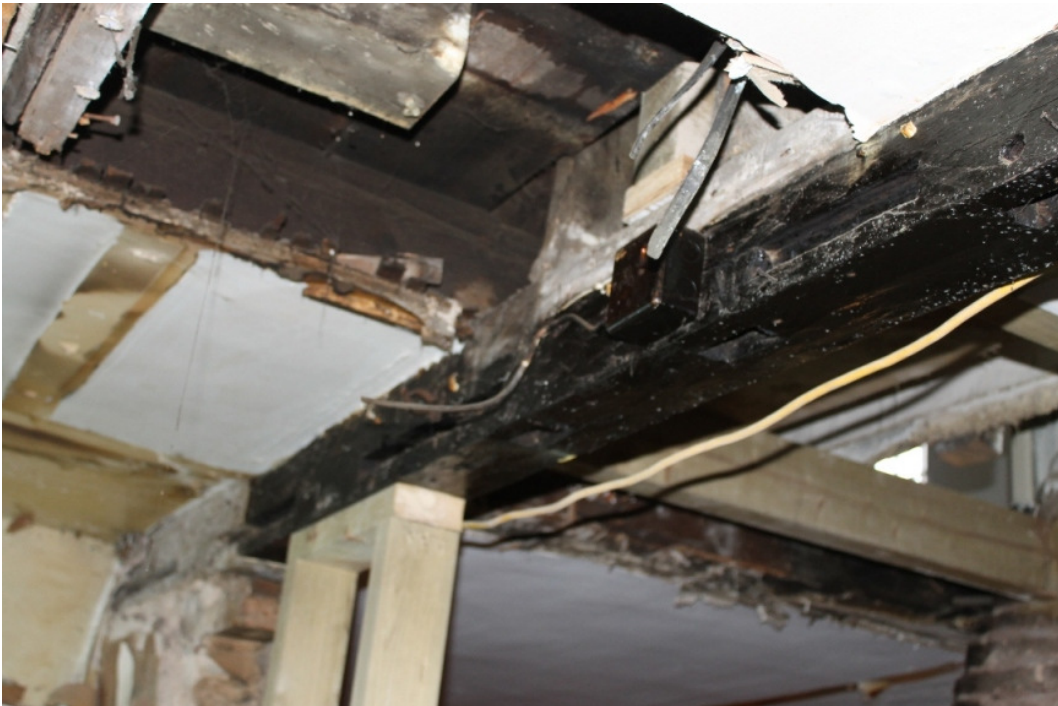
Plate 6 Mortices in the external face of the Phase 1 girding beam, indicative of a structure that once projected from the rear of the main range - view south-east
