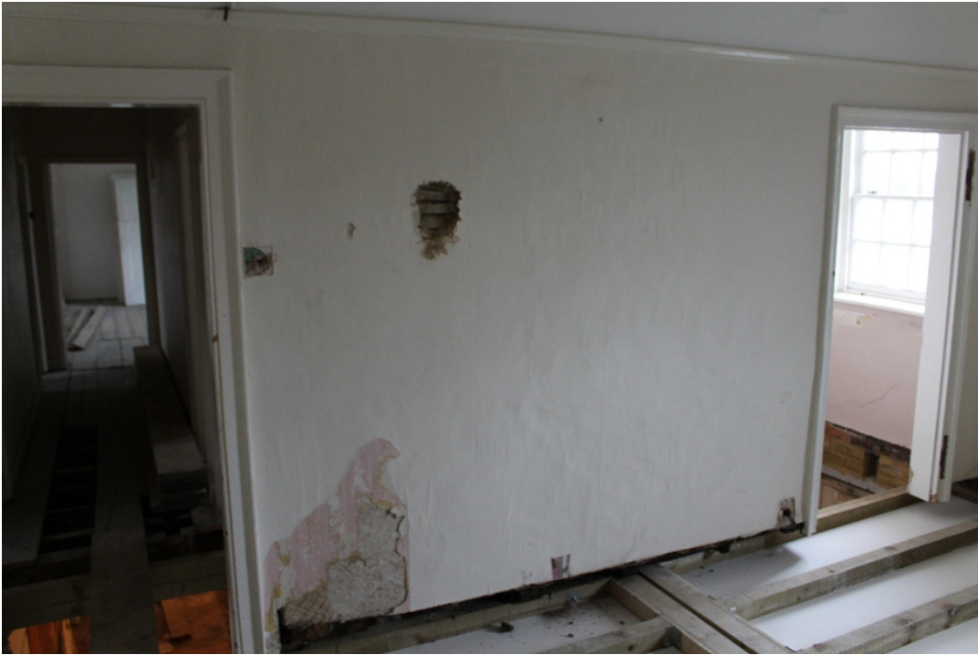
Plate 16 Bedroom 1, showing dividing wall to chimney stack, with lath and plaster over original Phase 1 timber framing - view south-east
