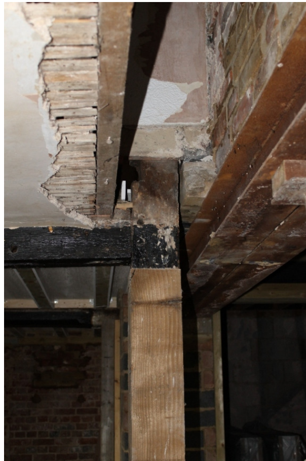
Plate 4 The west wall of the main range, showing the surviving timber frame of Phase 1 inside the brick skin of Phase 2 - view north
