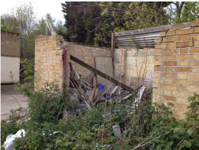
Plate 11: view south-west into interior of derelict 1956 building B
