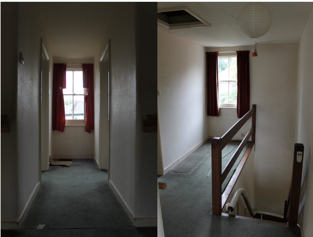
Plate 10 Staggered first floor landings showing 20th-century stairs in reversed position - view north-east and south-west.
