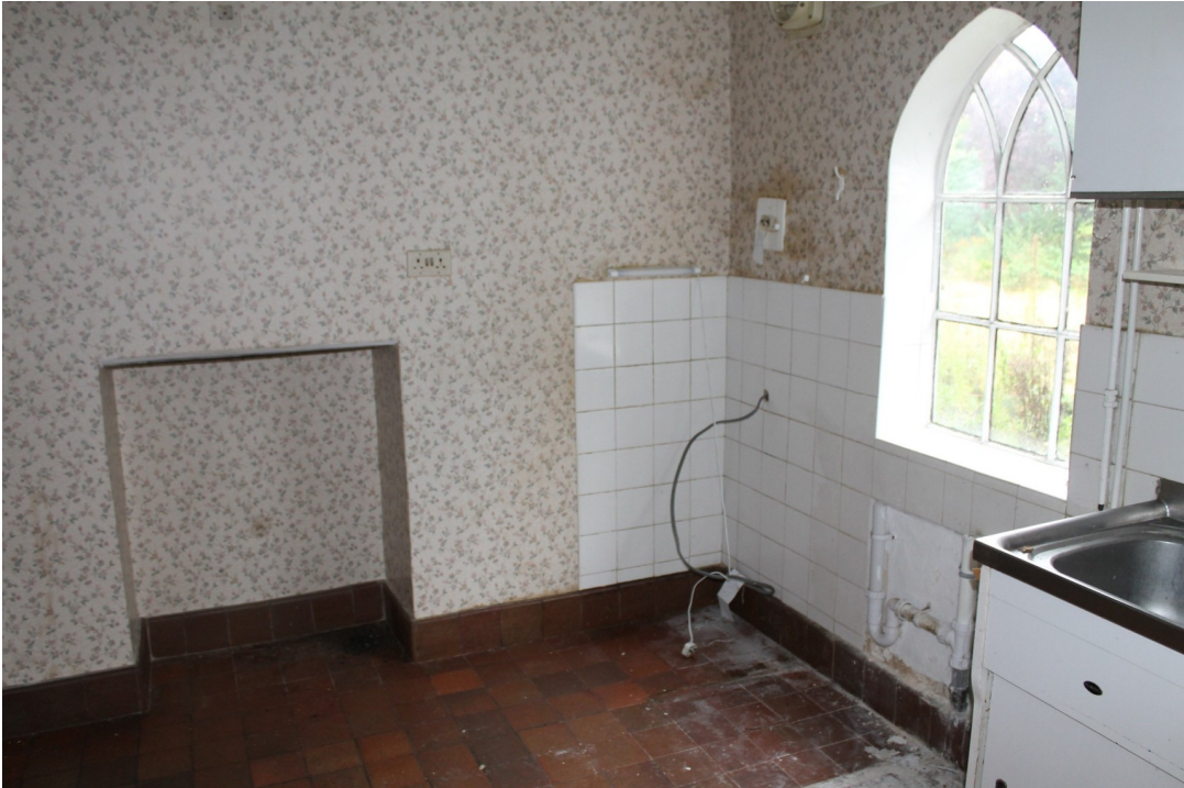
Plate 9 Interior of kitchen with 20th-century alterations and original fireplace opening - view north-east.
