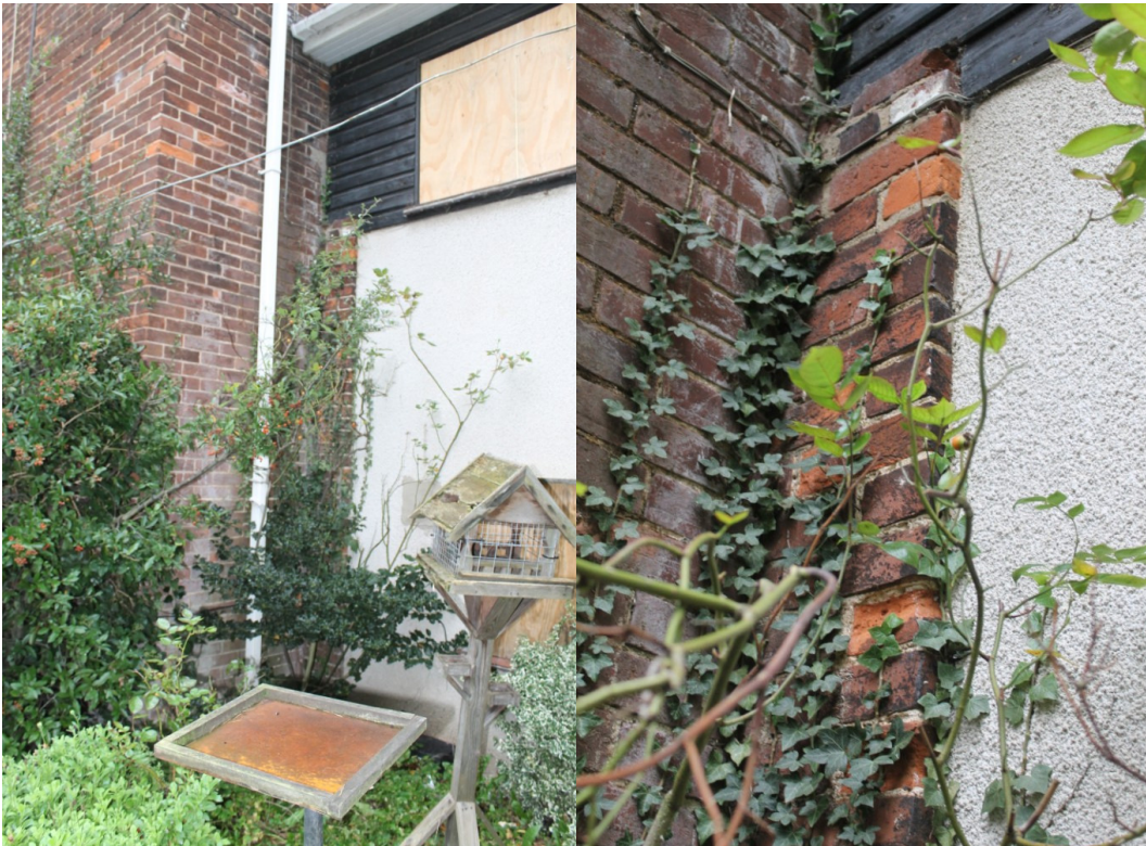
Photographs 6 & 7 (Left) Single-storey stub of brickwork between the main range and the 20th-century extension, probably all that survives of the original 19th-century service wing but potentially part of an earlier cottage. (Right) Detail of the brickwork – view north.
