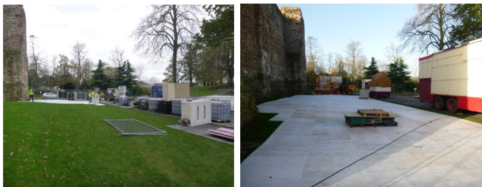
Photographs 3-4 North side of Colchester Castle during and after construction of the temporary flooring, looking W
