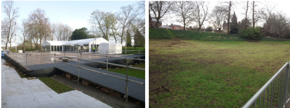
Photograph 11-12 East side of Colchester Castle with raised floor for ice rink and coffee hut/skate exchange marquee, looking NE and east side of Colchester Castle after removal of Winter Wonderland and raised floor, looking SE.
