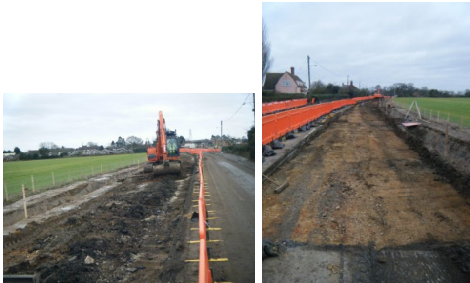
Photographs 5-6 Removal of pre-existing surface, looking S, and stripping to natural, looking N
