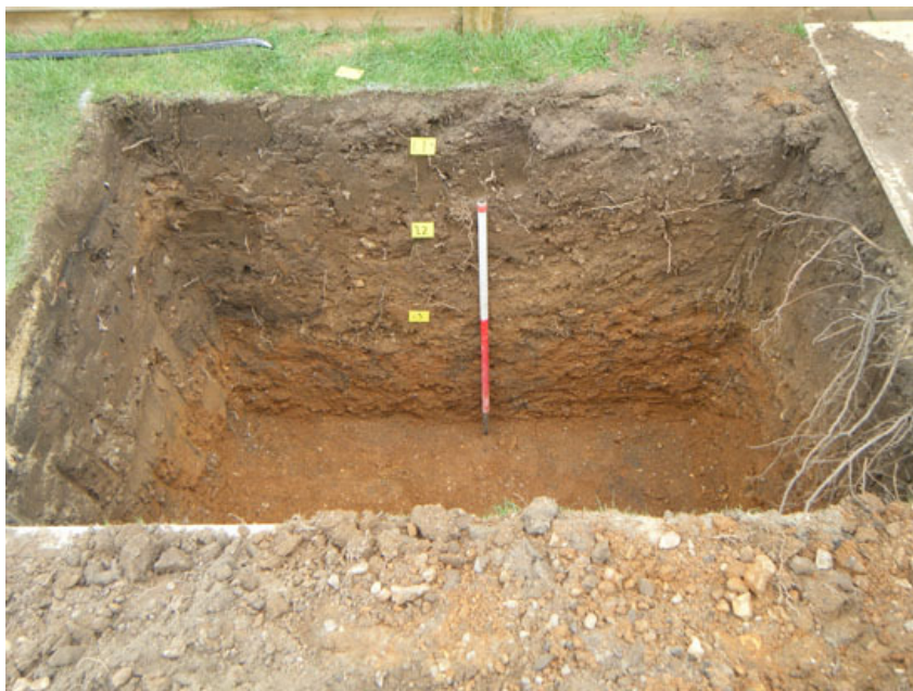
Photograph 2 Soakaway, looking E
