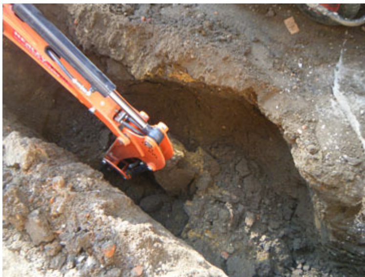
Photograph 1 Feature F1 after collapse of section, looking S
