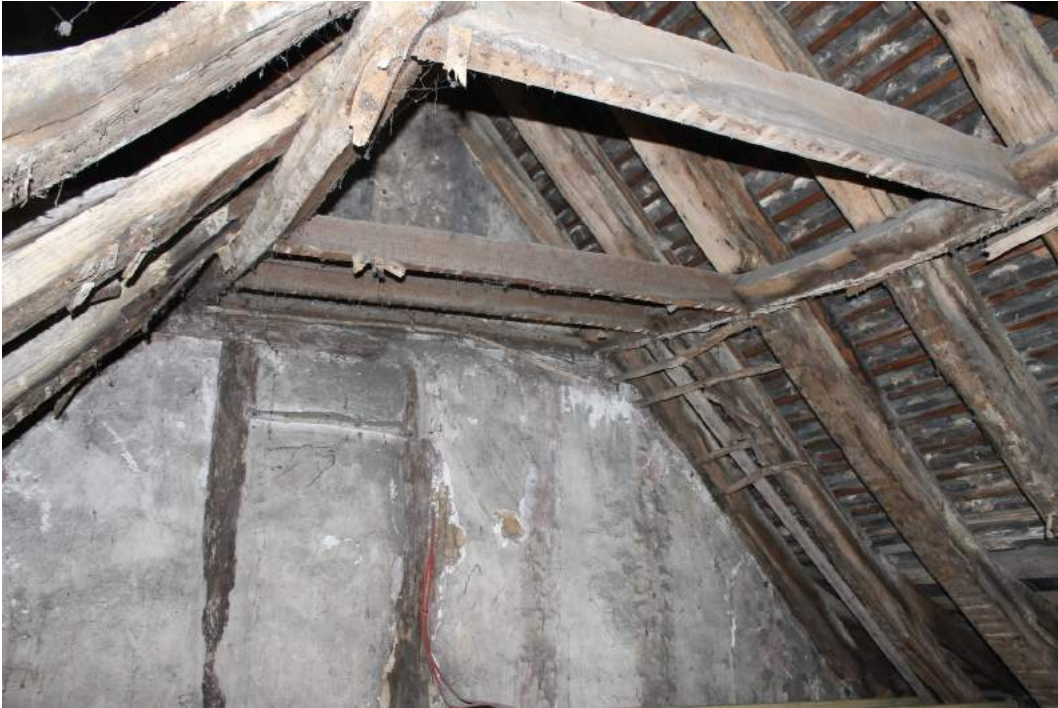
Photograph 10 Interior of the roof space looking towards the gable frame with the original wattle and daub infill panels – view north
