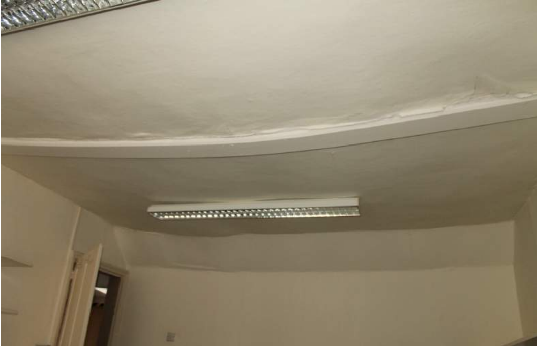
Photograph 4 Sagging ceiling, with bowed bridging beam in first floor room – view west
