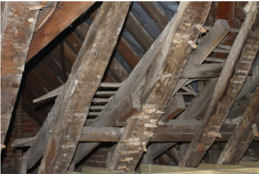
Photograph 16 Longer sprockets at the feet of the rear side rafters, allowing the roof to flare out over the possible earlier 19th-century extension, with the machine-cut timbers of the 19th-century extension behind – view north-west
