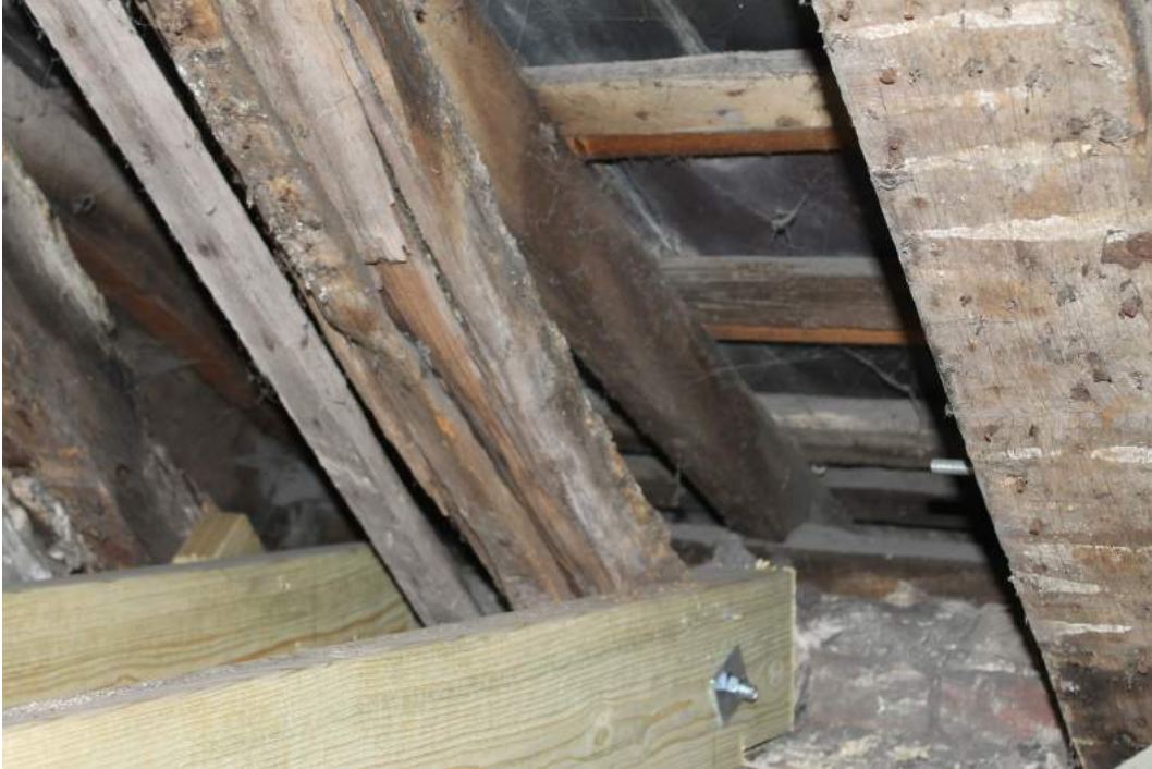
Photograph 15 Sprockets at the feet of the street side rafters, allowing the roof to flare out over the brick facing – note the slate roof covering above the battens – view north-east
