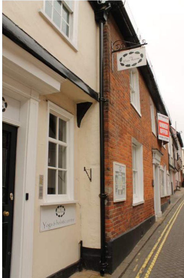
Photograph 2 Brick facing to No. 11 with the jettied first floor of No. 12 showing what is concealed by the brick facing – view north-west
