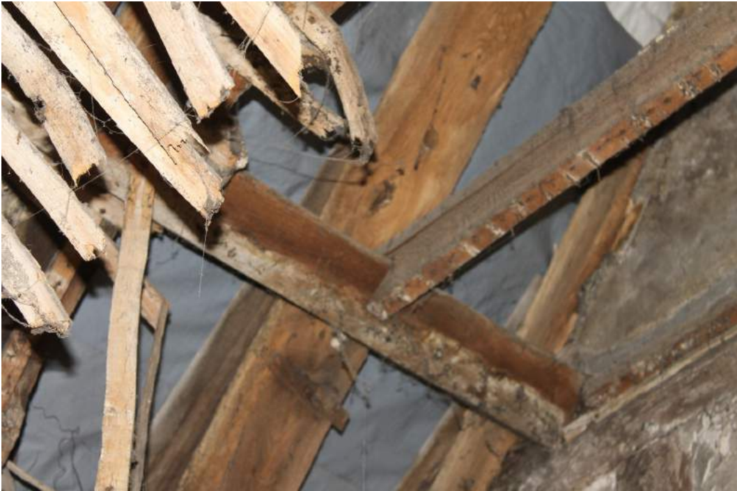
Photograph 8 Machine-cut collar with birdsmouth scarf joint to the purlin, to which the earlier lath and horsehair plaster ceiling was nailed – view south-east
