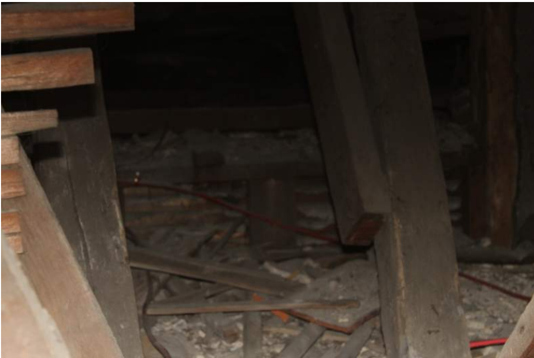
Photograph 5 Interior of roof space showing debris from earlier ceiling on top of existing ceiling – view east
