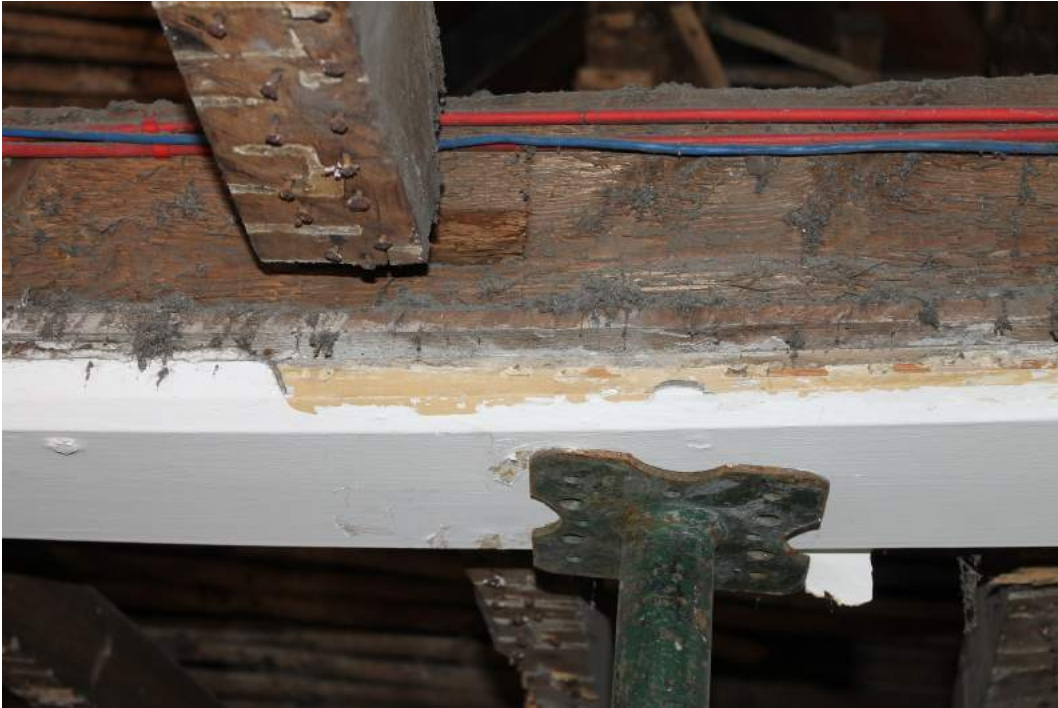
Photograph 7 Staggered mortises for the 19th-century ceiling joists in the bridging beam – view west
