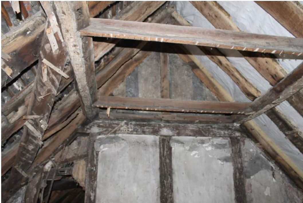
Photograph 9 Interior of the roof space looking towards the central cross frame with the original wattle and daub infill panels. The wind brace can be seen on the left, below the street side purlin which displays toolmarks on its underside and empty mortises, indicating it is a re-used timber – view south
