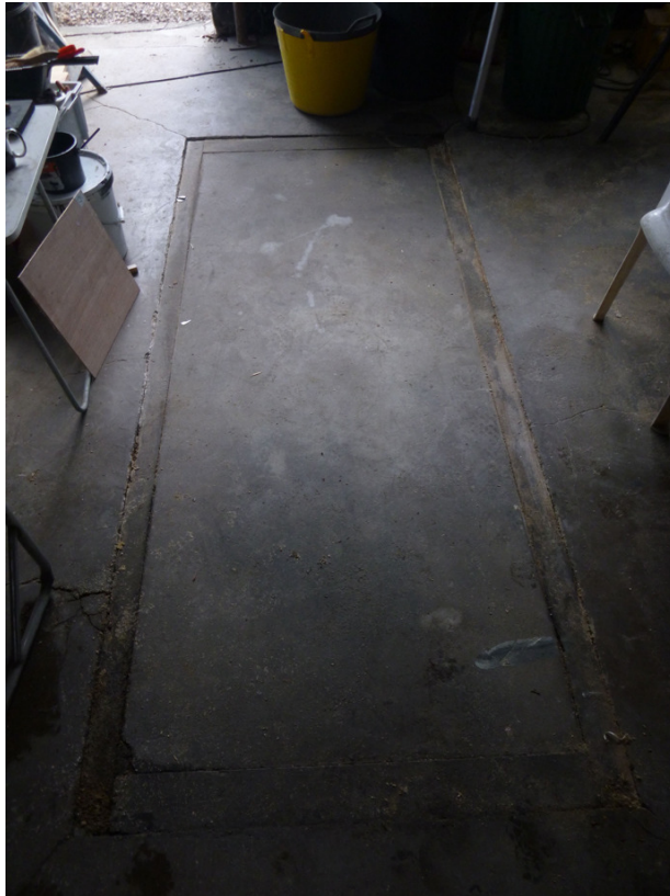
Photograph 12 Backfilled and concreted over inspection pit in main building – shot taken facing east.
