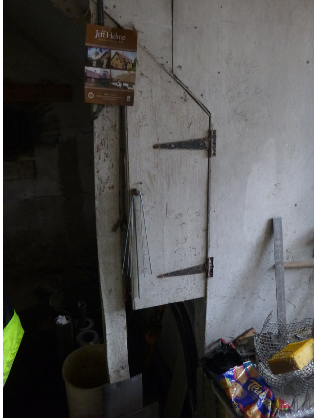
Photograph 11 Hatch in-between wall and supporting post in north wing – shot taken facing north.
