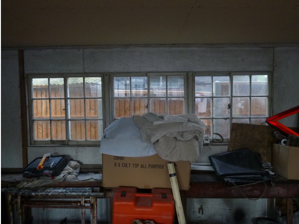
Photograph 7 Interior shot of three sliding casement windows on west elevation – shot taken facing west.
