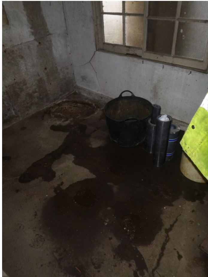
Photograph 10 Scars on floor of concrete in north wing, showing location of possible machinery – shot taken facing north-east.
