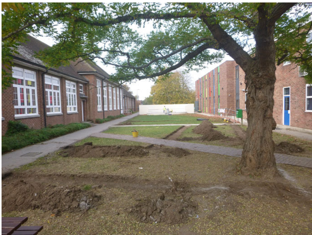
Photograph 10 Full excavation of line of Roman temple walls ready for the paving slabs to be laid, looking W
