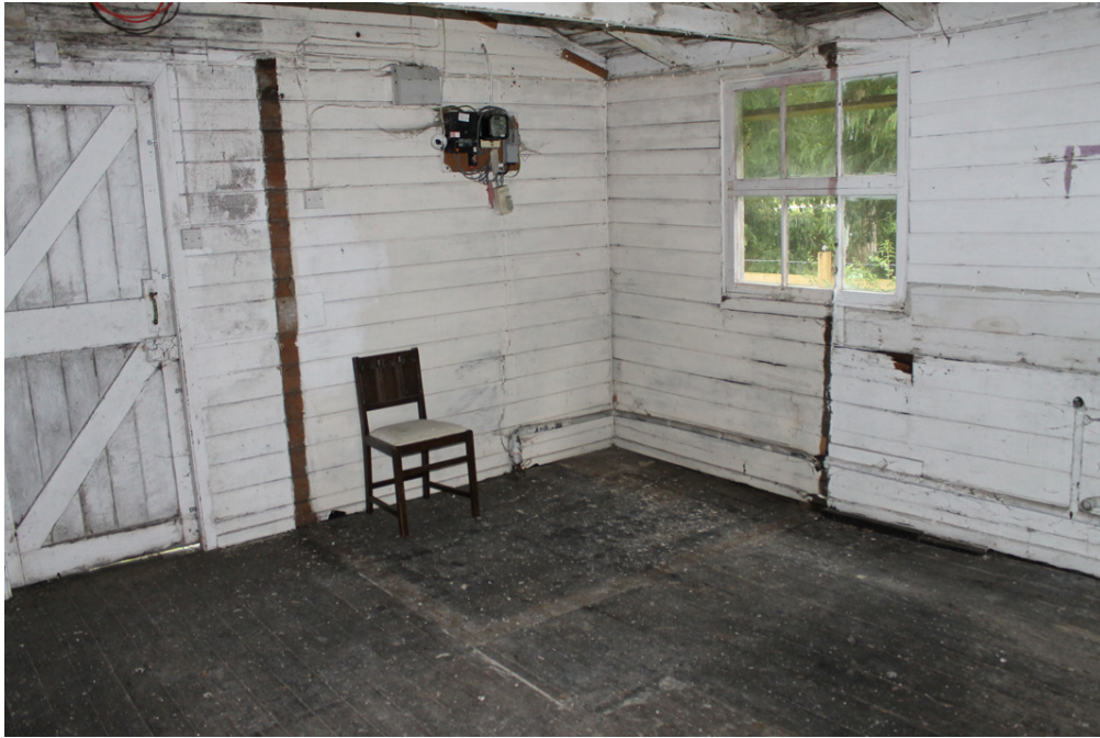
Photograph 7 Recently removed division in the south-east corner of the Hall. Shot taken facing south-east.
