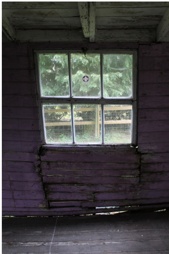
Photograph 8 Detailed shot of one of the six-light windows on the southern elevation. Photograph taken facing south.
