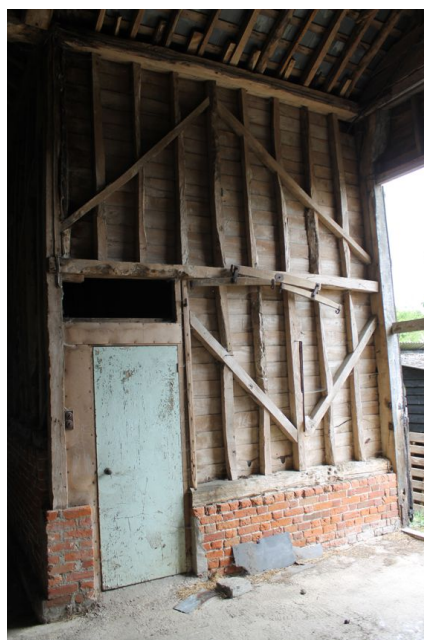
Photograph 7 South-east elevation of the midstrey. Machine-cut timber visible as primary bracing. Photograph taken facing south-east.
