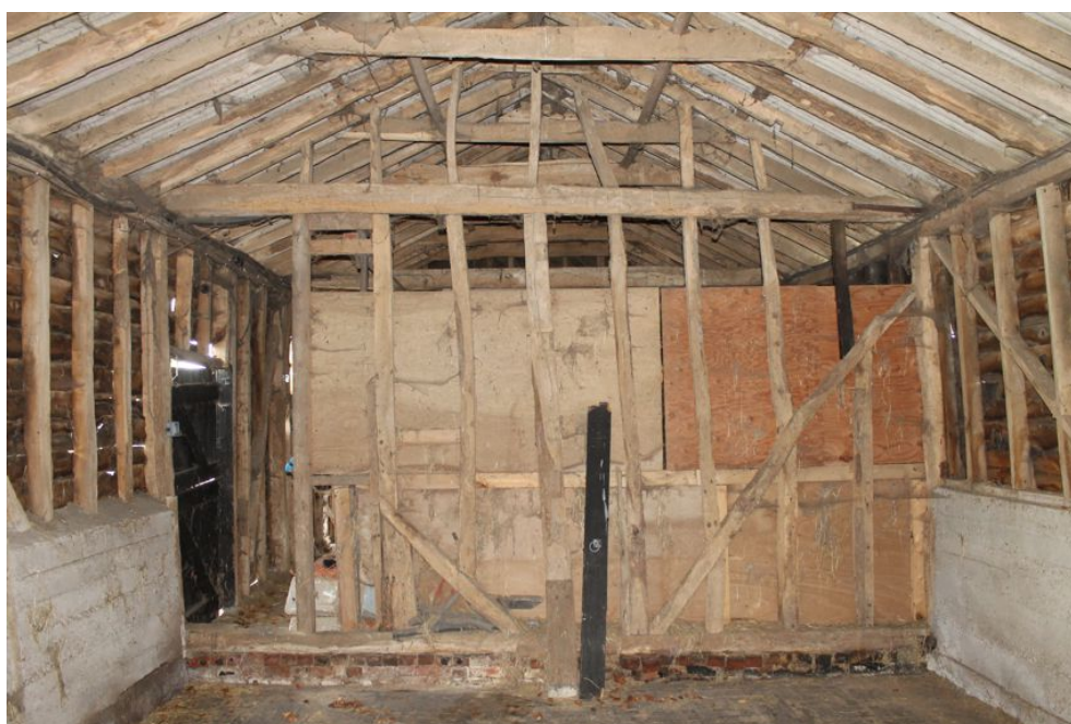
Photograph 20 Dividing wall in the centre of Building C. Photograph taken facing south-west.
