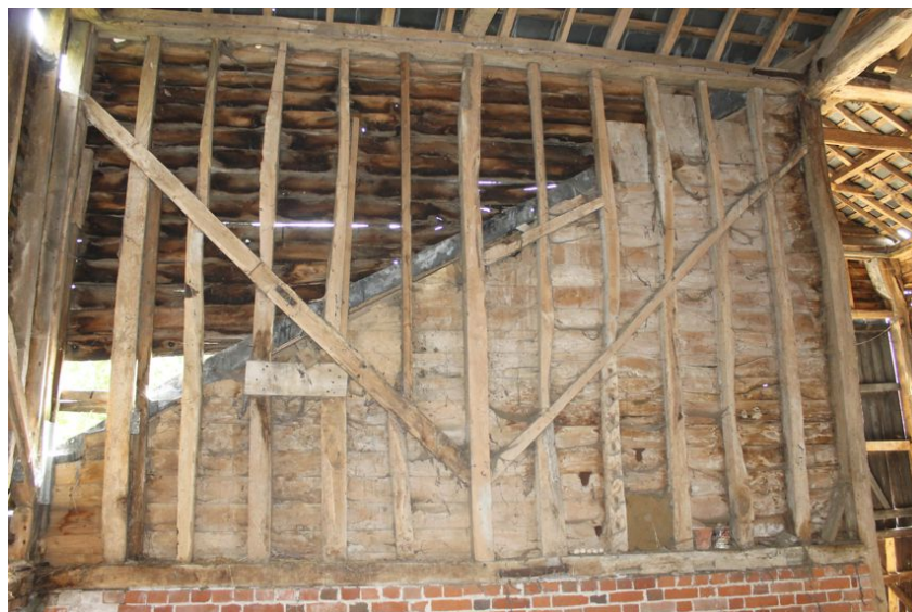
Photograph 6 South-west elevation of bays 4 and 5. Re-used primary bracing visible, as well as old weatherboarding. Photograph taken facing south-west.
