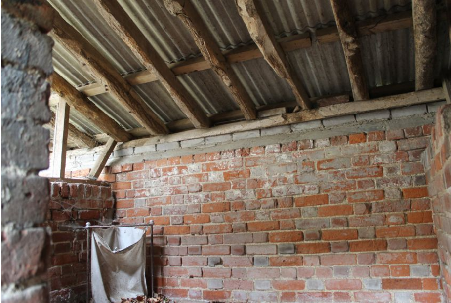
Photograph 35 Interior of original half of Building H, showing brickwork and rafters. Photograph taken facing east.
