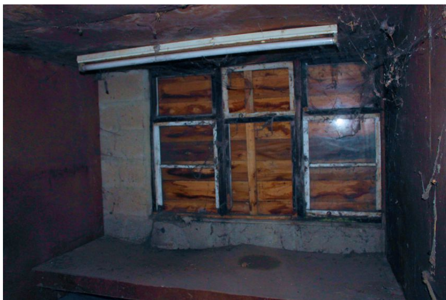
Photograph 30 Interior shot of Building F, showing blocked modern window. Photograph taken facing south.
