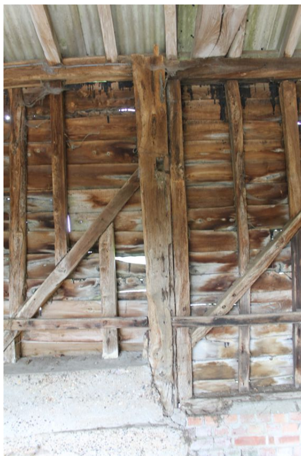
Photograph 27 Principal post in north-west elevation of Building D, with tenon set to one side visible at apex. Photograph taken facing north-west.
