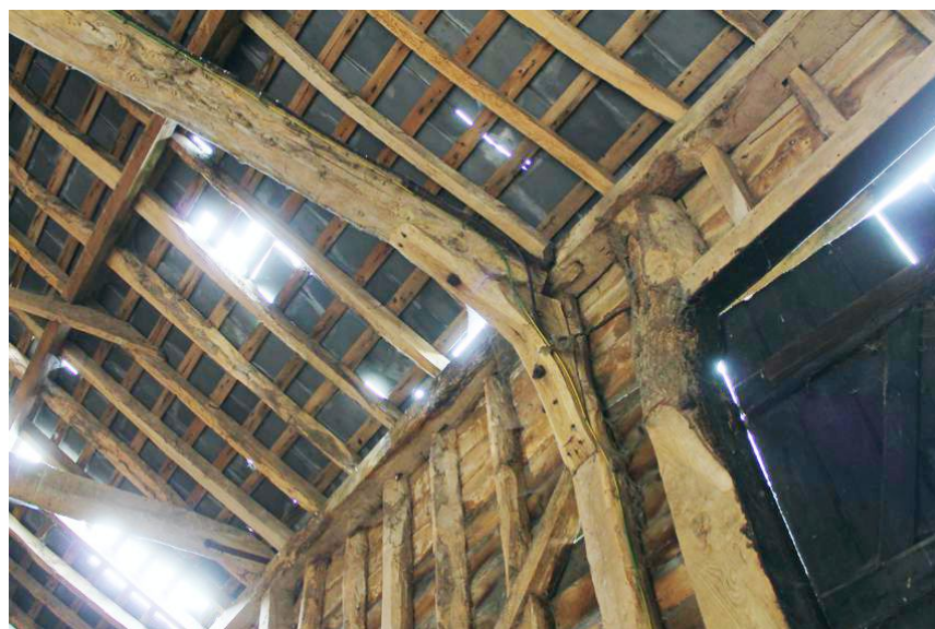
Photograph 12 Detailed shot of knee brace supporting tie-beam between bays 2 and 3. Photograph taken facing north.
