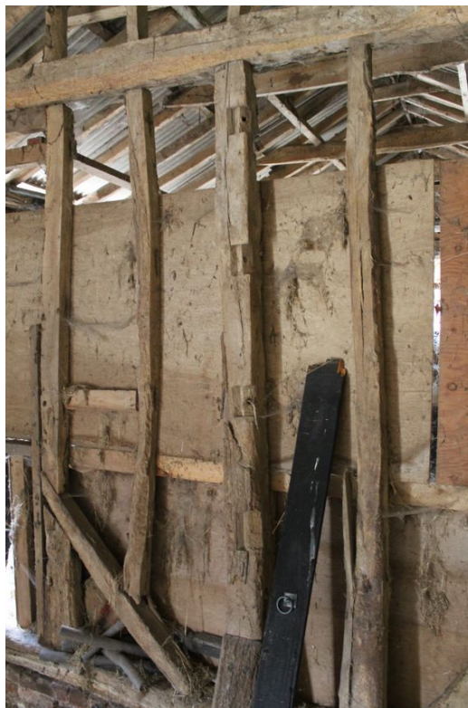
Photograph 21 Detailed shot of re-used intermediate post in dividing wall in the centre of Building C. Photograph taken facing south.
