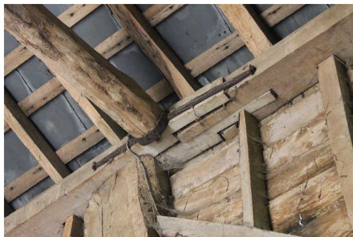
Photograph 10 Detailed shot of scarf joint in wall-plate on north-east side of bay 4. Photograph taken facing north.
