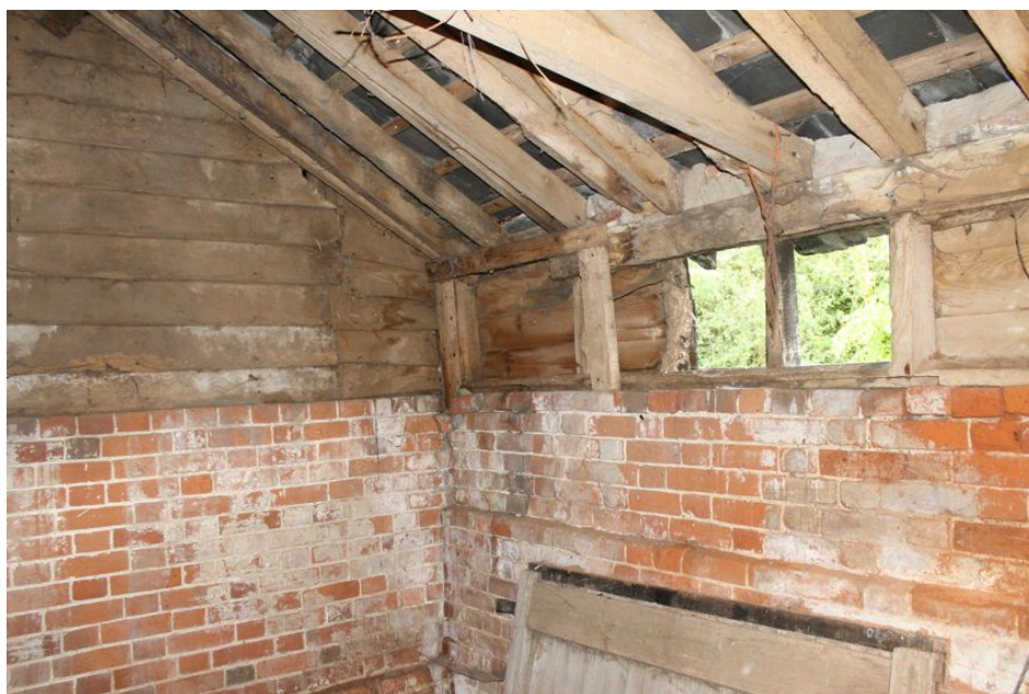
Photograph 33 Interior shot of Building G, showing timber-framing above wall. Photograph taken facing east.
