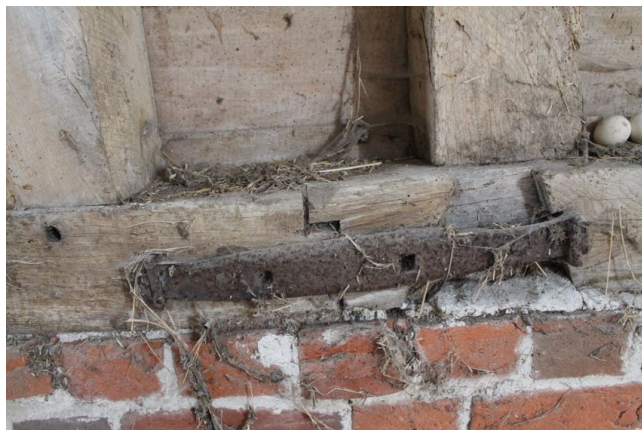
Photograph 9 Detailed shot of scarf joint in sill-beam on south-west side of bay 4. Photograph taken facing south-west.
