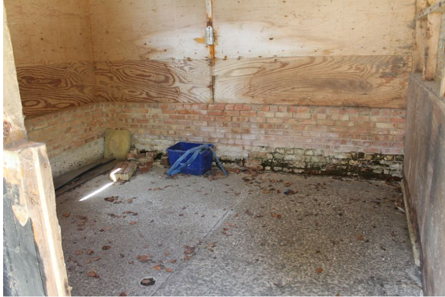
Photograph 18 Interior shot of Building B, showing different bricks visible in plinth. Photograph taken facing west.
