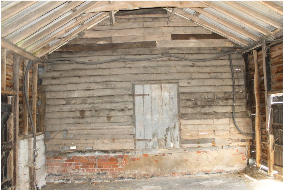
Photograph 25 South-west elevation of Building D, from inside Building C. Photograph taken facing north-east.
