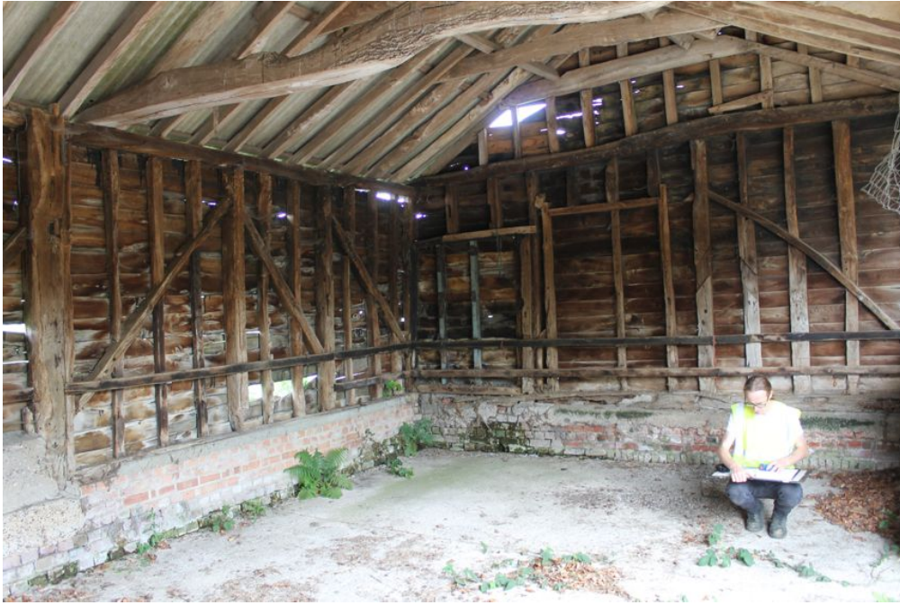
Photograph 29 Interior shot of Building D, with two modern timbers and possible blocked entrance visible in centre of photo. Photograph taken facing north.
