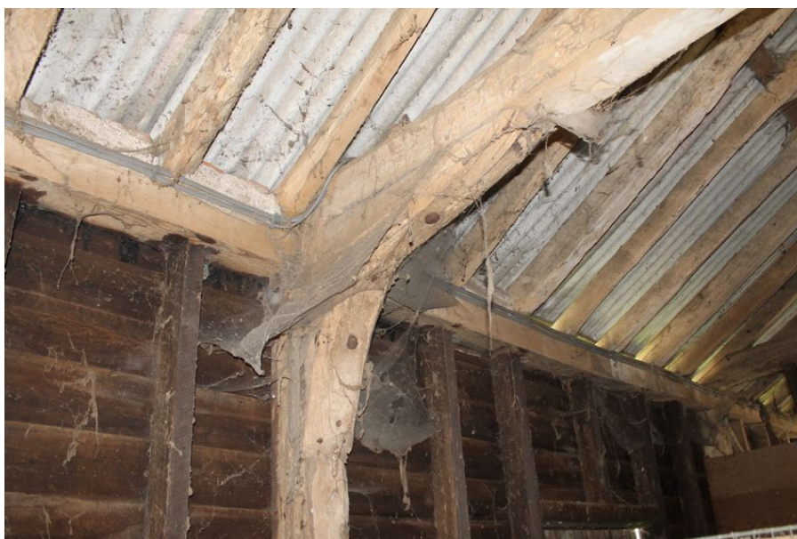
Photograph 23 Knee brace supporting tie-beam in Building C. Photograph taken facing north.
