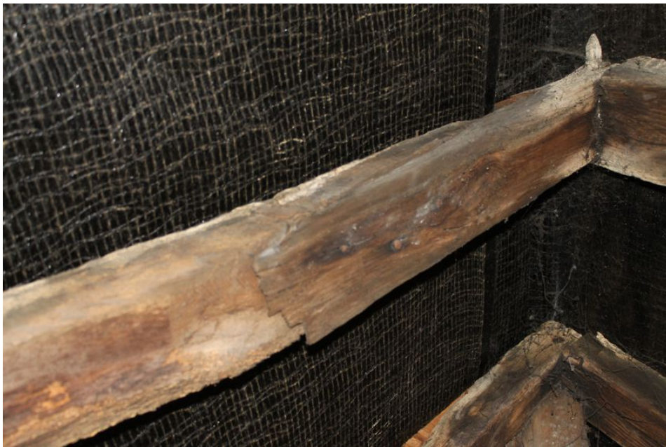
Photograph 24 Detail of rafters in Building A. Peg at apex visible, along with scarf joint/repair to rafter.
