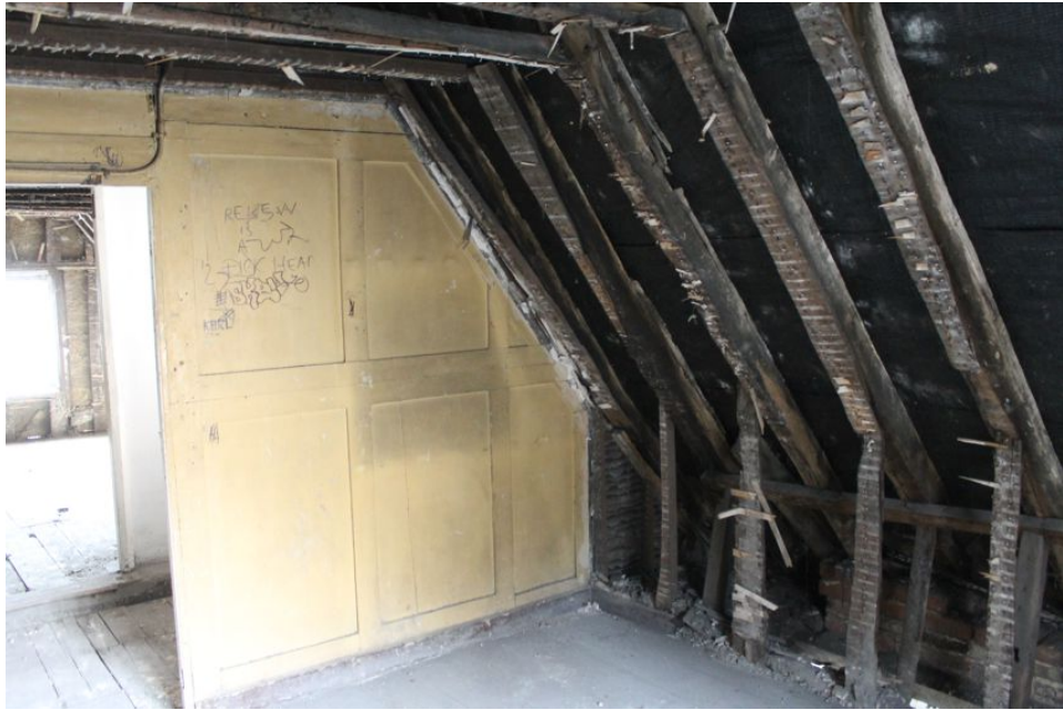
Photograph 34 East room on second-floor of Building A. smoke-blackened rafters visible. Photograph taken facing north-west.
