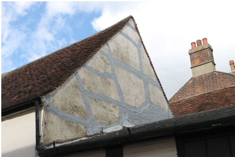
Photograph 38 Eastern gable-end of Building B, showing repairs to plaster. Photograph taken facing north-west.
