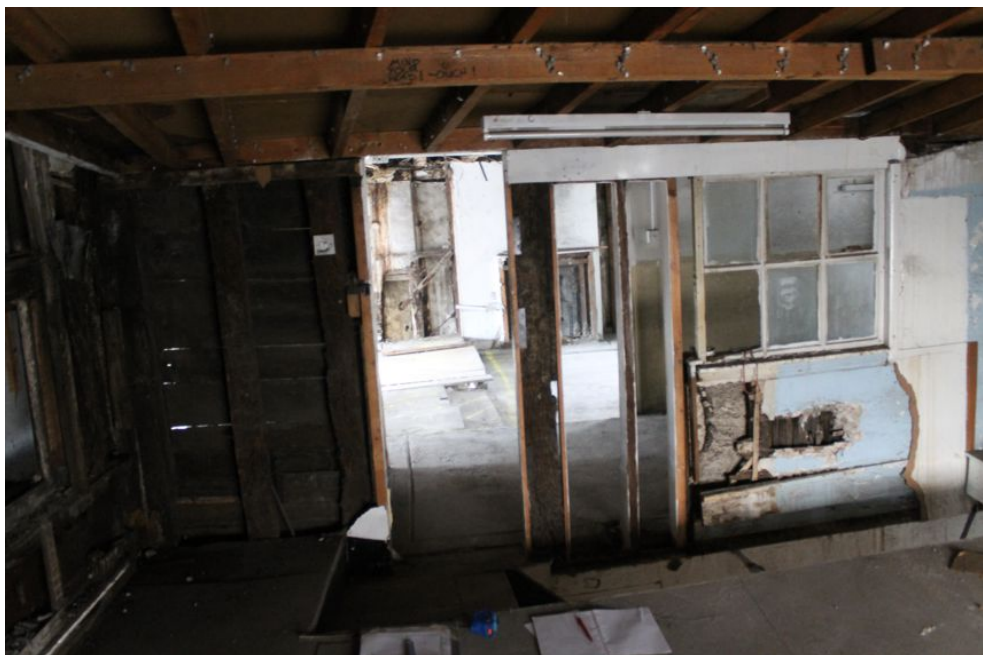
Photograph 4 Southern exterior elevation of the first-floor of Building A, with exposed lath and plaster below inserted window. Photograph taken inside Building C, facing north.
