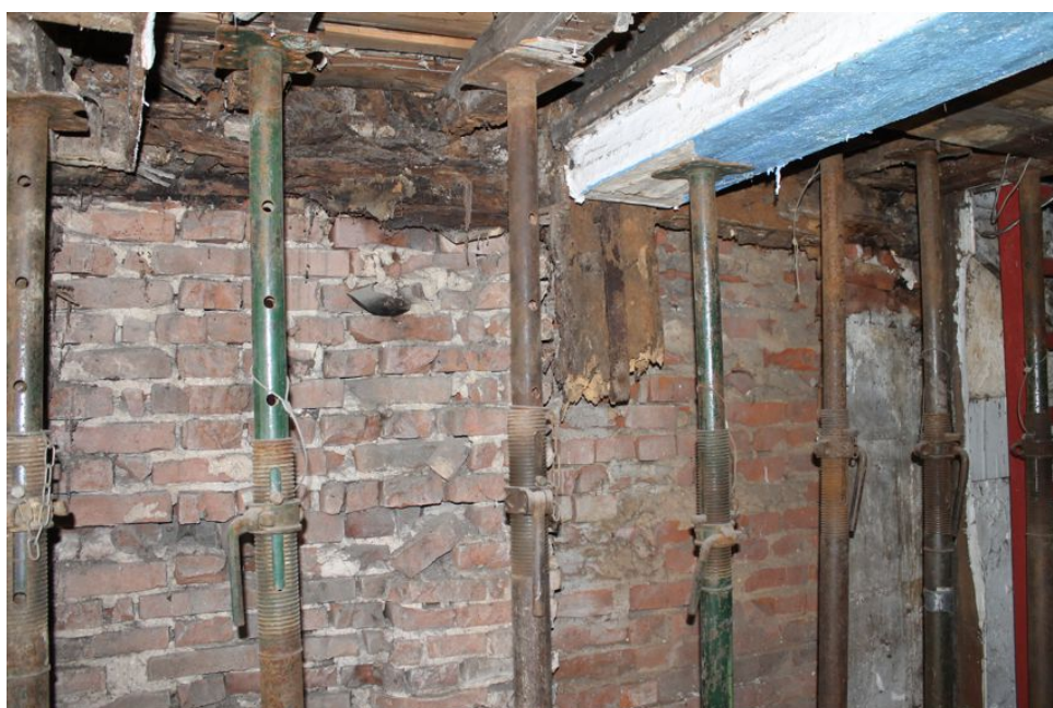
Photograph 10 Remains of principal-post on ground-floor on the northern elevation of Building A. Underpinning of girder-beam by brickwork also visible. Photograph taken facing north.
