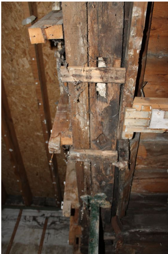
Photograph 13 Underside of girding-beam on eastern side of Building A. Diamond window mullions visible.
