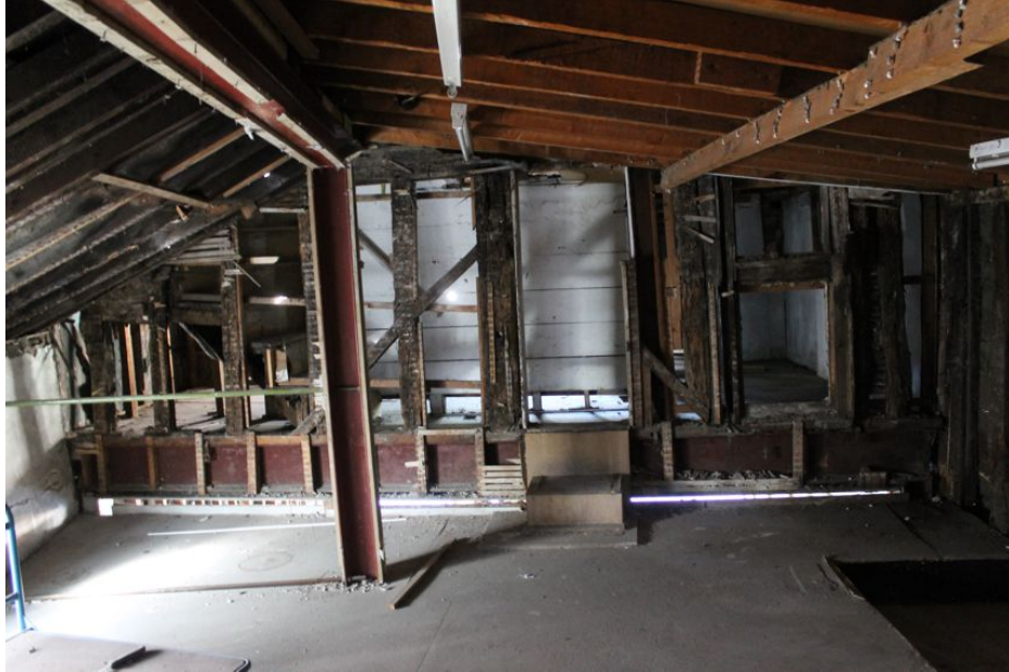
Photograph 39 Eastern elevation of exterior of first-floor of Building B, showing inserted doorway and window-frame. Also visible is metal beam supporting raised first-floor. Photograph taken facing west.
