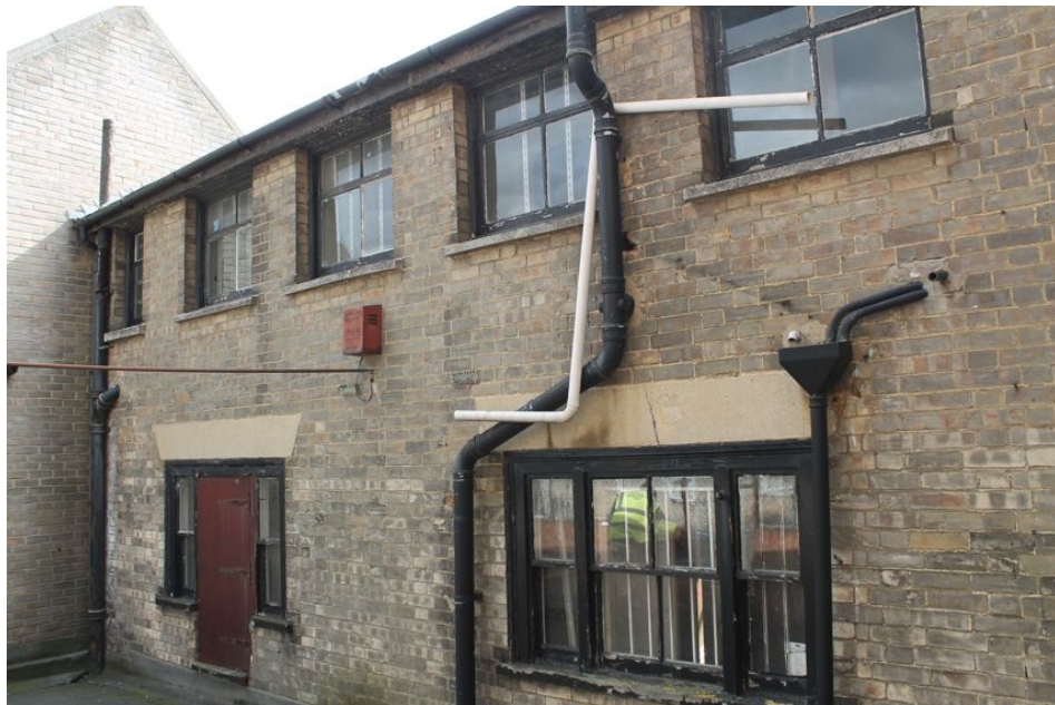
Photograph 72 Northern elevation of Building D. Photograph taken from roof of Building E, facing south-east.
