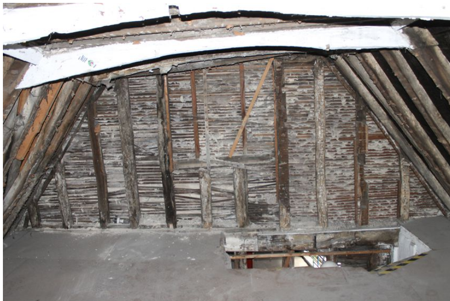
Photograph 64 East gable end in Building B, showing inserted window opening that has been covered in lath and plaster. Photograph taken facing east.
