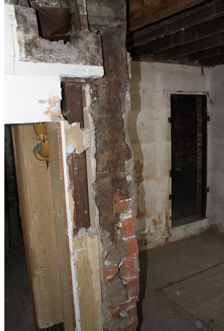
Photograph 8 Remains of south-east corner-post of Building A at the ground floor. Photograph taken facing north-east.
