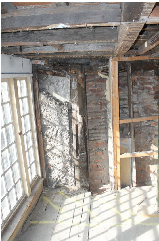
Photograph 18 North-west corner-post of Building A, showing unused mortice for arch brace and scarf joint above. Photograph taken facing north.
