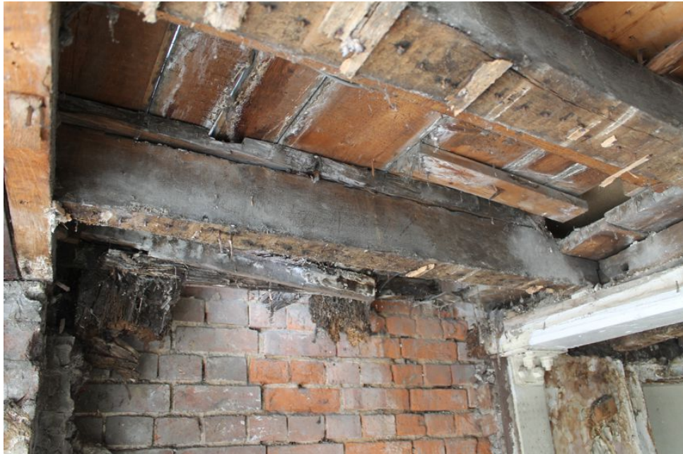
Photograph 11 Remains of current corner-post (left) and possible original corner-post projecting from first-floor (centre) on ground-floor on the northern elevation of Building A. Photograph taken facing north.
