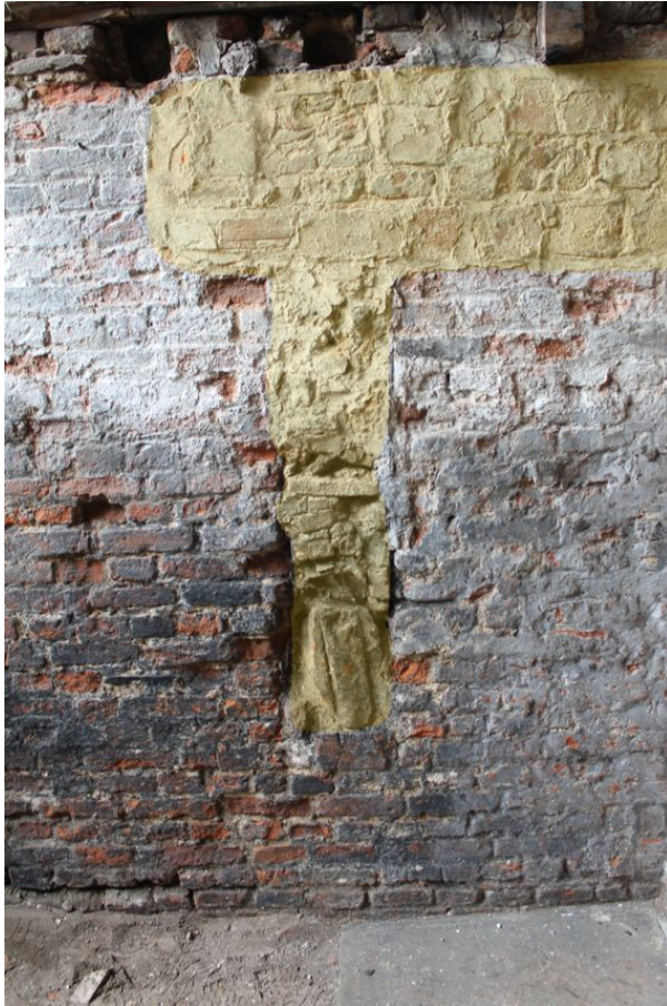
Photograph 47 Northern elevation of cellar, with repaired section of wall highlighted. Photograph taken facing north.
