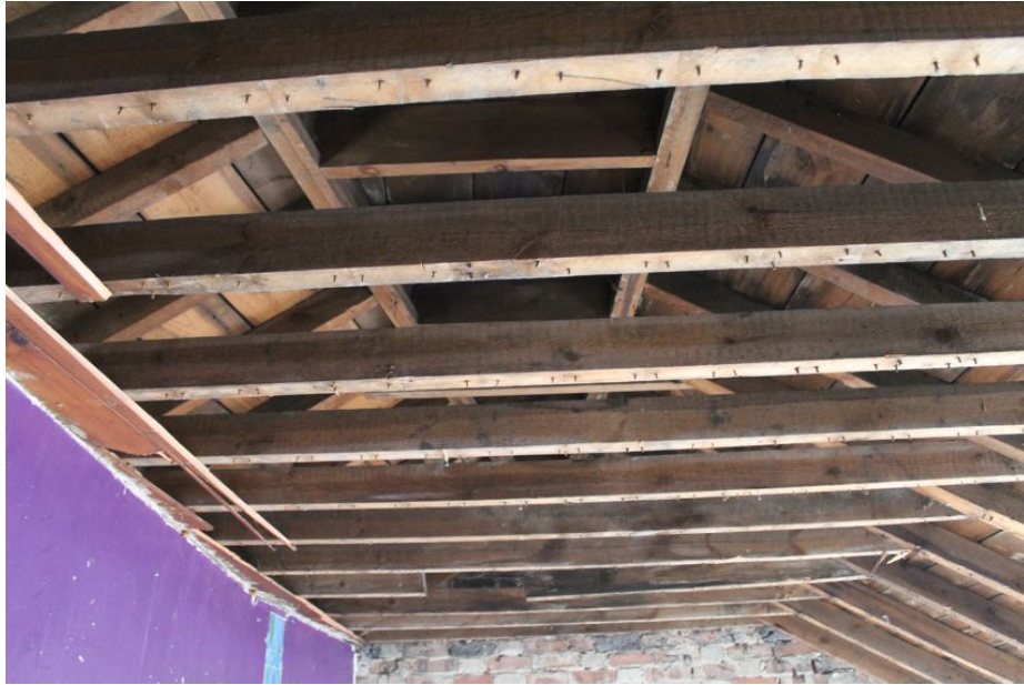
Photograph 77 Detail of roof in Building D, showing the tapering of the gambrel roof to a gable. Photograph taken facing east.
