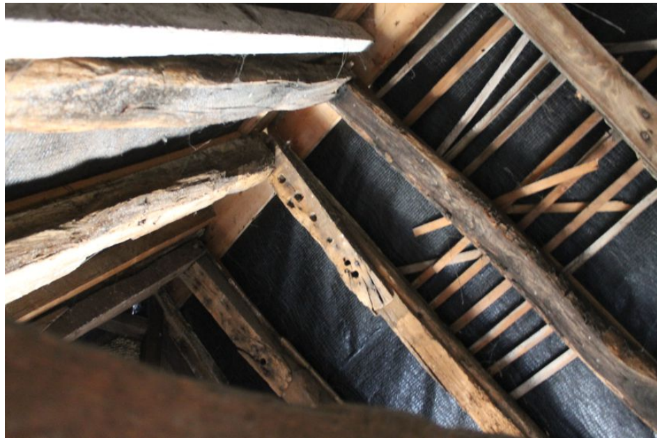
Photograph 61 Roof of Building B with scarf joints on rafters. Photograph taken facing south-east.
