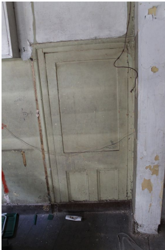
Photograph 73 Blocked door in western wall of ground-floor of Building D. Photograph taken facing west.
