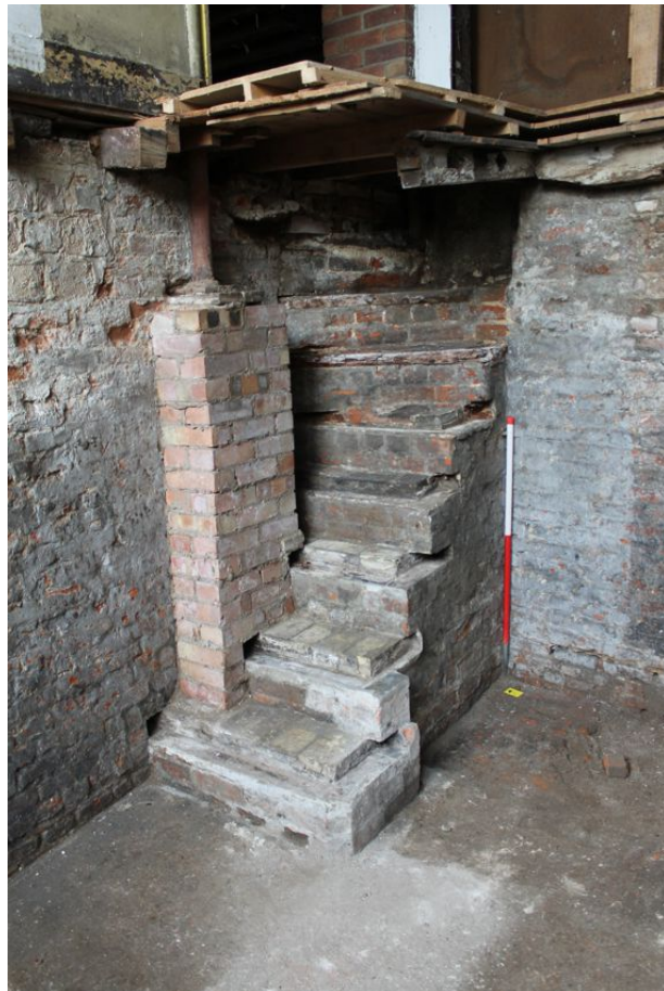
Photograph 43 Brick stairway into cellar. Also visible is brick pillar added to support metal post. Photograph taken facing north-east.
