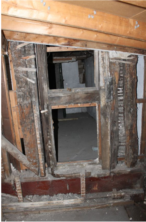
Photograph 55 Detail of inserted window-frame in east wall of Building B's first-floor. Photograph taken facing west.
