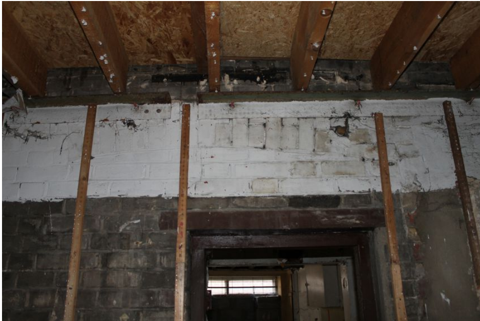
Photograph 71 Archway above inserted doorway in northern elevation of Building D, showing location of original window. Photograph taken facing south.
