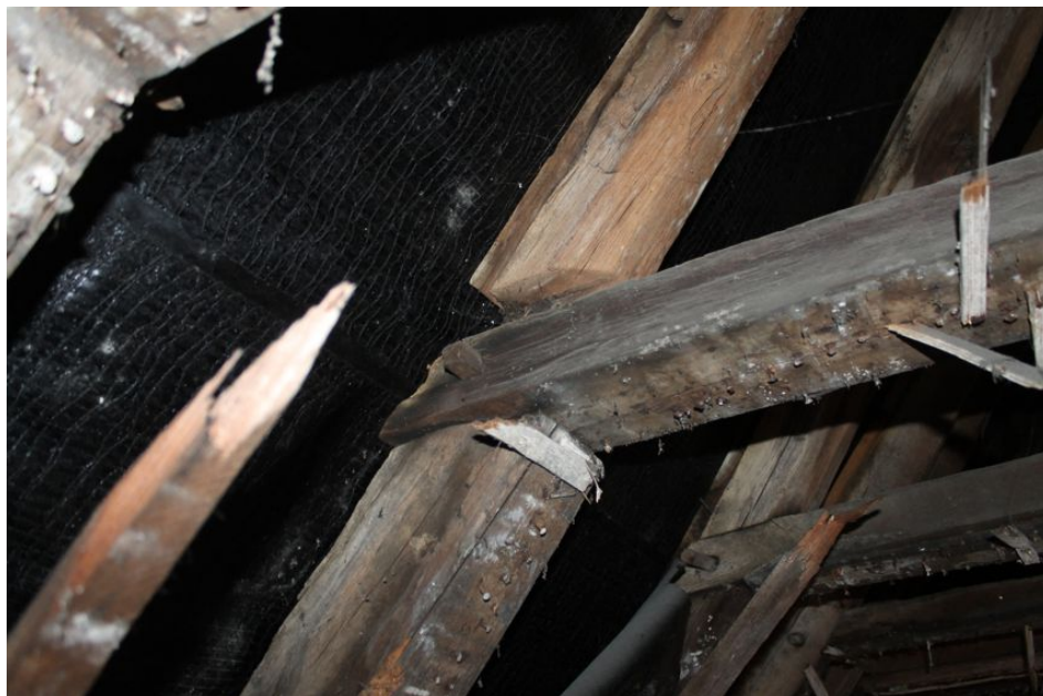
Photograph 25 Detail of peg joining collar and rafter in east room of Building A. Photograph taken facing north-east.
