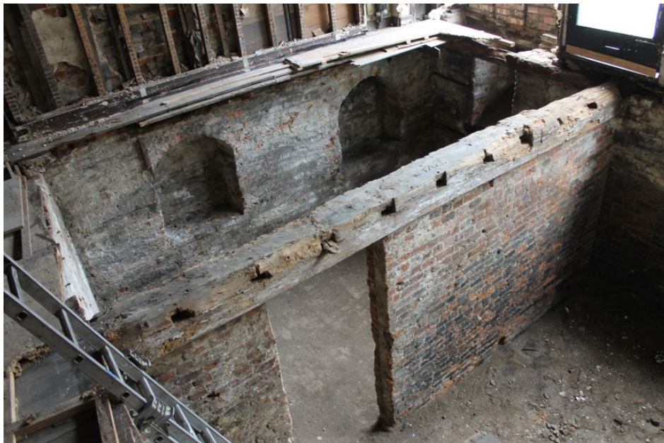
Photograph 41 Cellar beneath Building B, showing recesses for shelving. Photograph taken facing south-east.
