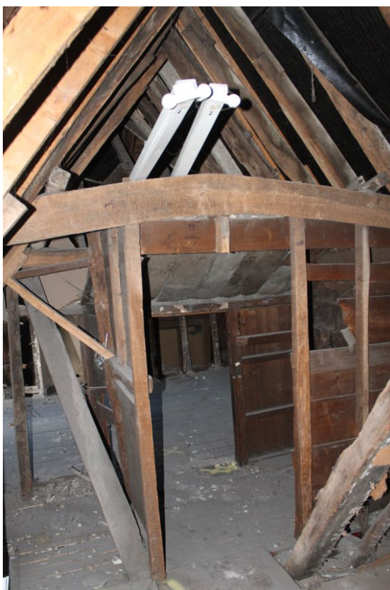
Photograph 32 Small timber room in the joining section of roof between the second-floor of Buildings A and B. Arched collar used as part of the structure. Photograph taken facing north.
