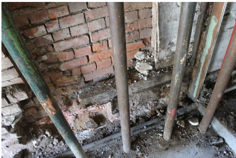
Photograph 9 Remains of sill-beam and brick plinth on northern elevation of Building A. Photograph taken facing north.
