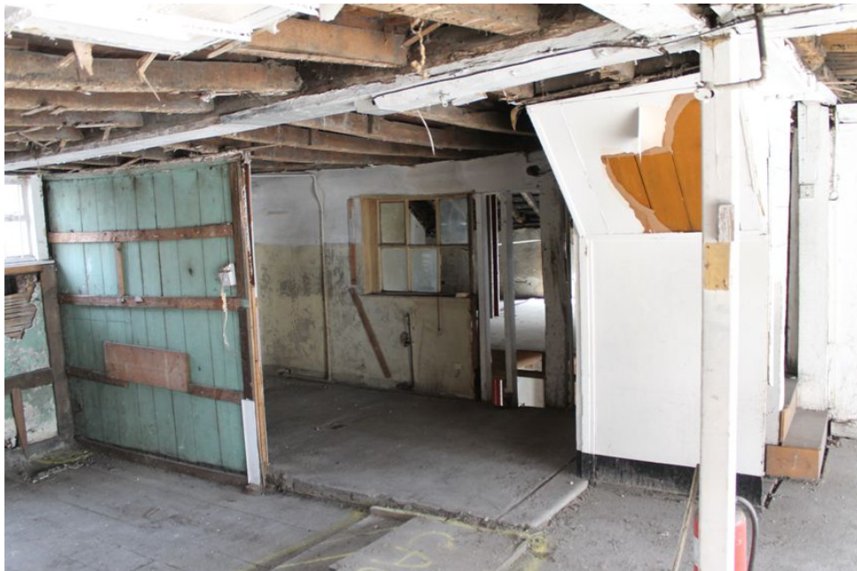
Photograph 21 First-floor of Building A, with binding-beams visible supporting floor above and modern post in centre of building. Photograph taken facing south-east.
