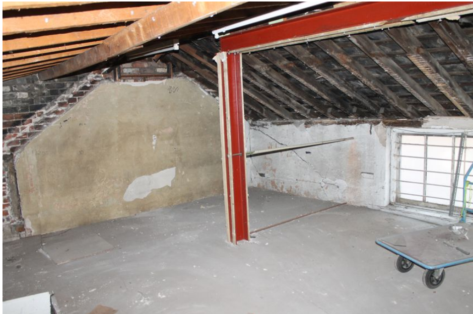
Photograph 69 First-floor of Building C, with original outline of roof against Building D visible. Photograph taken facing south-east.
