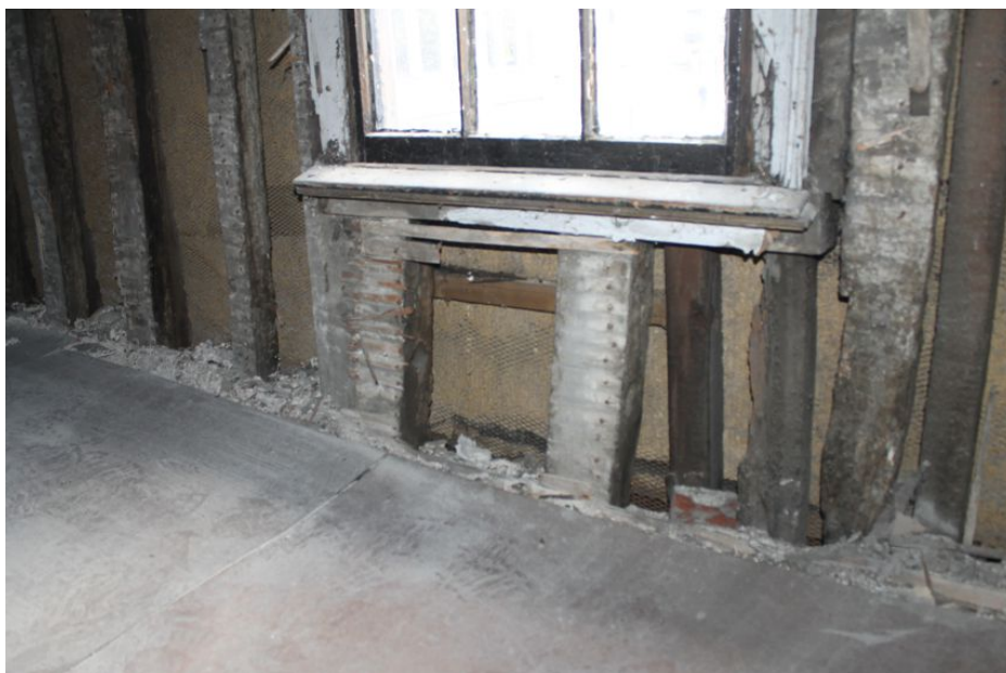
Photograph 65 Cut studs beneath inserted window in west gable end of Building B. Diamond mullions visible on left stud. Photograph taken facing south-west.
