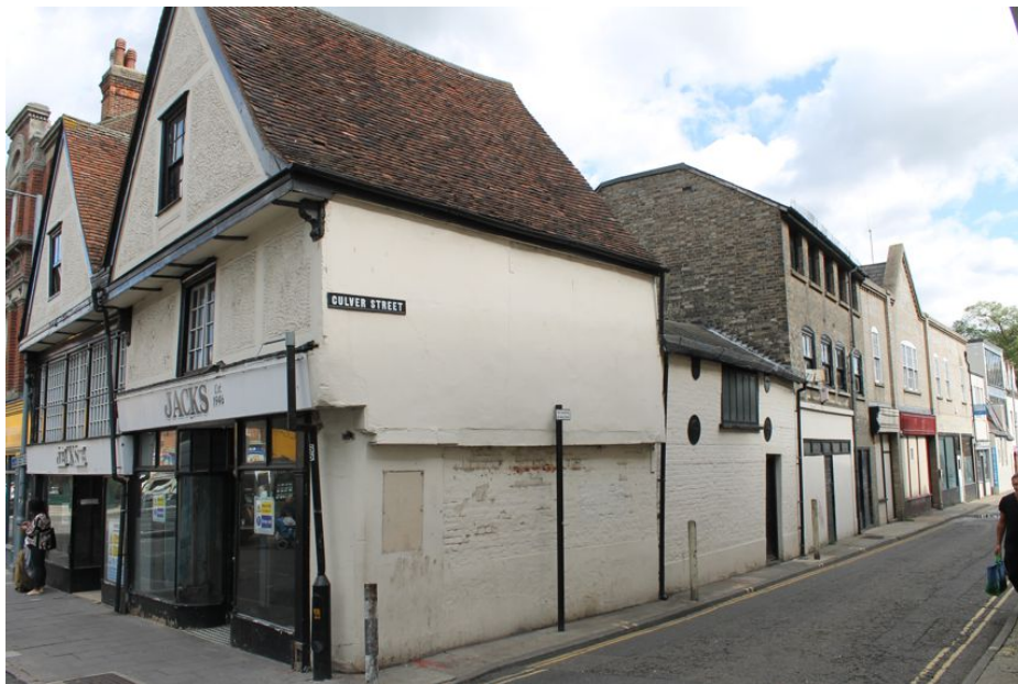
Photograph 40 Southern elevation of Building B, showing brick underbuilding. Photograph taken facing north-east.
