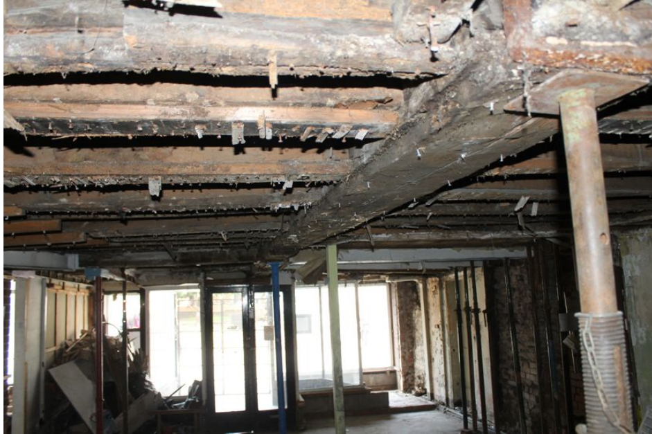
Photograph 14 Underside of first-floor in Building A. Chamfered binding-beam and supporting iron strap visible. Photograph taken facing west.
