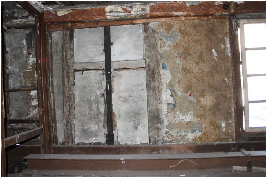
Photograph 58 Western wall of first-floor in Building B, showing possible infilled window opening. Photograph taken facing west.
