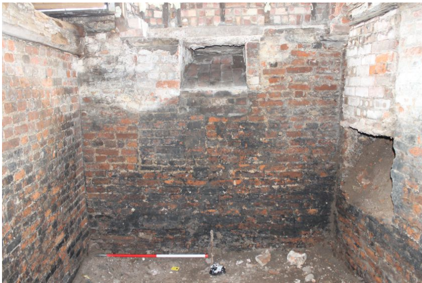
Photograph 46 Western elevation of northern room, showing coal chute replacing an earlier, bricked up, opening. Photograph taken facing west.
