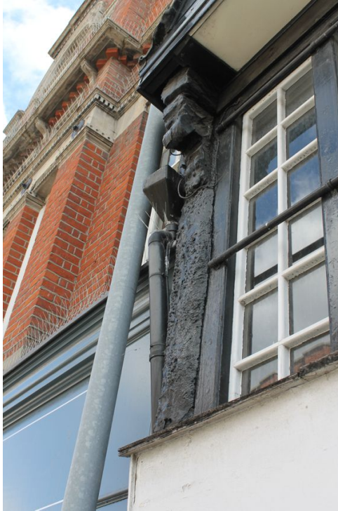
Photograph 5 North-west corner-post supporting second-floor jetty. Note carved top. Photograph taken facing north-east.
