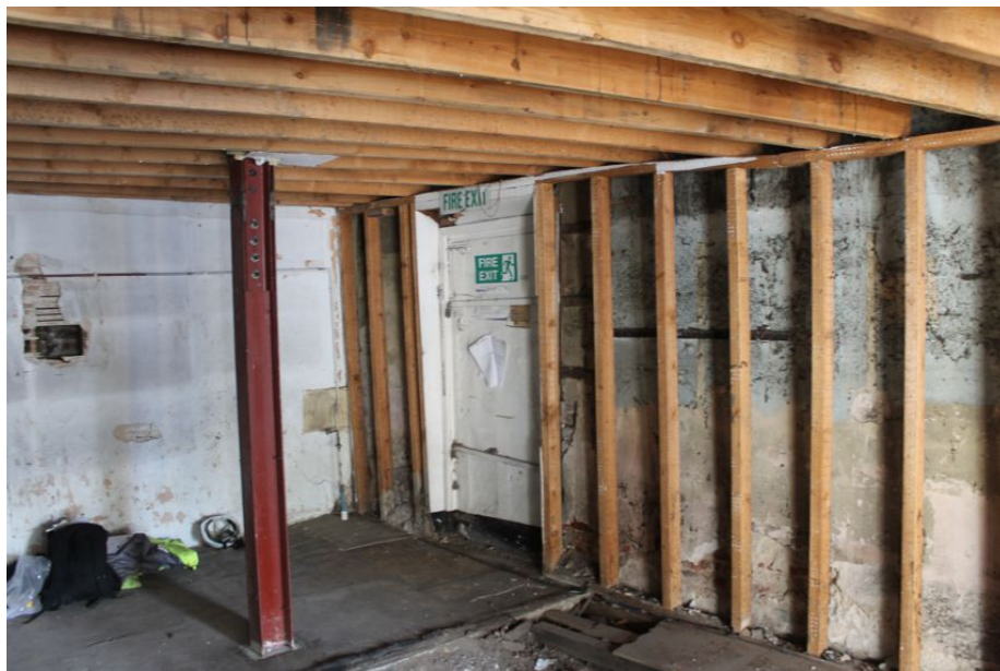
Photograph 68 Ground-floor of Building C, showing modern timber-frame in inside brickwork exterior. Photograph taken facing south-east.
