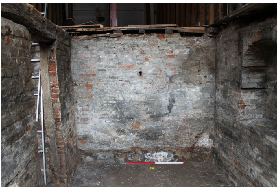
Photograph 51 Eastern wall in southern room of cellar, with Roman foundation at base. Photograph taken facing east.
