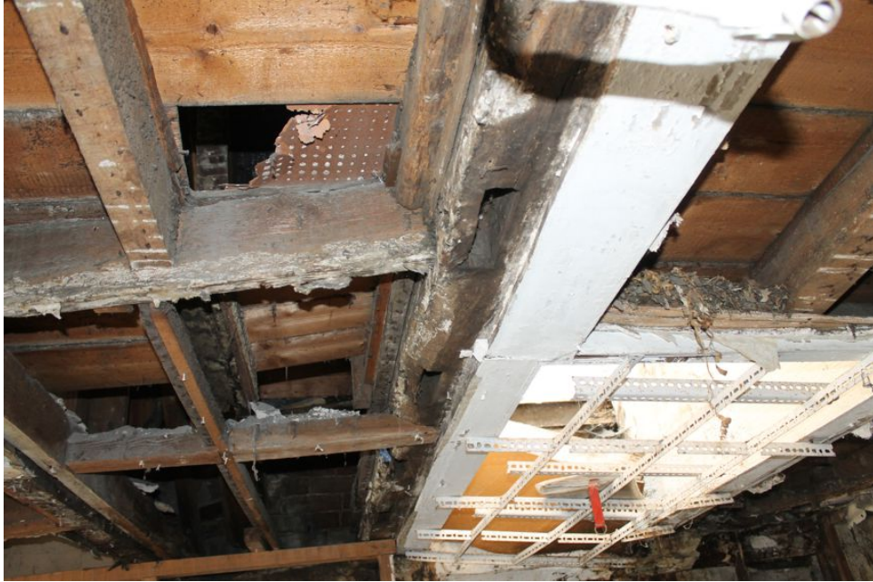
Photograph 22 Underside of north-south binding-beam supporting the second-floor, showing unused mortices. Photograph taken facing north.
