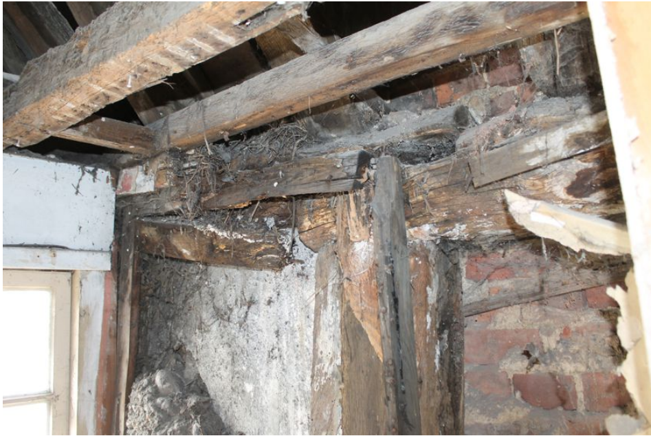
Photograph 19 Detailed photograph showing scarf joint in wall-plate above north-west corner-post in Building A. Photograph taken facing north-west.
