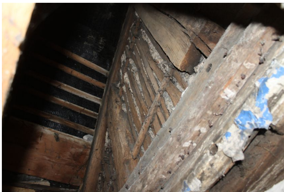
Photograph 33 Possible original rudimentary lath and plaster on west side of the modern skylight in Building A. Photograph taken from first-floor looking up.
