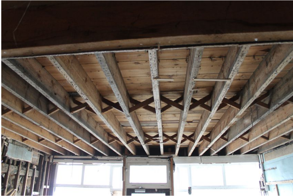
Photograph 53 Underside of raised first-floor in Building B, showing herringbone strutting supporting joists. Photograph taken facing west.
