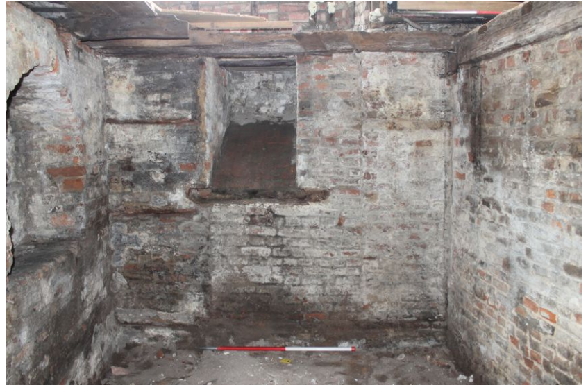
Photograph 45 Western elevation of southern room, showing coal chute inserted into an earlier, bricked up, opening. Photograph taken facing west.
