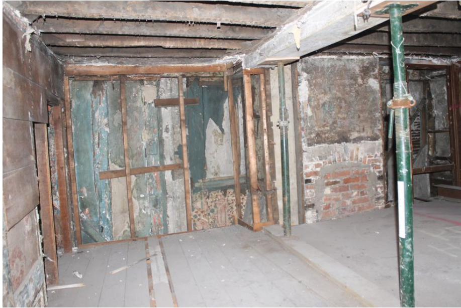
Photograph 57 Internal southern elevation of first-floor in Building B. Photograph taken facing south.
