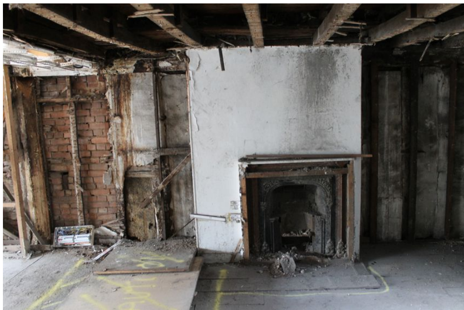
Photograph 16 Chimney-stack and later fireplace in first-floor of Building A. Photograph taken facing north.
