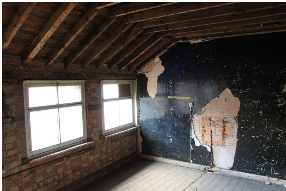
Photograph 76 Second-floor of Building D. Hollow-tile bricks visible beneath plaster to right. Photograph taken facing south-west.
