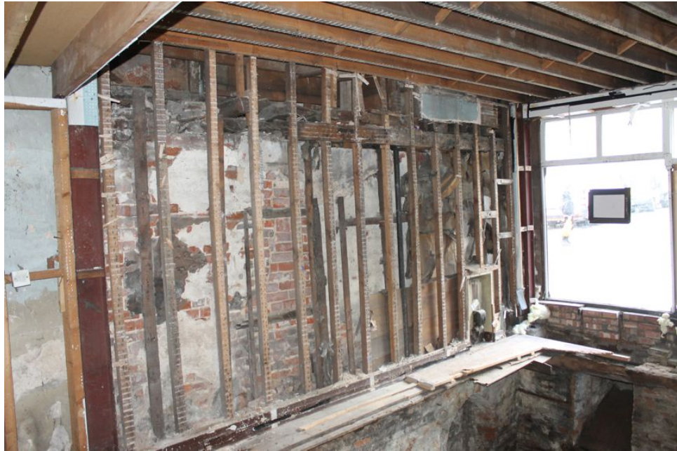
Photograph 52 Southern elevation of ground-floor of Building B, showing timber-frame partially surviving but obscured by later brickwork. Partially surviving girding-beam visible. Photograph taken facing south-west.
