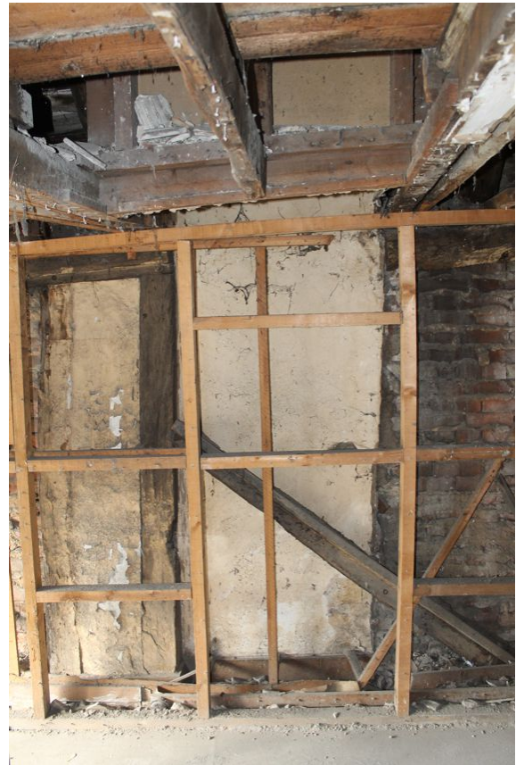
Photograph 17 Wall-plate cut and lath and plaster added behind on first-floor of Building A. Photograph taken facing north.
