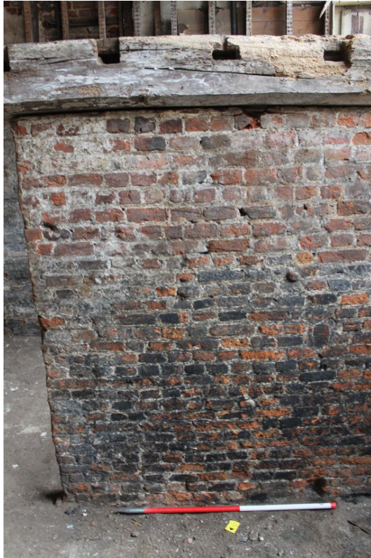
Photograph 49 Detail of dividing wall in cellar, showing two phases of brickwork. Photograph taken facing south.
