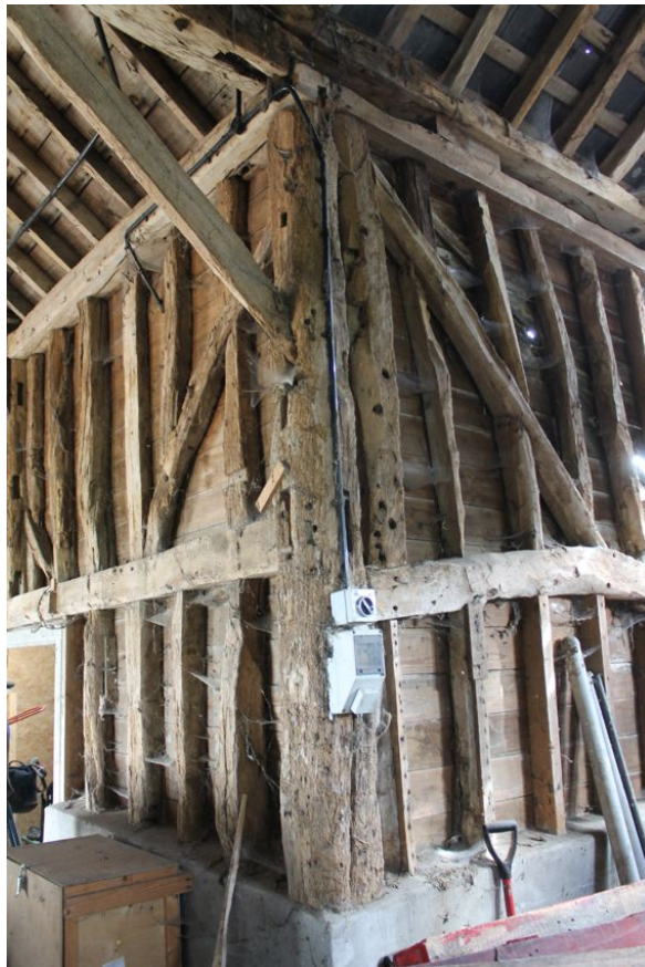
Photograph 18 Principal-post on southern elevation between bays 3 and 4. Open mortice for possible gird-beam visible on west (right) face. Cut wall-plate visible at top of post. Photograph taken facing south-east.
