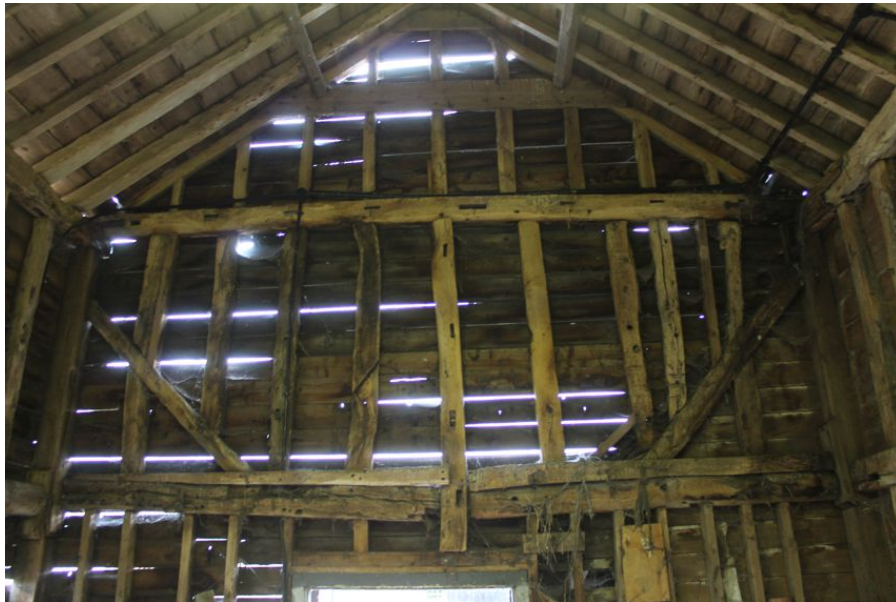
Photograph 9 Detail of eastern gable-end of barn, showing multiple re-used timbers. Photograph taken facing east.
