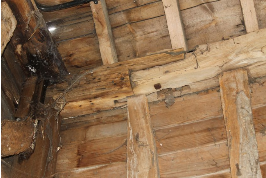
Photograph 14 Edge-halved scarf joint with bridled abutments in southern wall-plate of bay 5, adjacent to south-east corner-post. Photograph taken facing south.
