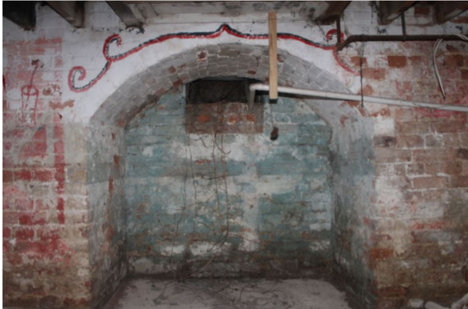
Photograph 30 Alcove in western wall of cellar. Bricked up skylight? visible. Photograph taken facing west.
