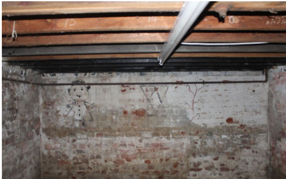
Photograph 31 Graffiti on southern wall of cellar. Photograph taken facing south.
