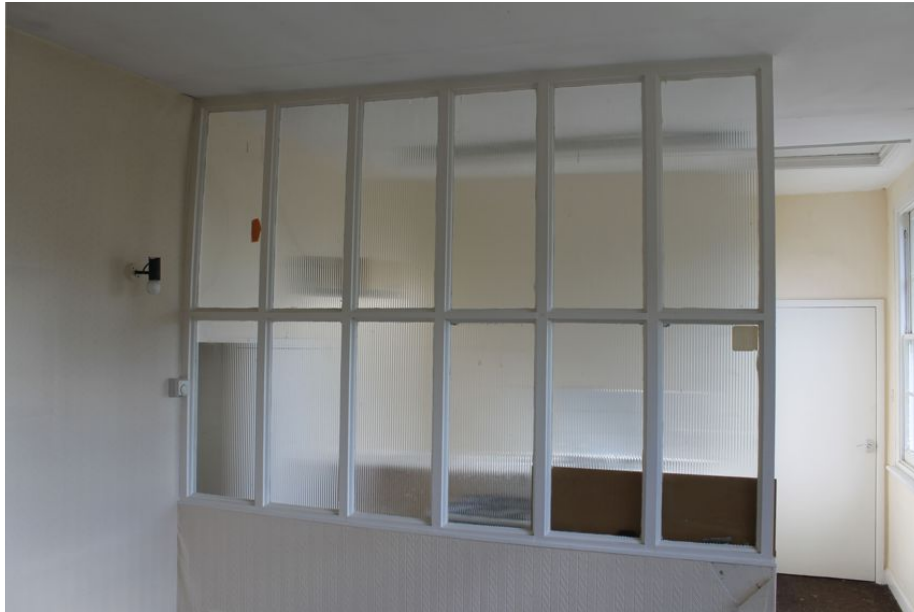
Photograph 36 Glass division in first-floor of farmhouse, added in 1976. Photograph taken facing north-west.
