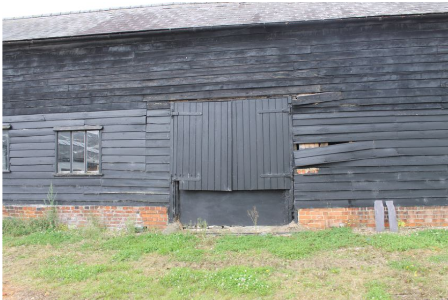
Photograph 3 Detail of double-door on northern elevation of barn, with evidence of rebuilt plinth visible. Photograph taken facing south.
