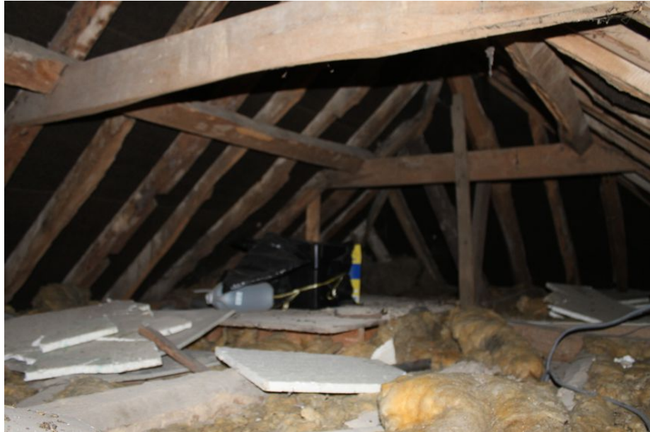
Photograph 38 Roof of farmhouse, with multiple re-used timbers and modern supports. Photograph taken facing north-west.
