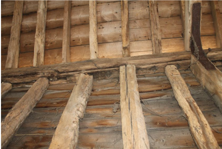
Photograph 10 Detail of underside of northern wall-plate in bay 4, showing diamond mullions. Photograph taken facing north.
