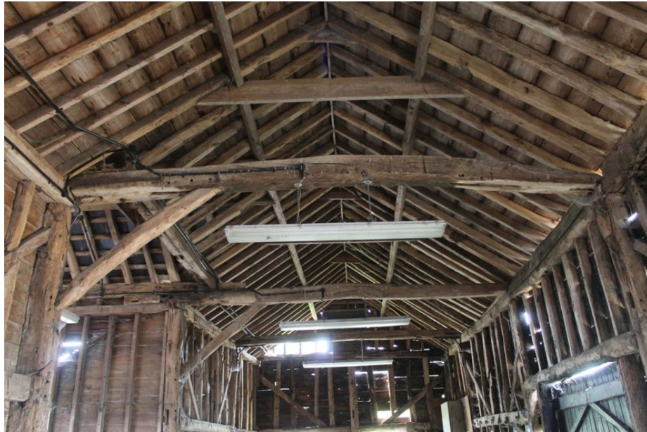
Photograph 15 Interior of barn, showing roof trusses. Tie-beam between bays 3 and 4 in foreground. Photograph taken facing west.
