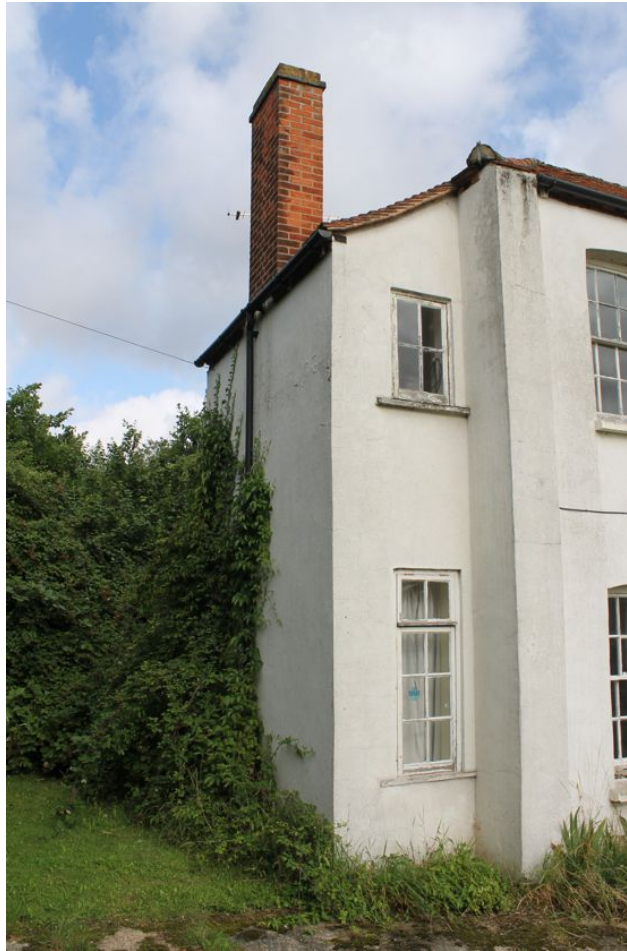
Photograph 26 Southern and eastern elevation of farmhouse, showing extension D. Photograph taken facing north-west.
