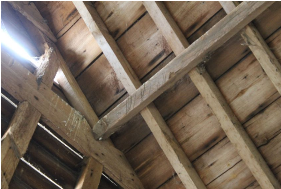
Photograph 23 Purlin on southern pitch of roof, adjacent to eastern gable-end. Baltic shipping marks visible. Photograph taken facing south-east.
