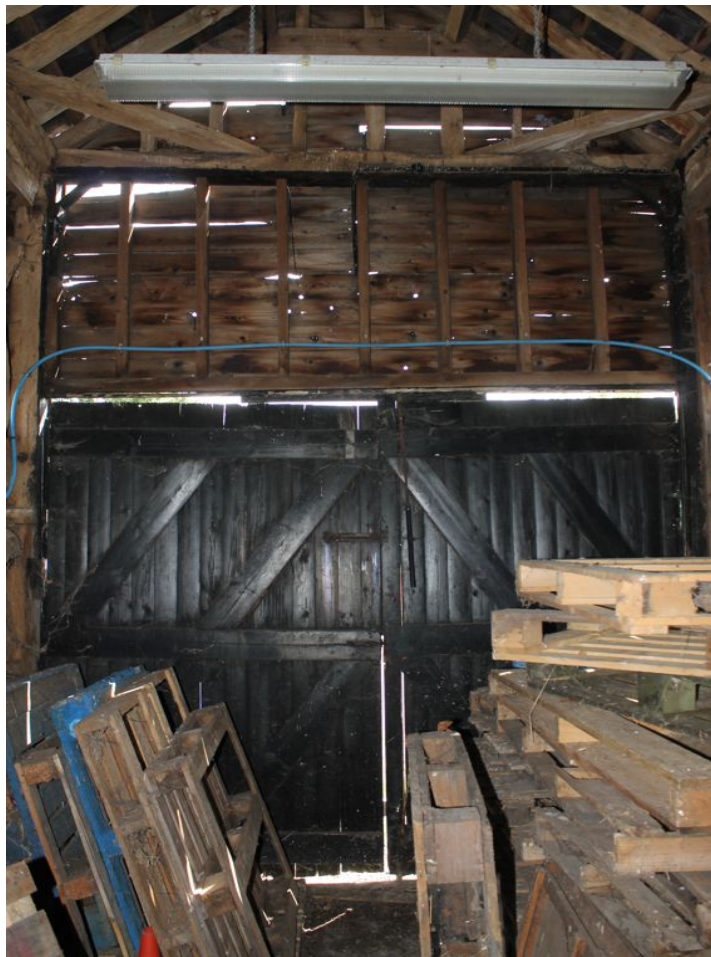
Photograph 22 Southern elevation of midstrey, with inserted modern timbers above double-doors. Original door would have been full height. Photograph taken facing south.
