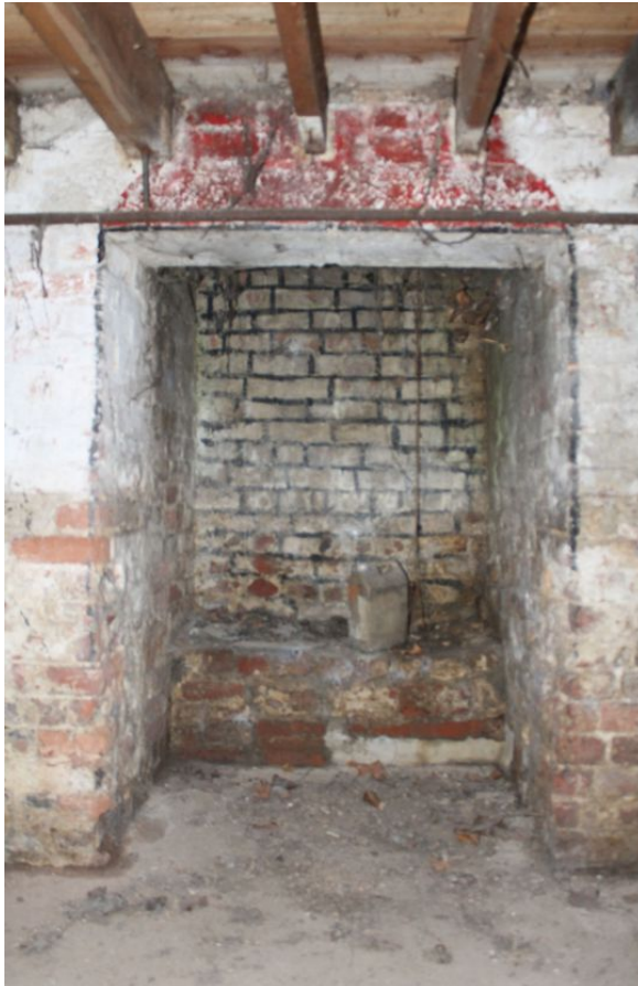
Photograph 29 Bricked up entrance? to cellar below skylight. Photograph taken facing east.
