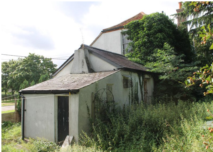
Photograph 27 Western and northern elevation of farmhouse, showing extensions A and B. Photograph taken facing south-east.
