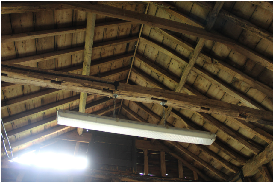
Photograph 16 Underside of roof truss between bays 1 and 2, showing unused mortices. Photograph taken facing west.
