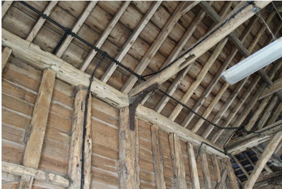
Photograph 17 Metal knee-brace supporting southern end of tie-beam between bays 4 and 5. Photograph taken facing south-west.
