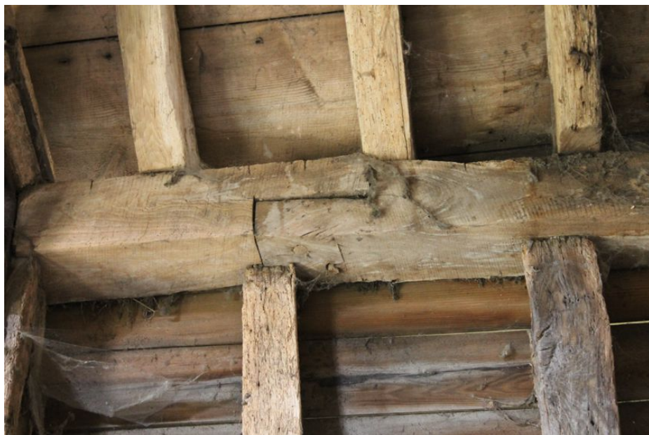
Photograph 13 Rudimentary scarf joint in northern wall-plate of bay 2. Photograph taken facing north.
