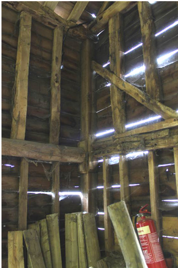
Photograph 11 Detail of north-east corner-post, showing extra timber supporting girding-beams. Photograph taken facing north-east.
