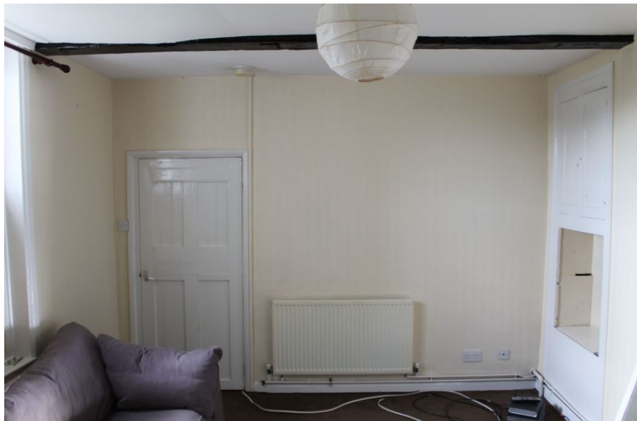
Photograph 33 Original southern wall of central room on ground-floor of farmhouse. Original door to left. Photograph taken facing south.
