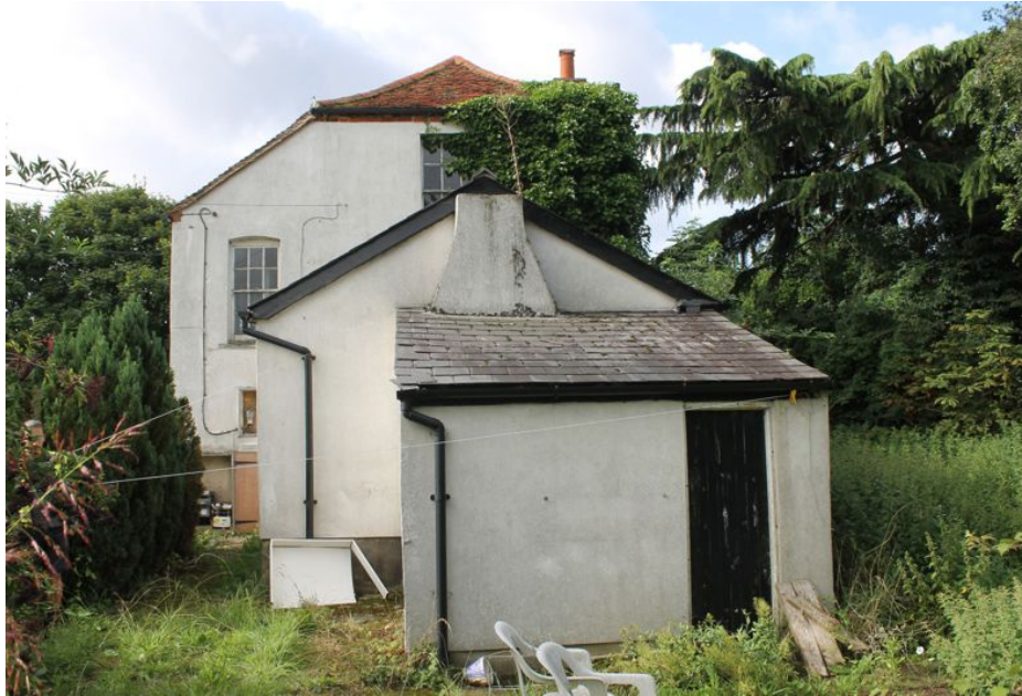
Photograph 25 Northern elevation of farmhouse, showing extensions B and C. Photograph taken facing south.
