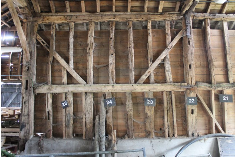
Photograph 12 Southern elevation of bay 2, showing multiple re-used timbers and rafters supported on intermediate timber, rather than wall-plate. Photograph taken facing south.
