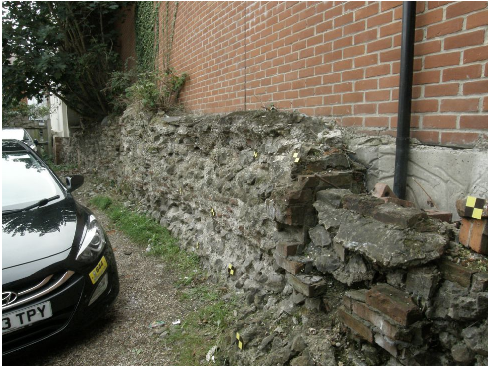
Photograph 6 Section 21 of the wall after removal of vegetation. Photograph taken facing south-east.
