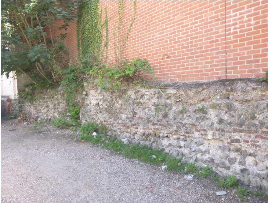
Photograph 5 Section 21 of the wall before removal of vegetation. Photograph taken facing south-east.
