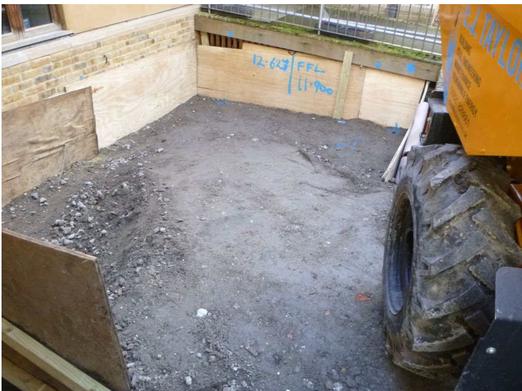
Photograph 2 Excavation area backfilled with Type 1 ballast ready for the piling rig – view south-east
