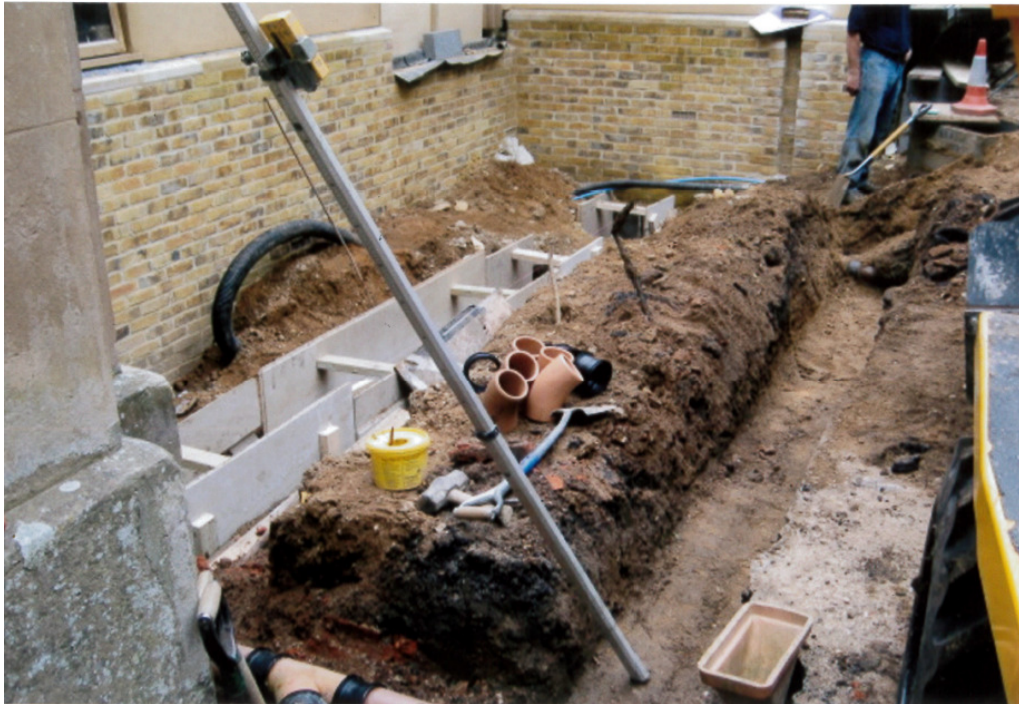
Photograph 4 The walled flower bed under construction after the demolition of the vestry and the construction of the 2009 extension – view south-east (photograph courtesy of St Leonard's Church PCC)
