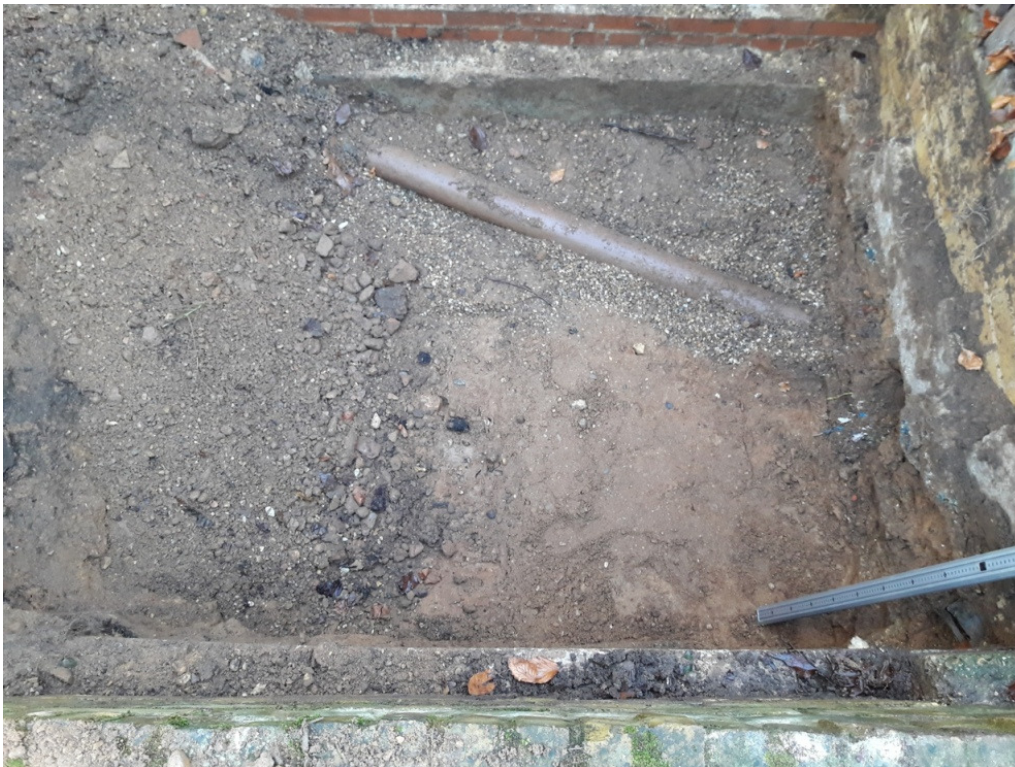
Photograph 1 Formation level in southern half of excavation area with services and retaining wall – view east
