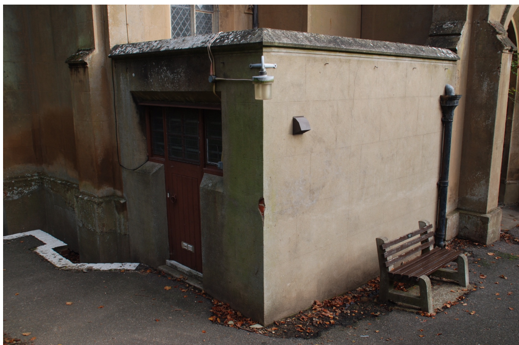
Photograph 3 The choir vestry prior to demolition – view north-east (photograph courtesy of St Leonard's Church PCC)
