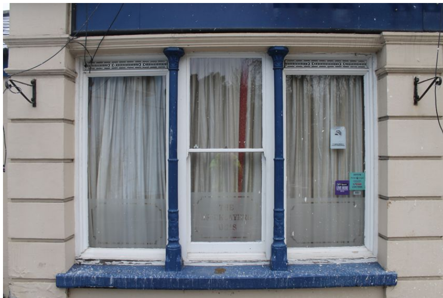
Photograph 9 Detail of fixed and sash-windows on south-east elevation. Photograph taken facing north-west.
