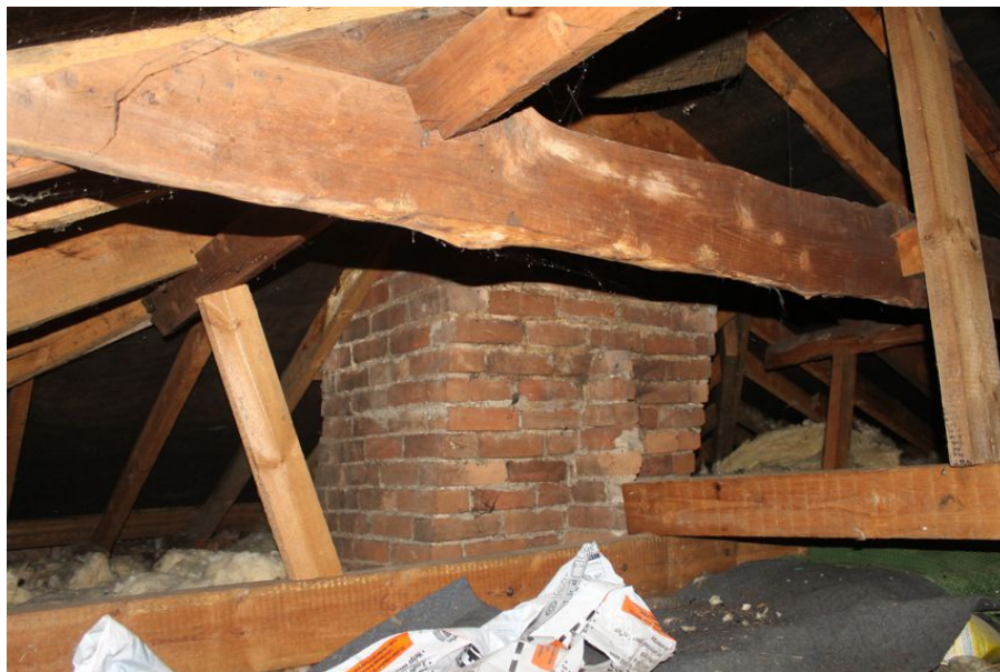
Photograph 26 Northern chimney-stack in roof. Also visible is rudimentary hand-sawn collar and clasped purlins. Photograph taken facing east.
