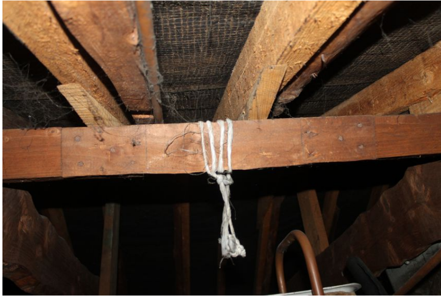
Photograph 25 Detail of purlin on north-west pitch of roof with two adjacent nailed scarf joints. Also at top of the frame visible are rafters with modern supporting timbers. Photograph taken facing south-east.
