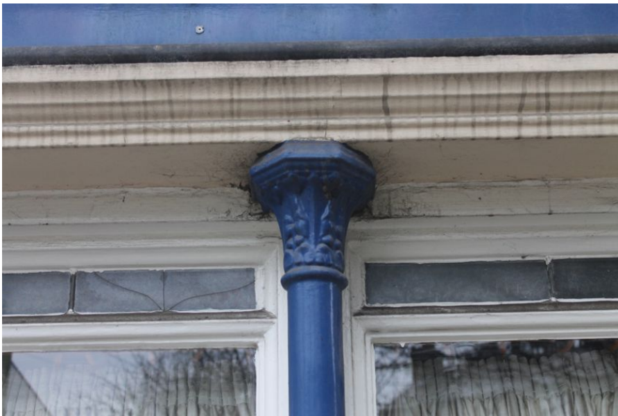
Photograph 11 Detail of decoration on apex of metal post between windows on the north-east elevation of pub. Photograph taken facing south-west.
