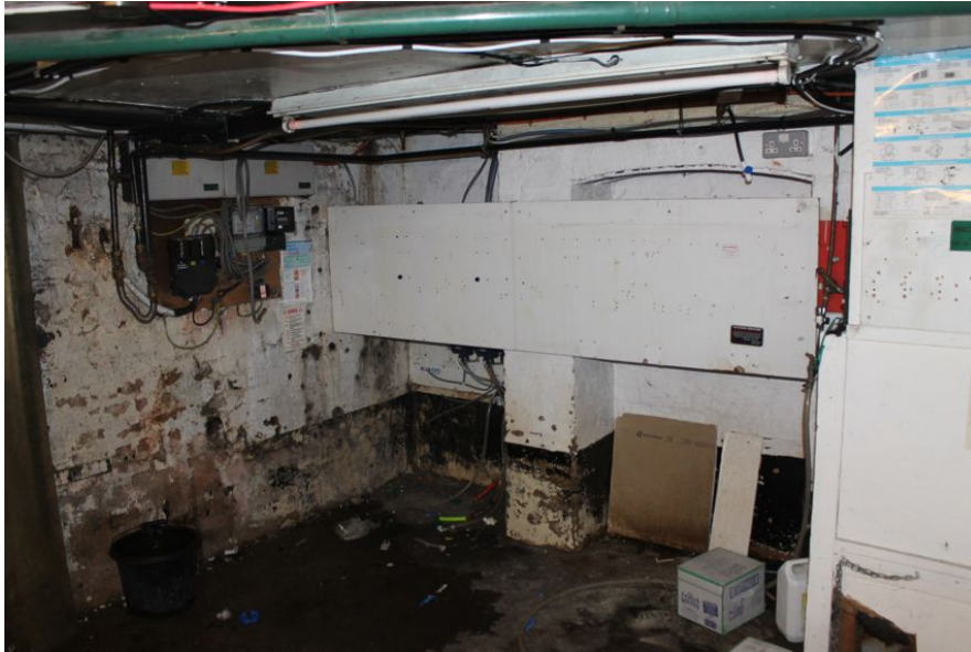
Photograph 14 Interior of cellar, showing brick arch supporting chimney-stack on upper floors. Photograph taken facing east.
