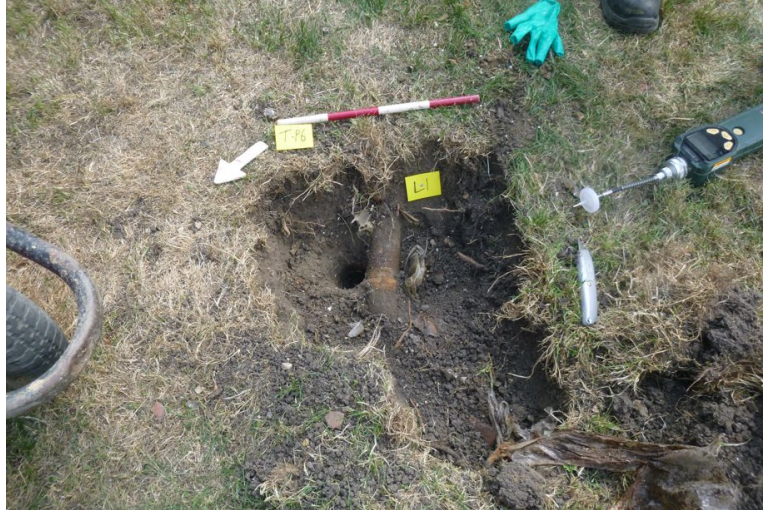
Photograph 7 TP6 after excavation, shows oil pipe turning west. Photograph taken facing south-east.
