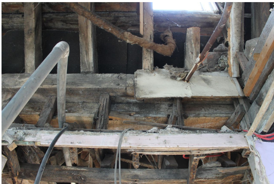
Photograph 60 Detail of scarf joint on north-west wall plate of Structure C. Photograph taken facing north-west.
