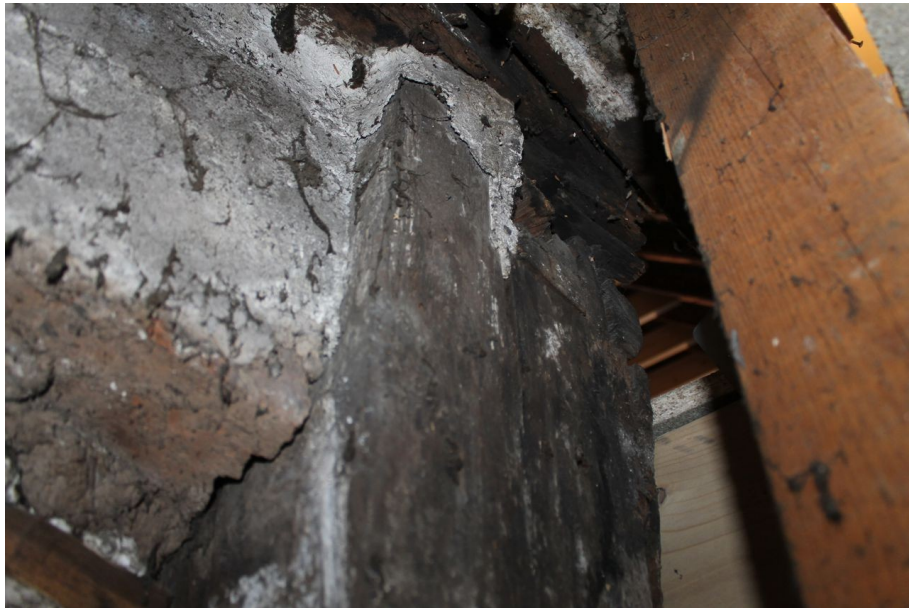
Photograph 48 Detail of mortice on northern corner-post of Structure A, possibly for supporting girding-beam of northern wing. Photograph taken facing west.
