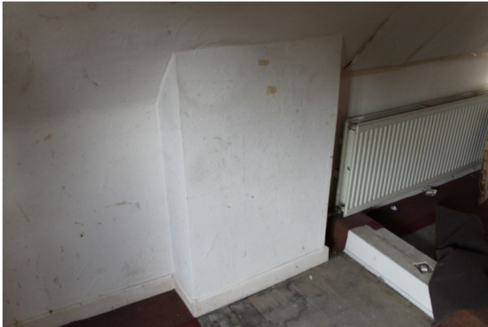
Photograph 33 Blocked fireplace and exposed tie-beam on second-floor of Structure C. Photograph taken facing north.
