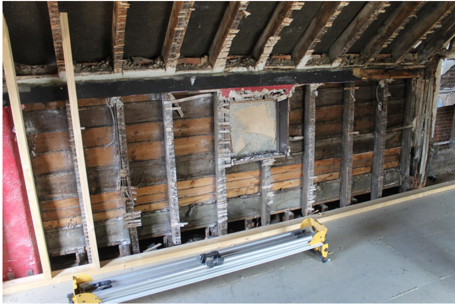
Photograph 51 Exposed machine-cut timber-frame of Structure B on north-east elevation, including inserted window. Photograph taken facing east.
