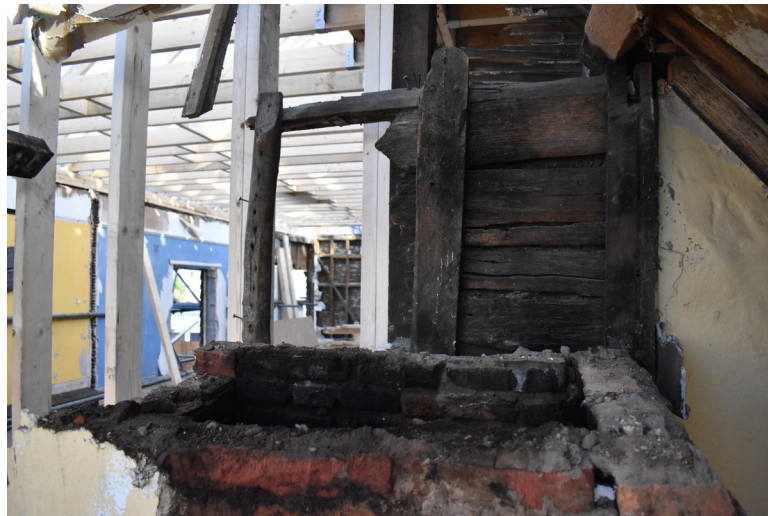
Photograph 64 Detail of possibly original weatherboarding behind chimney-stack on northern elevation of Structure A. Photograph taken facing north-east.
