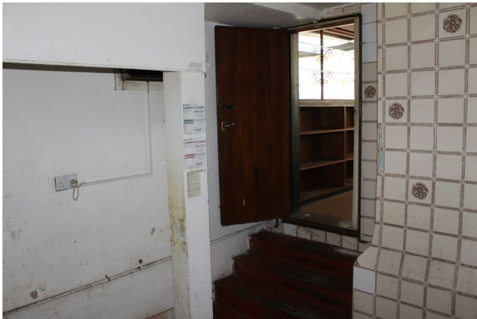
Photograph 35 Photo showing floor-level difference between Structure D and Structure C. Photograph taken facing east.
