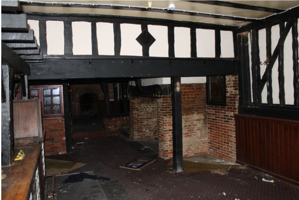
Photograph 13 South-east elevation of Structure A from interior of Structure F. Inserted beam and post visible. Photograph taken facing north-west.
