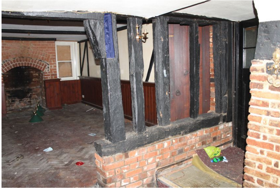
Photograph 17 Section of surviving original stud-work in north-west wall of Structure A. Modern inserted timber blocking doorway second from right. Mortice for brace supporting original first-floor highlighted in blue. Photograph taken facing north.
