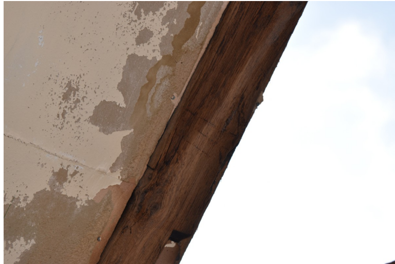
Photograph 63 Detail of carpenter's mark "III" on eastern rafter of Structure A. Photograph taken facing south.
