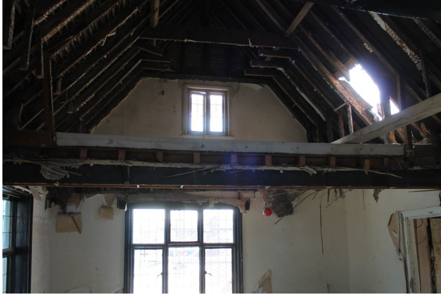
Photograph 56 Southern-most tie-beam in Structure C, showing secondary modern timber attached to its upper face for reinforcement. Photograph taken facing south-west.
