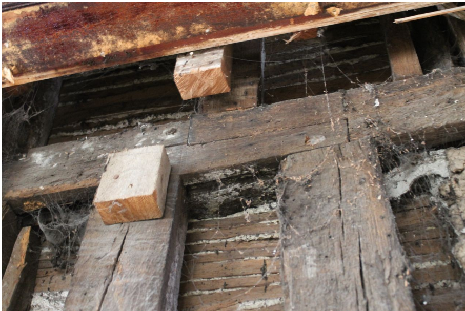
Photograph 46 Detail of scarf joint on south-east girding-beam of Structure A. Photograph taken facing north-west.
