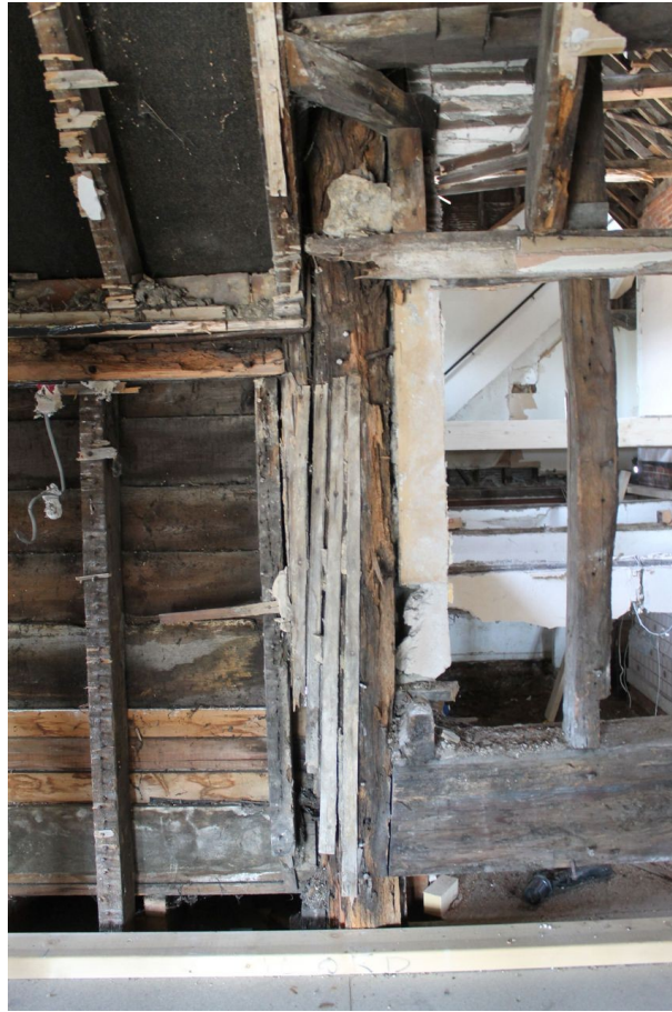
Photograph 58 Detail of west reused corner-post of Structure D, photo taken from within Structure B. Photograph taken facing north-east.
