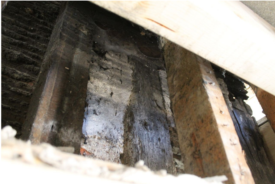
Photograph 50 Timber and plaster behind chimney stack in Structure A. Photograph taken facing west.
