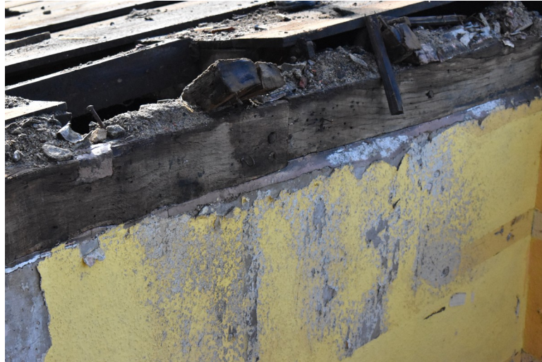
Photograph 61 Detail of edge-halved scarf-joint on eastern wall-plate of Structure A. Photograph taken facing south.
