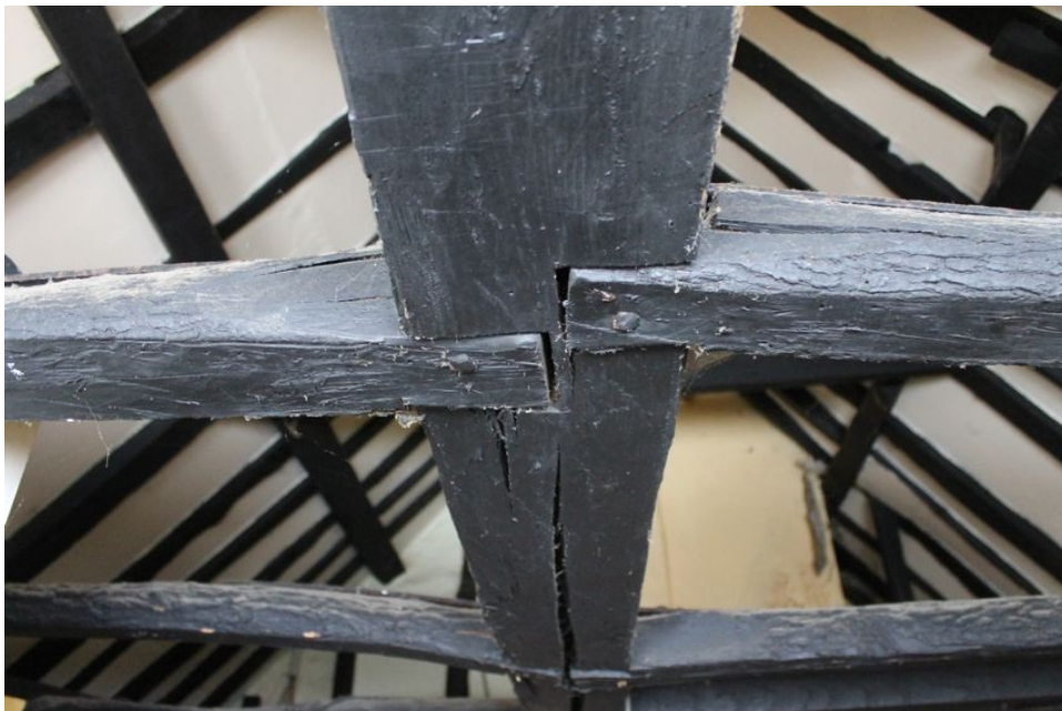
Photograph 21 Detail of underside of collar-purlin, showing joggled lap-joints. Photograph taken facing north-east.
