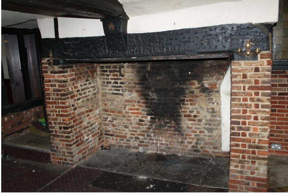
Photograph 14 Large fireplace in north-east ground-floor wall of Structure A. Photograph taken facing north.
