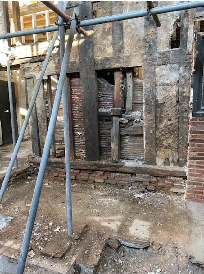
Photograph 65 Northern elevation of Structure A after complete removal of chimney, with plaster and timber infilling visible. Photograph taken facing north.
