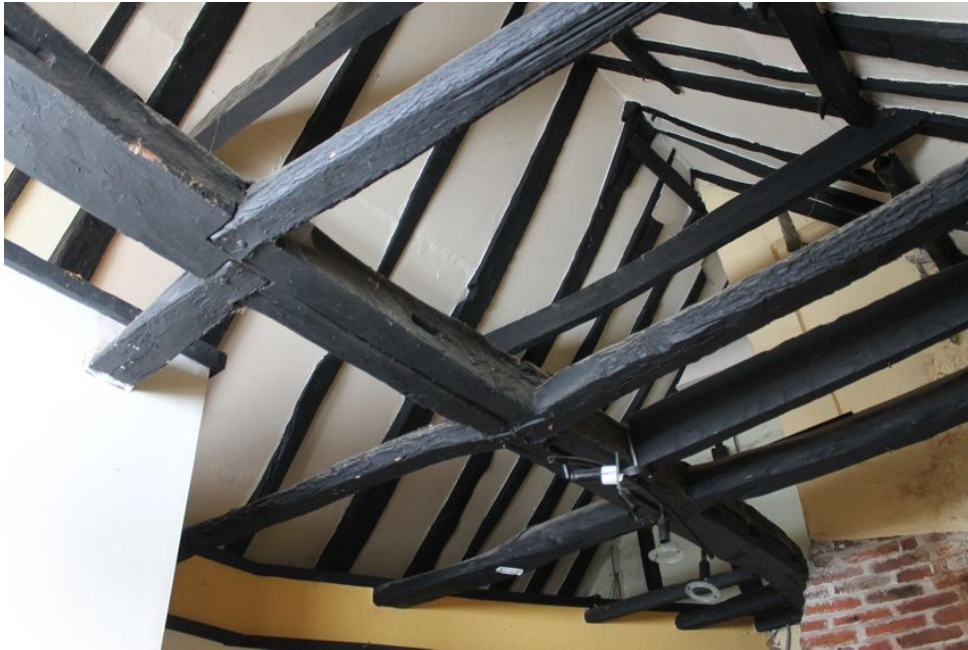
Photograph 20 Roof structure of Structure A, showing collar-purlin and braces. Photograph taken facing north.
