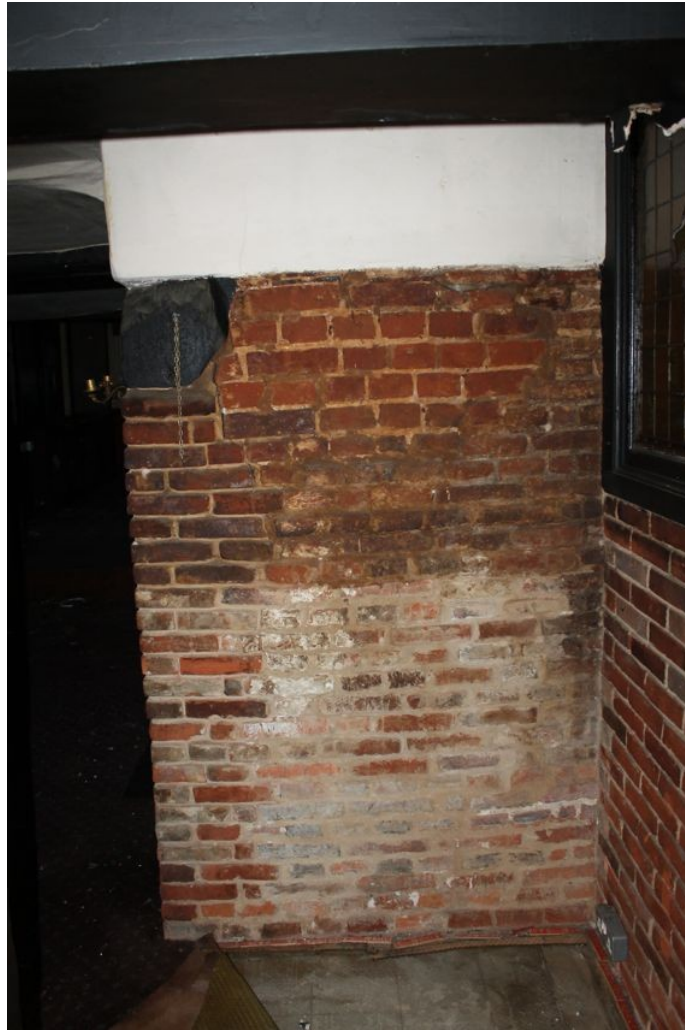
Photograph 15 South-east side of fireplace, showing rebuilt areas compared to original brickwork. Photograph taken facing north-west.
