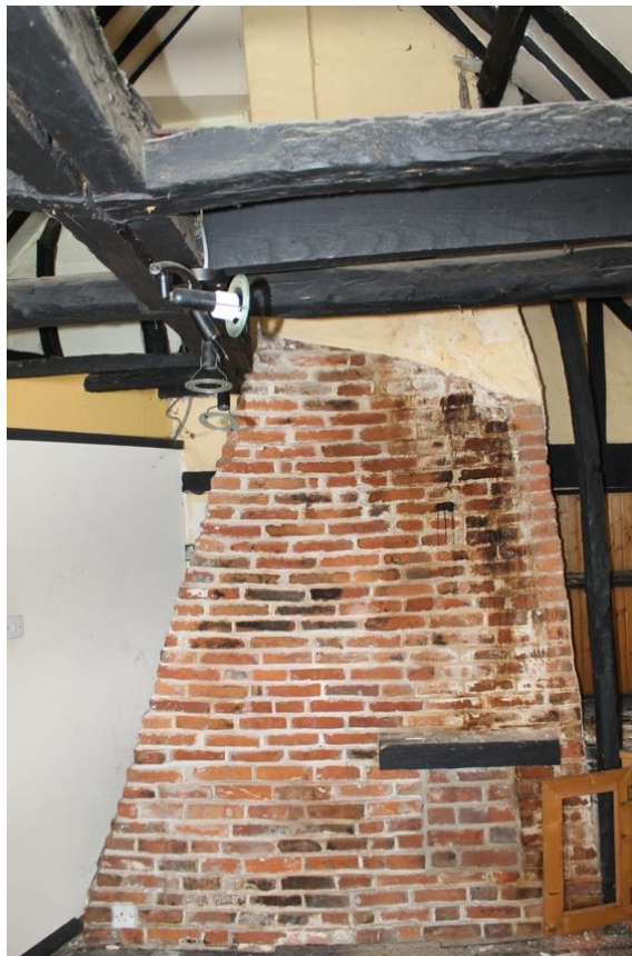
Photograph 19 Chimney stack in north-east first-floor wall of Structure A. Photograph taken facing north-east.
