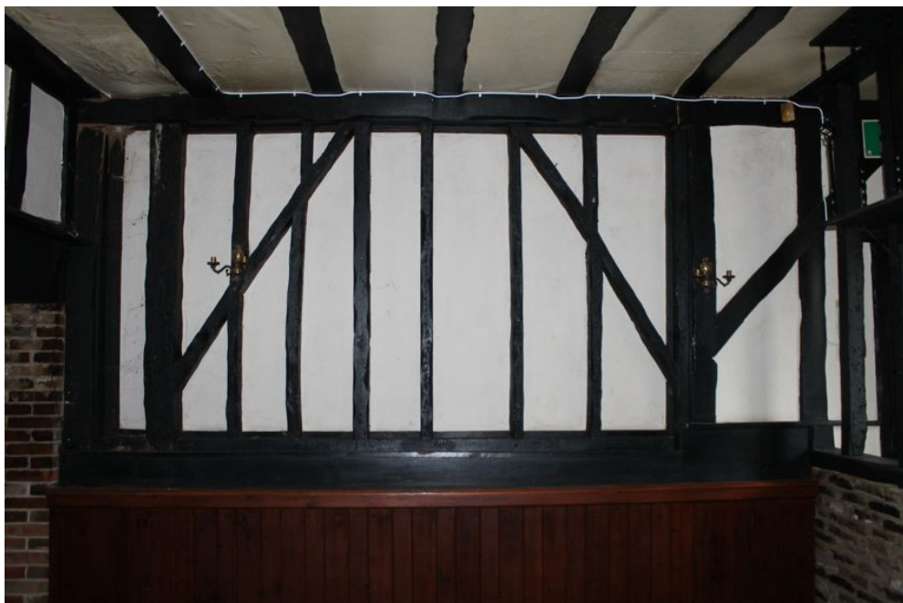
Photograph 40 Stud-work on north-east elevation of Structure F, including some re-used timbers. Photograph taken facing north-east.
