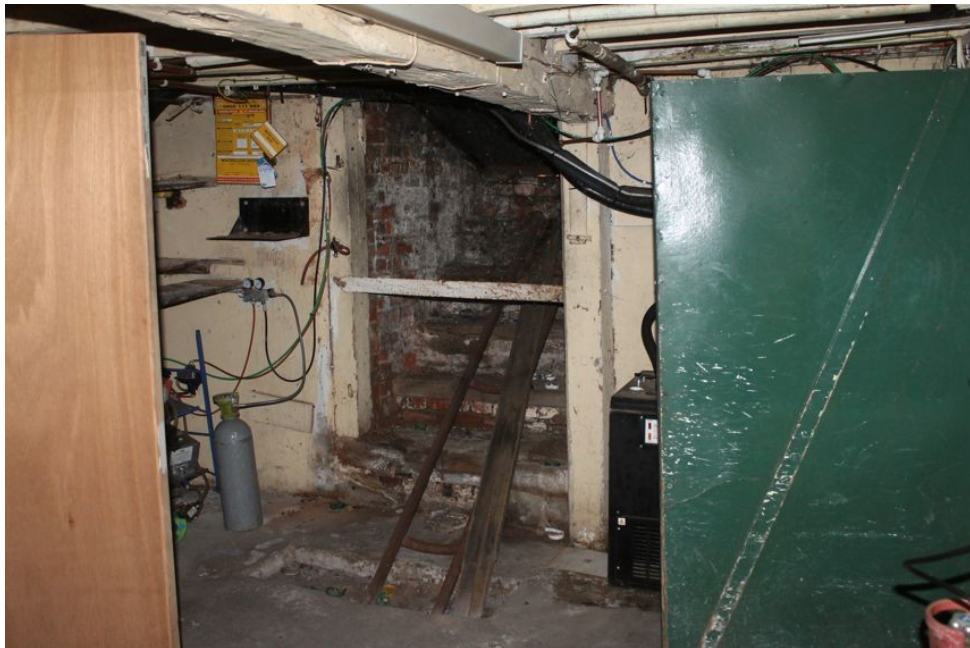
Photograph 30 Cellar below Structure C, showing barrel chute from pavement. Photograph taken facing east.
