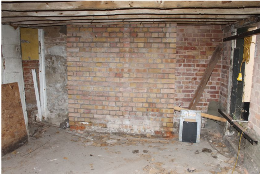
Photograph 21 Rebuilt chimney-stack of Rising Sun, visible in basement of Structure 2. Photograph taken facing east.
