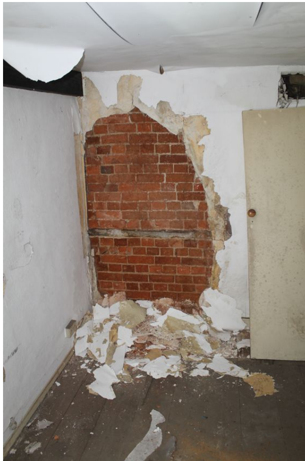
Photograph 17 Exposed English-bond brickwork on first-floor of Rising Sun. Photograph taken facing north-east.
