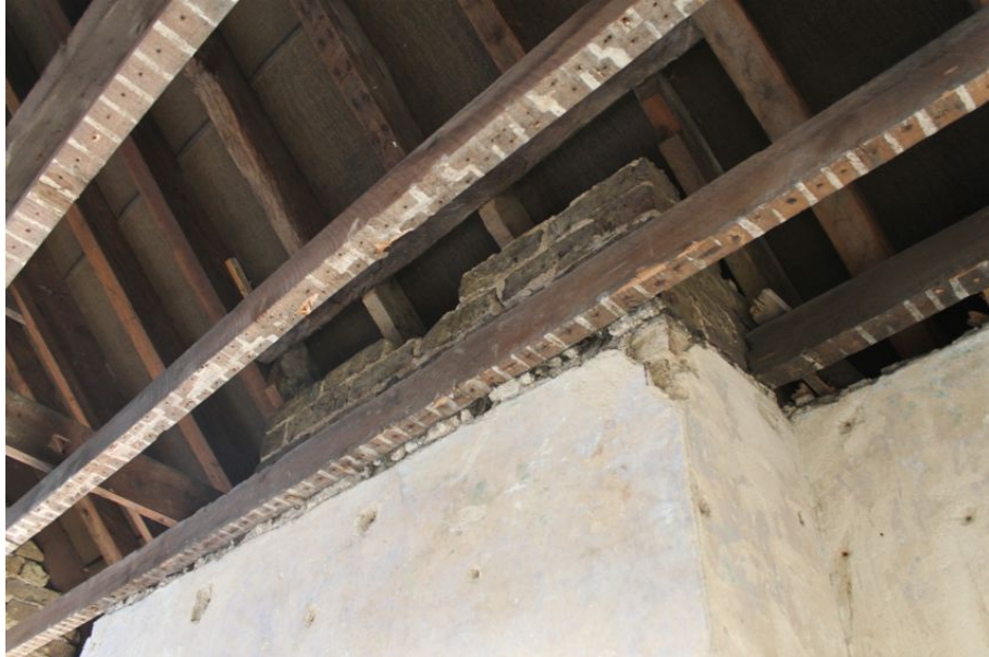
Photograph 52 Top of chimney-stack in Structure 5, having been removed to below the rafters. Note the modern rafters above it. Photograph taken facing north-west.
