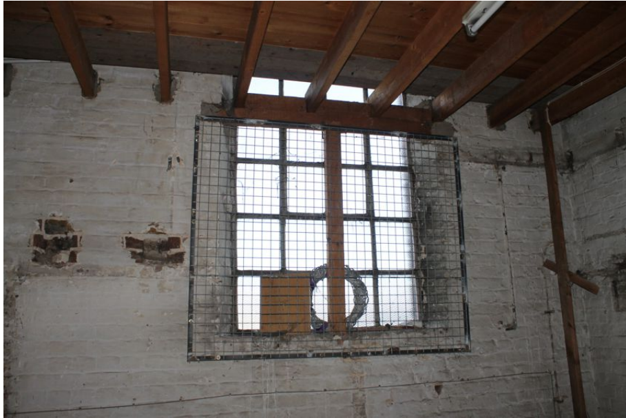
Photograph 78 Window opening bisected by insertion of second-floor in Structure 7. Photograph taken facing south-east.
