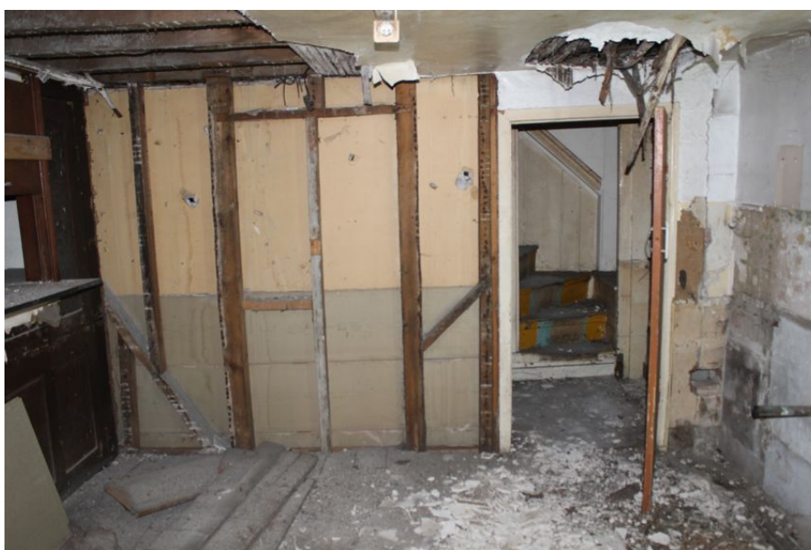
Photograph 15 Eastern wall of south-west room on ground-floor of Rising Sun. Blocked doorway visible to left of frame, inserted doorway visible to right. Photograph taken facing north-east.
