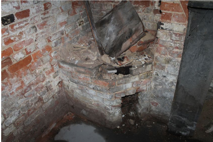
Photograph 44 Brick-built water heater in eastern room of Structure 5's basement adjacent to fireplace. Photograph taken facing north-west.
