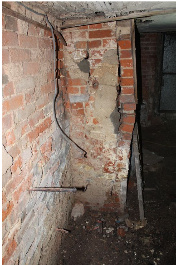
Photograph 24 Eastern side of fireplace in northern room of house extension, showing damage. Photograph taken facing south-west.
