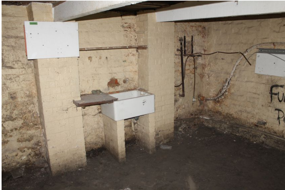
Photograph 10 Basement of the Rising Sun, showing inserted brick plinths supporting modern beams in north-east room. Photograph taken facing south-east.
