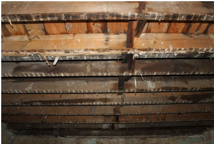
Photograph 48 Underside of second-floor in Structure 5, showing supporting herringbone-strutting. Photograph taken facing north.
