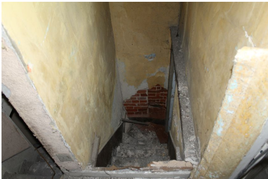
Photograph 30 Southern staircase, view from the first-floor. Note top step is boarded over. Timber to right of frame would have supported boards covering whole staircase. Also visible at bottom of staircase is exposed brickwork with joint and queen closers. Photograph taken facing north-east.
