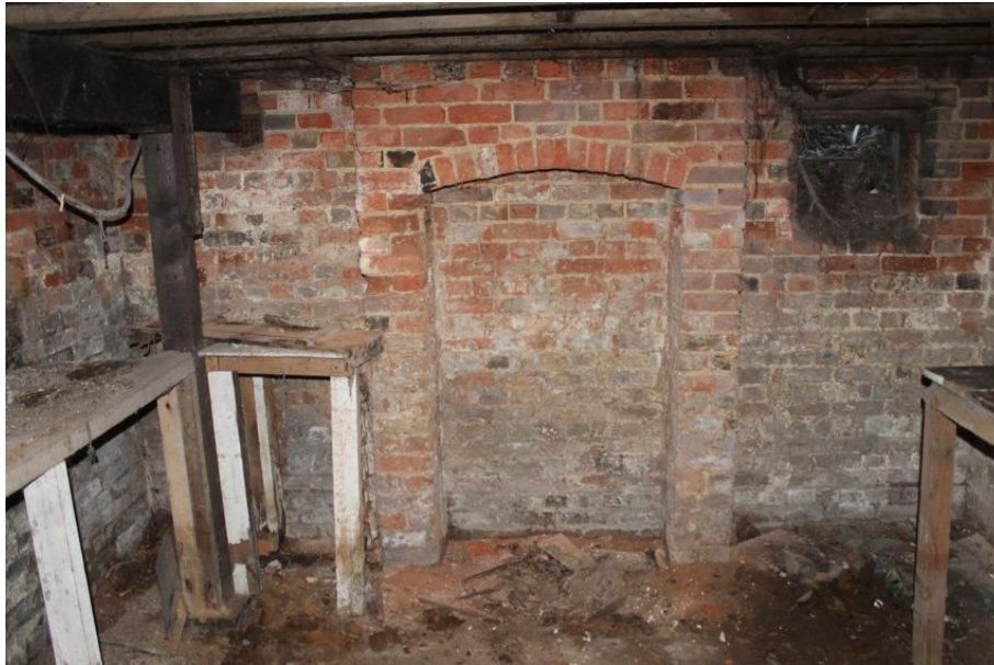
Photograph 43 Fireplace in western room of basement in Structure 5. Photograph taken facing north.
