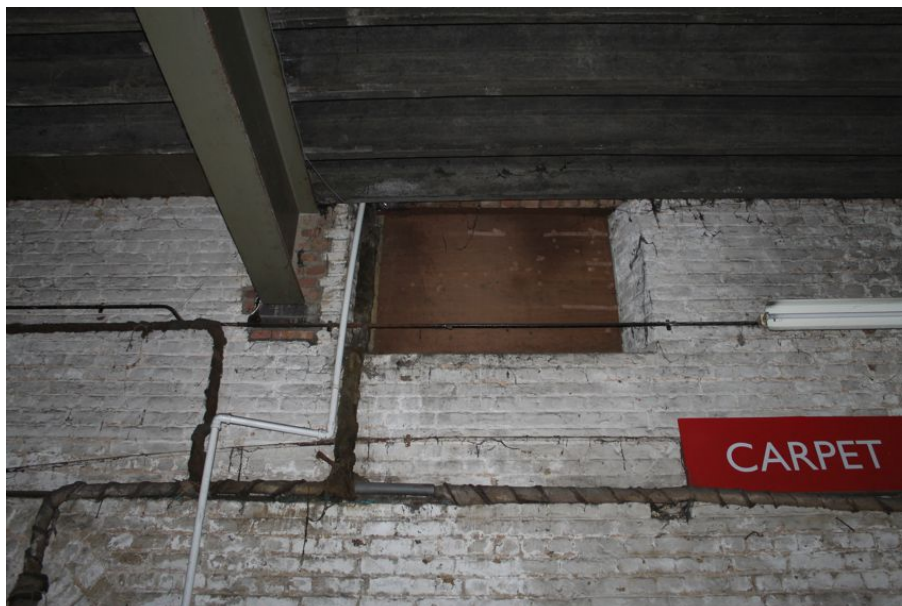
Photograph 64 Metal-beam supporting inserted first-floor of Structure 6, adjacent to a bisected window opening. Photograph taken facing north.
