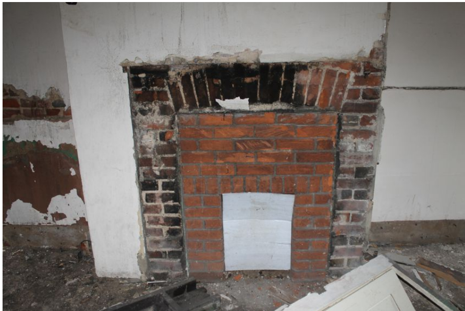
Photograph 47 Partially blocked fireplace in eastern room on ground-floor of Structure 5. Photograph taken facing north.
