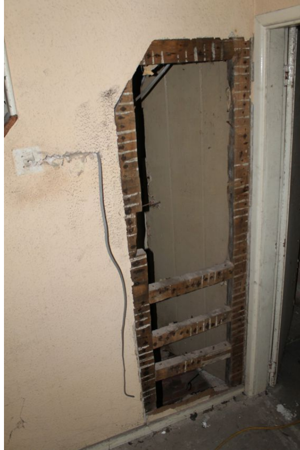
Photograph 29 Partially boarded over original door to basement in north-east room of ground-floor in Structure 2. Photograph taken facing south.
