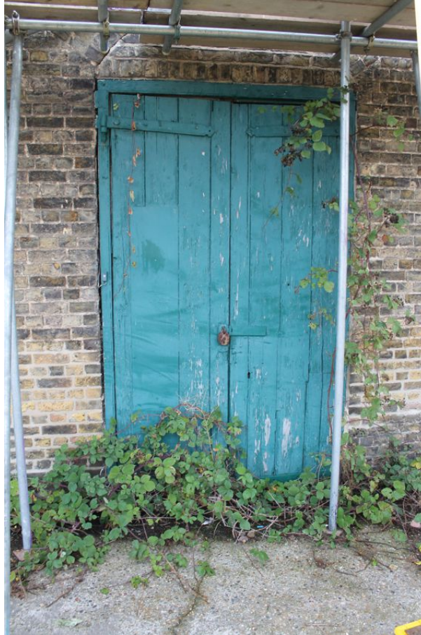
Photograph 69 Vertical-planked door on western elevation of Structure 7 (blocked from the inside). Photograph taken facing east.
