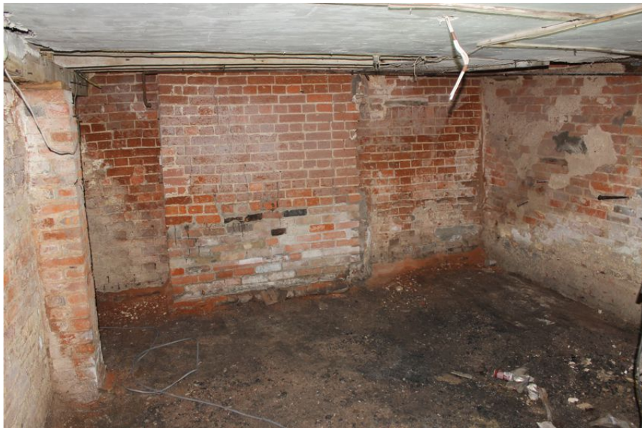
Photograph 26 Northern room of Structure 2's basement, showing west wall of Rising Sun. Note the central structural wall of the house extension (to right) is not bonded to the pub's walls. Photograph taken facing east.
