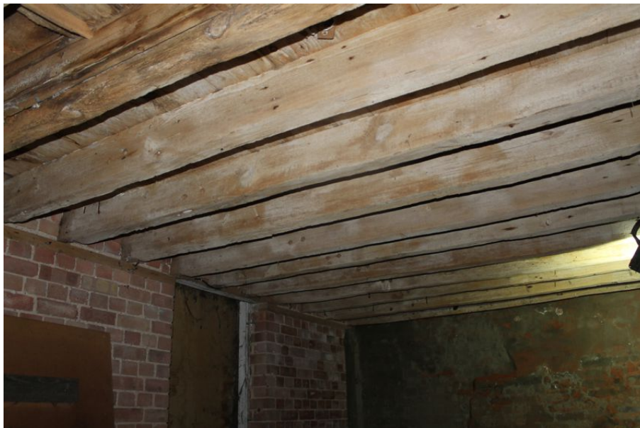
Photograph 27 Joists supporting ground-floor, view from southern room of basement in Structure 2. Photograph taken facing south.
