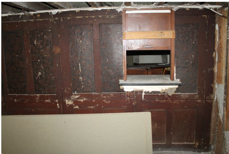
Photograph 14 Decorated wooden panels and inserted serving hatch in south-west room on ground-floor of Rising Sun. Photograph taken facing north-west.
