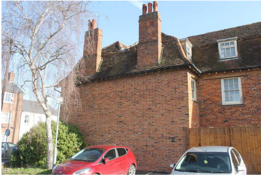
Photograph 3 Western elevation of 79 Magdalen Street. Two chimney-stacks visible on main range. Photograph taken facing north-east.
