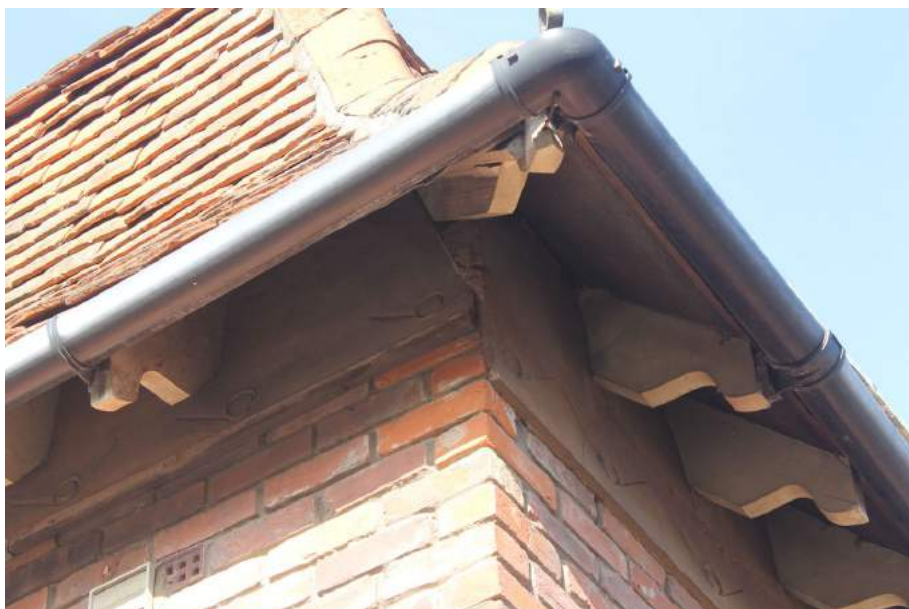
Photograph 2 Detail of cornice around entire building. Chamfered rafter-ends and incised cement shown.
