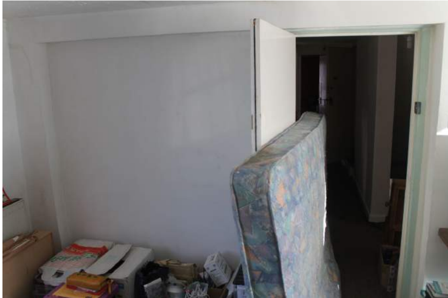
Photograph 24 View from extension showing entrance into main range on first-floor, alongside possible blocked entrance or window. Photograph taken facing north.
