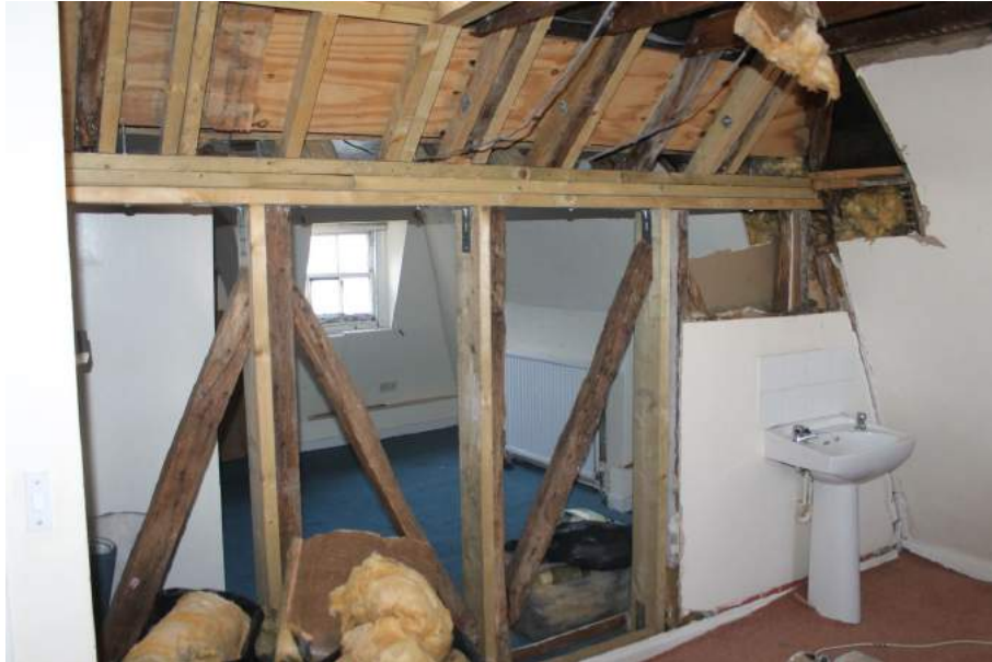
Photograph 26 Timber wall between north-west and south-west room in main range on second-floor. Mixture of modern machine-cut and historic hand-sawn timber visible. Photograph taken facing south-west.
