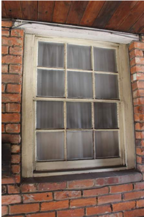
Photograph 10 Sash window on west side of passageway on ground-floor. Photograph taken facing west.
