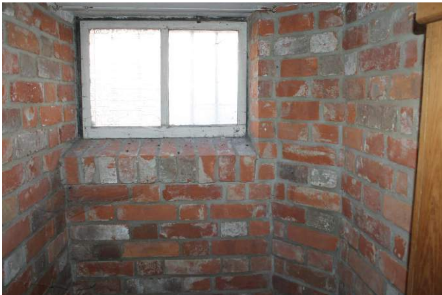
Photograph 15 Fixed window in cellar below bay window on ground-floor. Rebuilt brickwork around. Photograph taken facing north.
