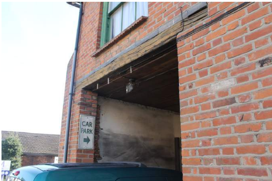
Photograph 6 Entrance into passage leading to rear of building on northern elevation. Substantial timber lintel visible. Photograph taken facing south-east.
