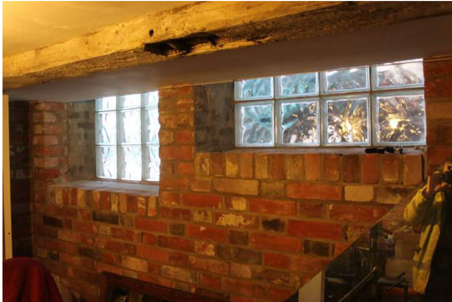
Photograph 14 Hammered-glass windows on east side of cellar, looking out onto passageway. Photograph taken facing north-east.
