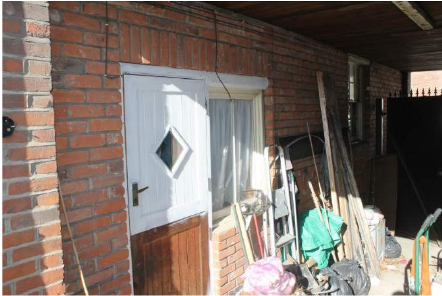
Photograph 9 Western wall of passageway on ground-floor of 79 Magdalen Street, showing rebuilt wall. Photograph taken facing north-west.
