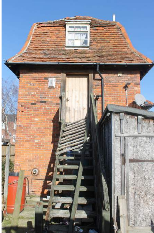
Photograph 11 Southern elevation of extension, showing staircase up to first-floor door. Photograph taken facing north.
