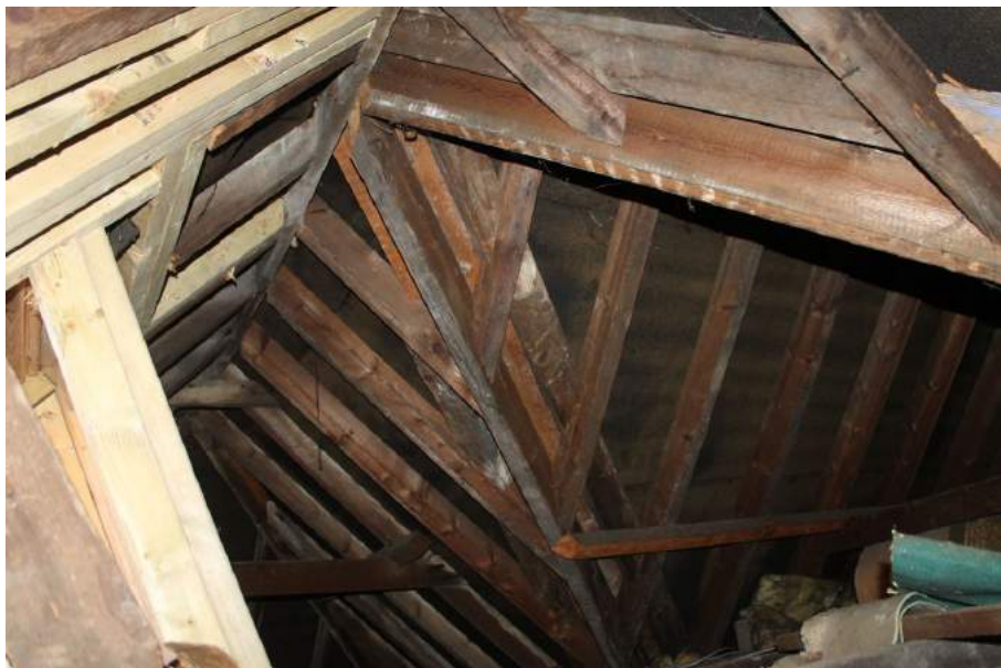
Photograph 27 Roof structure, showing extension's roof to right attaching to main ranges roof. Photograph taken facing east.
