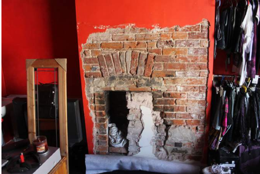
Photograph 22 Blocked then partially reopened northern fireplace on first-floor. Photograph taken facing west.
