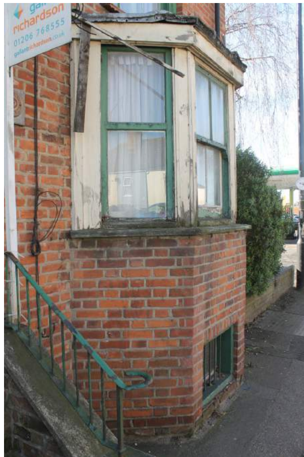
Photograph 4 Bay window on northern elevation of 79 Magdalen Street. Photograph taken facing south-west.
