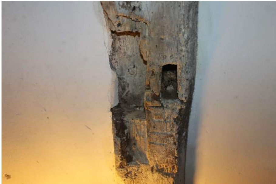
Photograph 17 Detail of empty mortise and carpenter's mark "IIII" on underside of joist in cellar.
