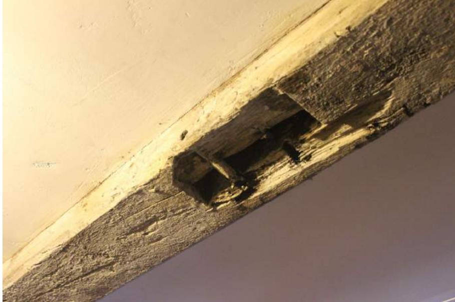
Photograph 16 Detail of empty mortise on joist in cellar. Photograph taken facing north-east.
