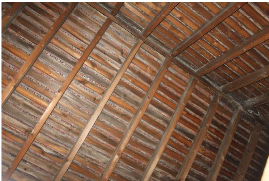
Photograph 18 Detail of roof structure in No 10, showing rafter pairs rising to a ridgeboard with no collar support.
