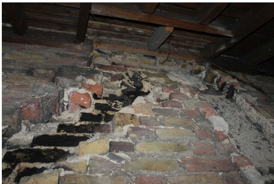
Photograph 13 Remains of chimney in the attic space of No 11's south-west wing. Photograph taken facing south-east.
