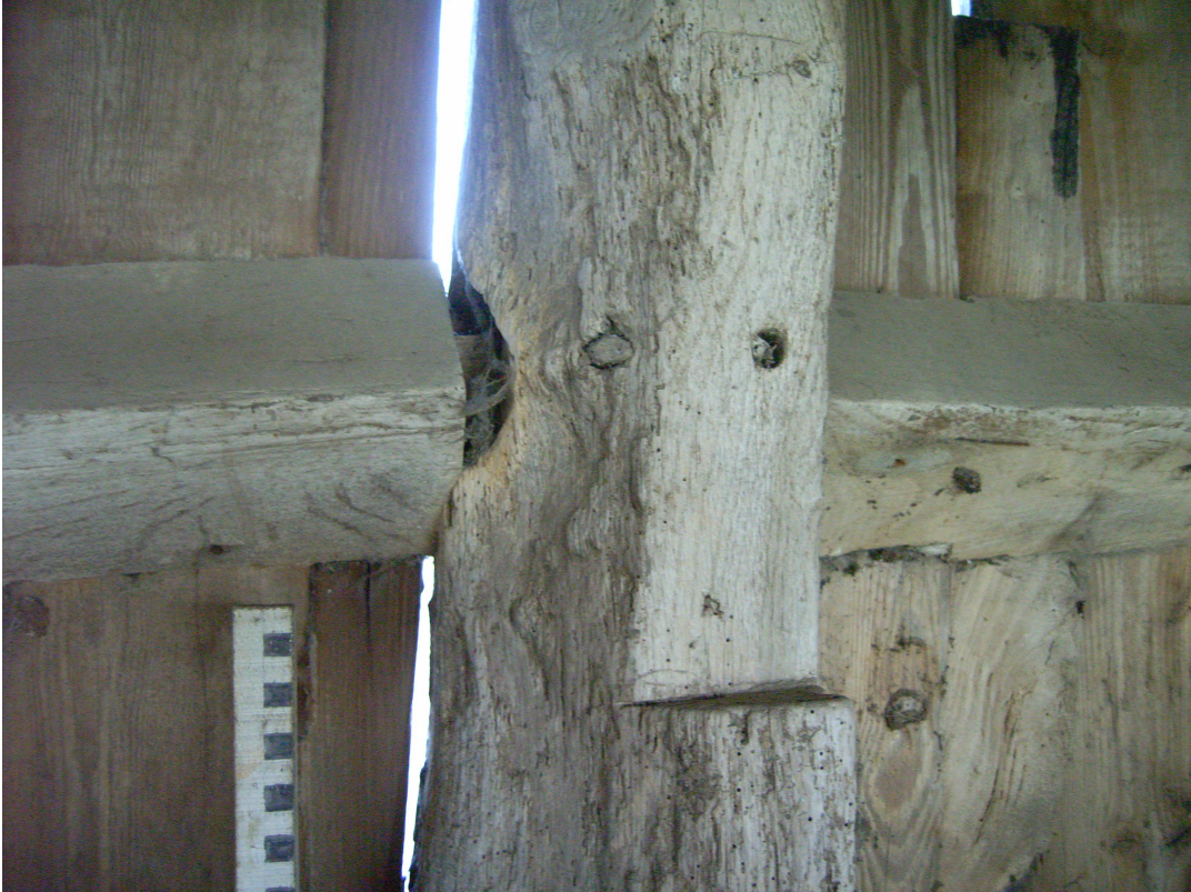
A2.13 Shed (3). Detail of a typical junction of the upper triangular rails with a post of the rear elevation, showing pegged tenons.
