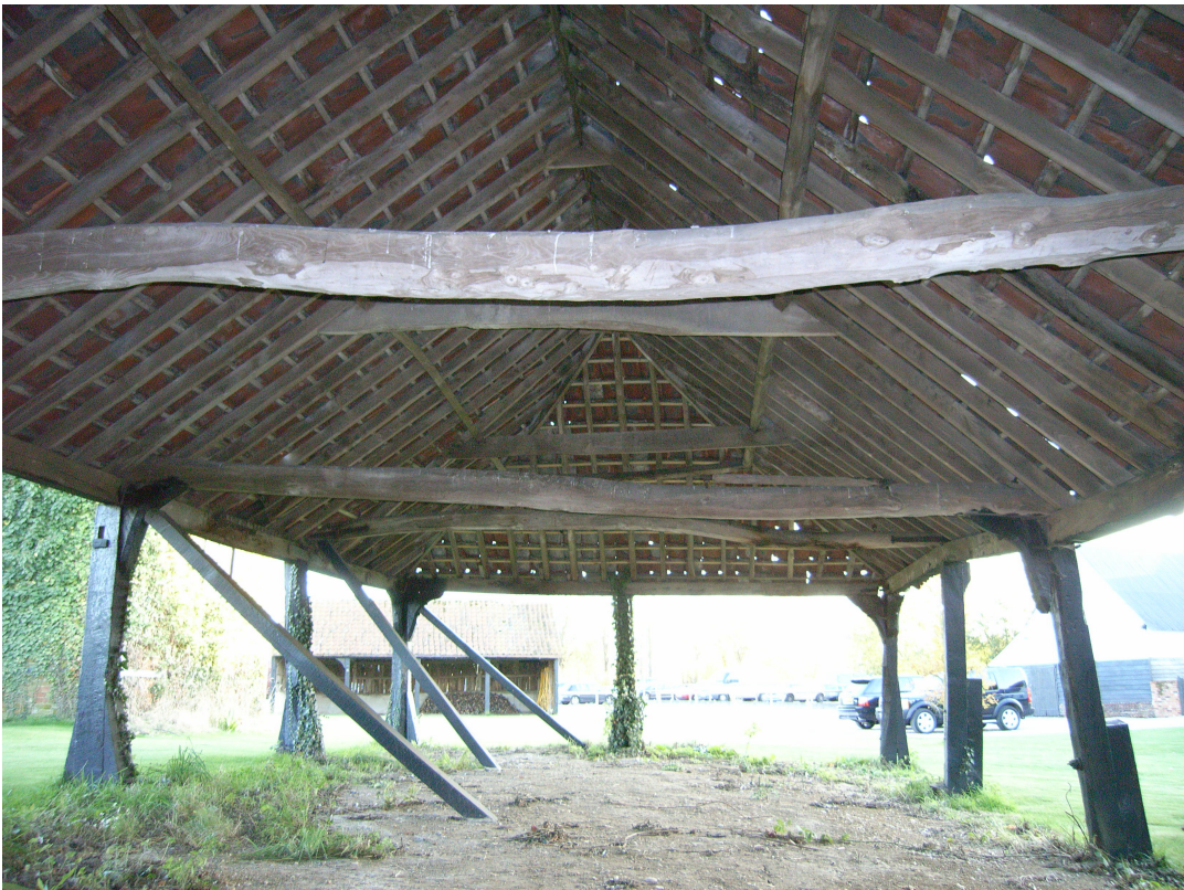
A2.6 Cart Lodge (1). Interior from north towards gable B-D. The diagonal props are recent.
