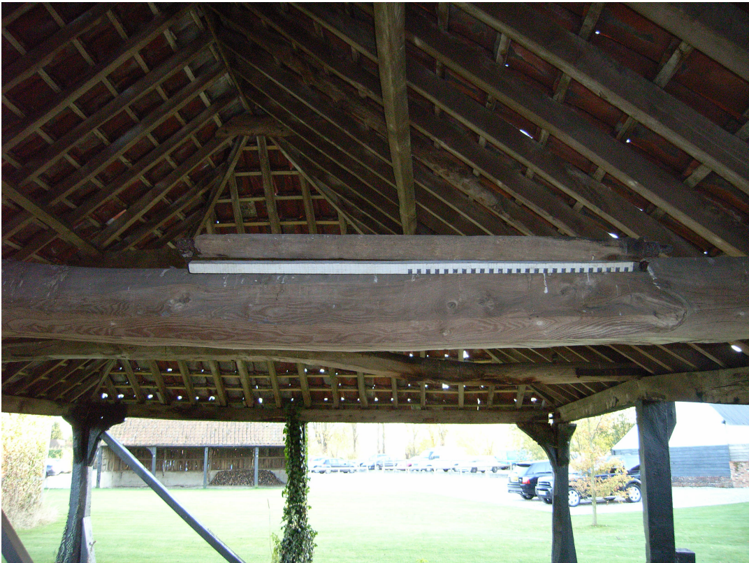
A2.8 Cart Lodge (1). Wooden roller on central tie-beam seen from north with 1 metre scale rod.
