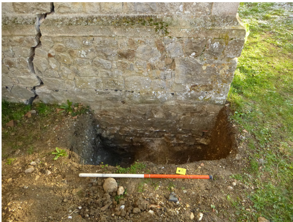
Photograph 1 Test-pit showing foundation of nave and south-west buttress. Substantial crack in wall visible to left. Photograph taken facing east.
