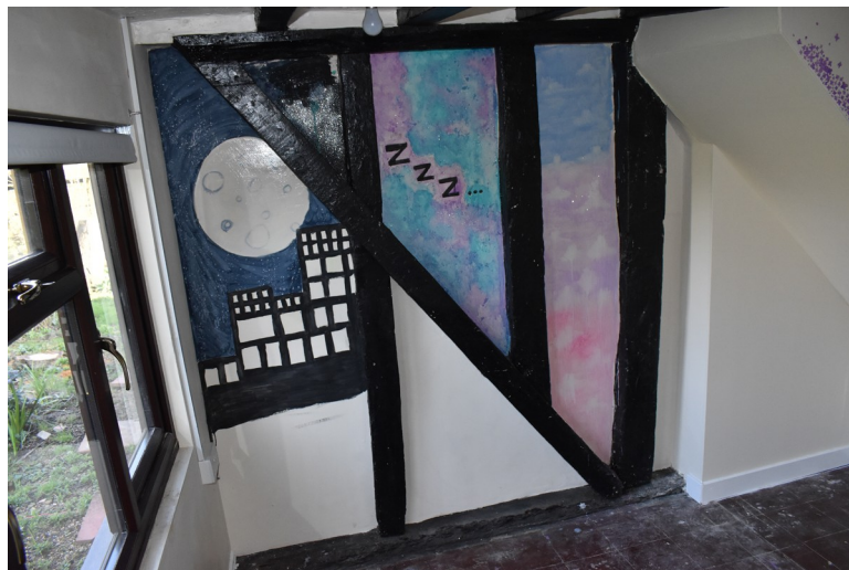
Photograph 12 Detail of exposed studwork in room 7, showing girding-beam cut short and supported by modern brace. Photograph taken facing north-east.
