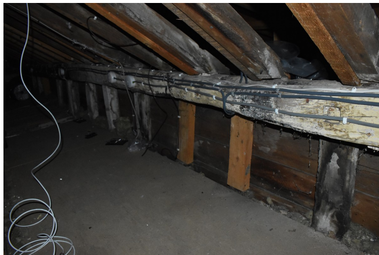
Photograph 25 Detail of eastern wall-plate of the building in the attic. Original studs visible, as well as modern replacements. Photograph taken facing east.
