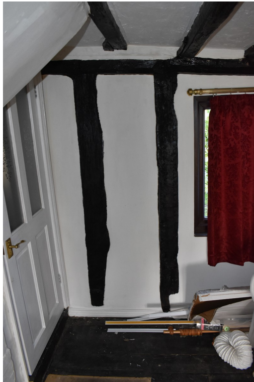
Photograph 14 Cut-off studs on the western wall of room 8. Photograph taken facing north-west.
