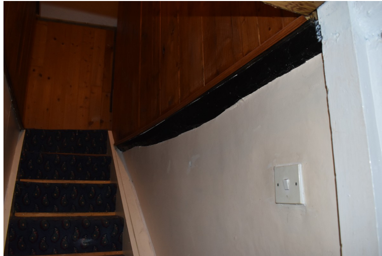
Photograph 9 Interior of room 6, showing chamfered girding-beam and staircase up to attic floor. Photograph taken facing north.
