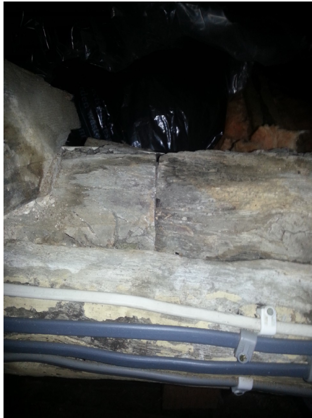
Photograph 27 Detail of possible scarf joint on eastern wall-plate, with timber addition to face of wall-plate visible. Photograph taken facing south-east.
