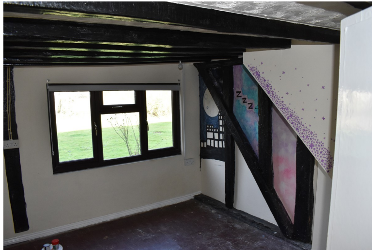
Photograph 11 Interior of room 7, showing exposed timber-frame, joists and inserted staircase. Photograph taken facing north.
