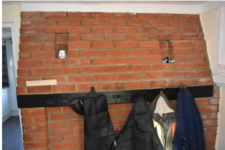
Photograph 19 Rebuilt chimney-breast in room 9, with imitation mantel-beam and blocked fireplace opening. Photograph taken facing north-west.
