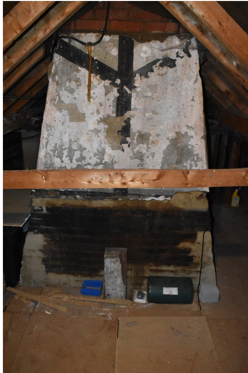
Photograph 24 South side of chimney-stack in room 15, showing exposed original brickwork. Photograph taken facing north-east.
