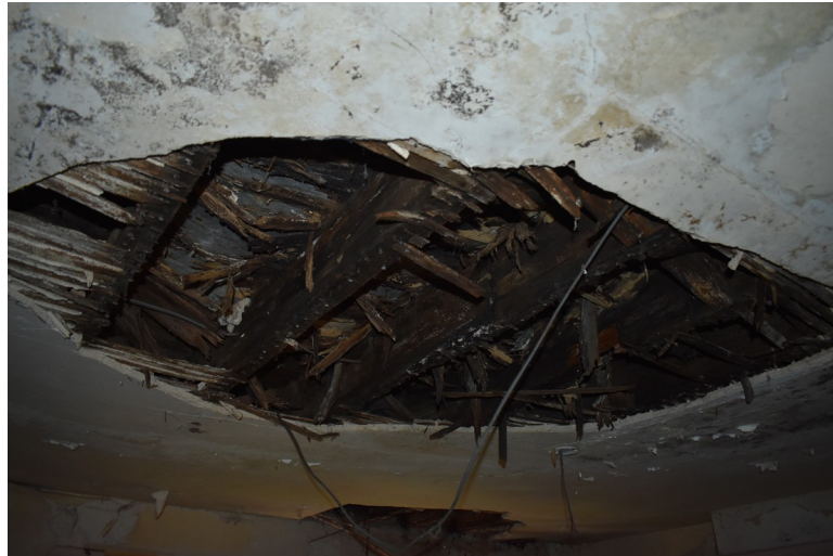
Photograph 11 Detail of damaged ceiling above room 1b, showing exposed joists. Photograph taken facing west.
