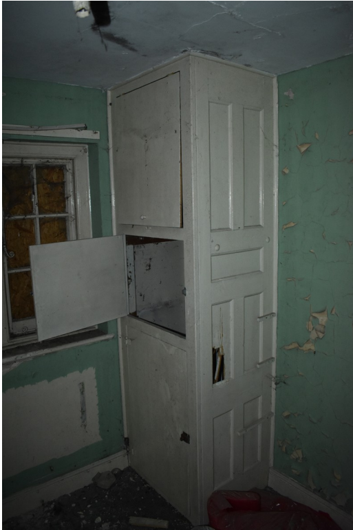
Photograph 22 Original cupboard in room 9a, with modern doors. Photograph taken facing east.
