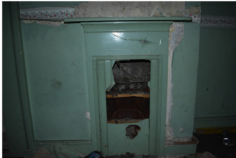
Photograph 21 Detail of fireplace in chimney-breast of room 8a. Photograph taken facing south-east.
