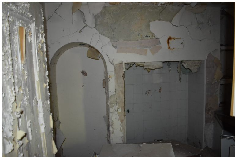
Photograph 15 Room 3b, with stoking hole visible above alcove. Photograph taken facing north-west.
