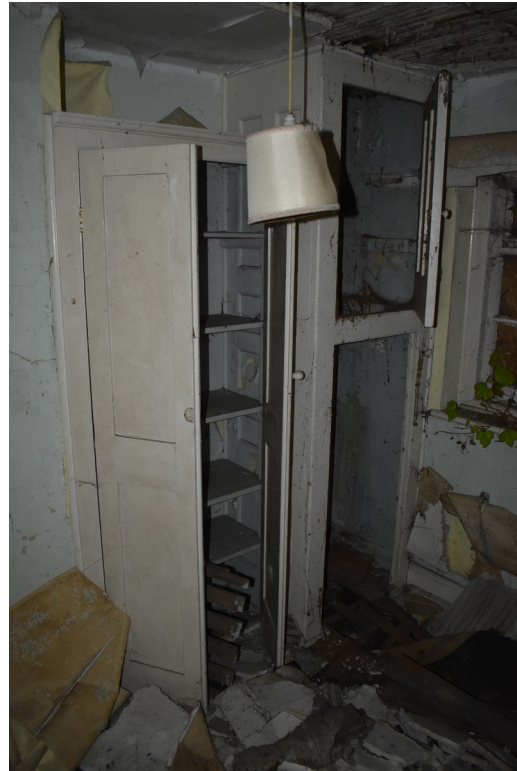
Photograph 23 Original cupboard in room 9b (right), with inserted cupboard alongside (left). Photograph taken facing north.
