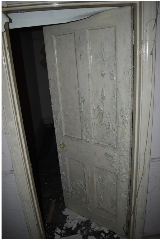
Photograph 9 Example of original door with bakelite handle, leading into room 2b. Photograph taken facing south-west.
