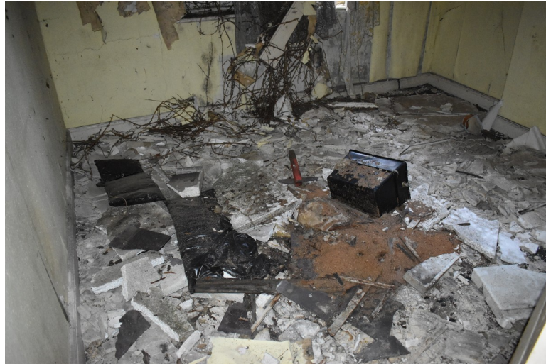
Photograph 20 Room 7b, showing damaged caused by collapsed ceiling. Photograph taken facing south-east.
