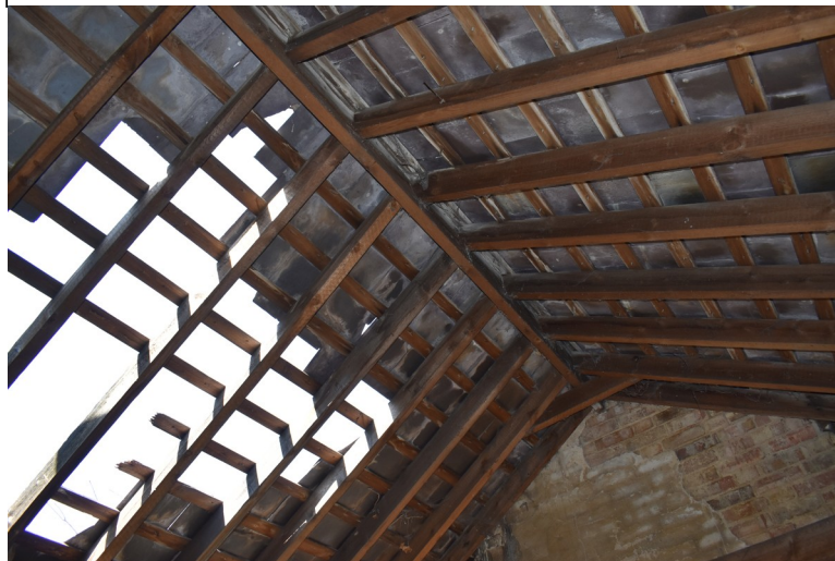
Photograph 26 Roof structure above rooms 7b and 9b, showing damage to roof fabric. Photograph taken facing west.
