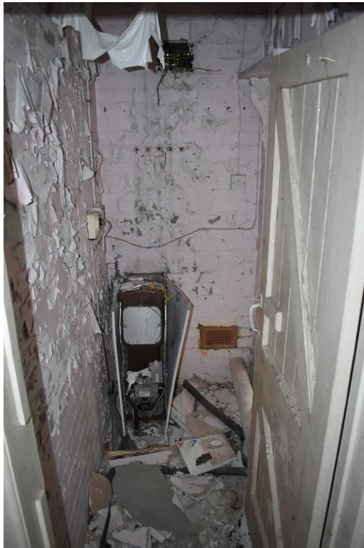
Photograph 18 Room 6a, showing vertical-planked door, visible brickwork and vent. Photograph taken facing north-east.
