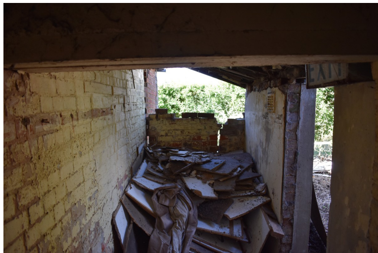
Photograph 26 Interior of western extension, showing damaged north-west elevation. Photograph taken facing north-west.
