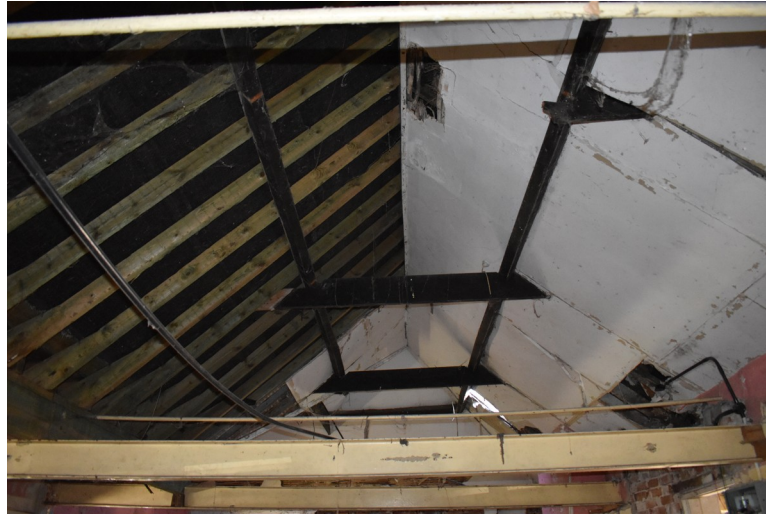
Photograph 21 Detail of roof structure above cross-wing. Rafters on left side are replacement timbers. Photograph taken facing north-west.
