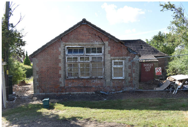
Photograph 15 North-west elevation of building, showing inserted windows in original partially bricked-in window openings. Photograph taken facing south-east.
