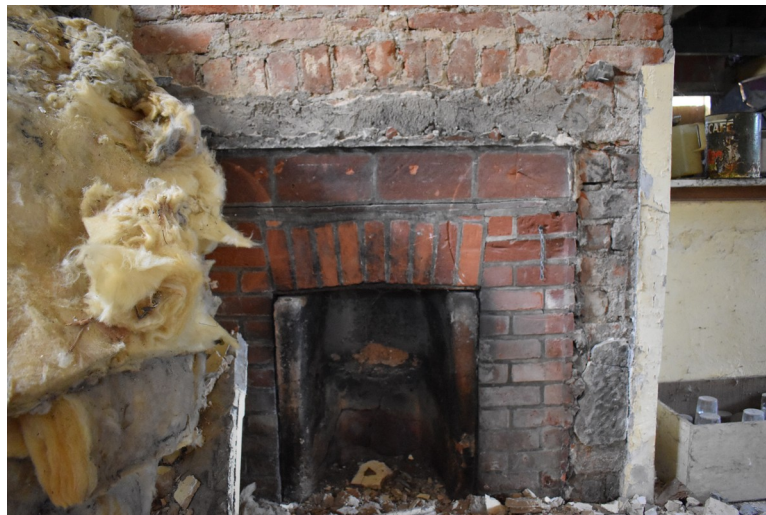
Photograph 24 Detail of inserted fireplace in chimney-breast on south-east elevation of northern room. Arch of original fireplace visible above. Photograph taken facing south-east.
