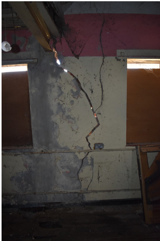
Photograph 19 Serious structural problems evident on south-east elevation of southern room. Photograph taken facing south-east.
