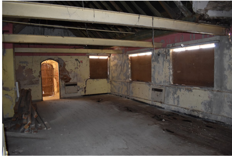
Photograph 16 Southern room of building, showing metal beams and damaged floorboards. Photograph taken facing east.
