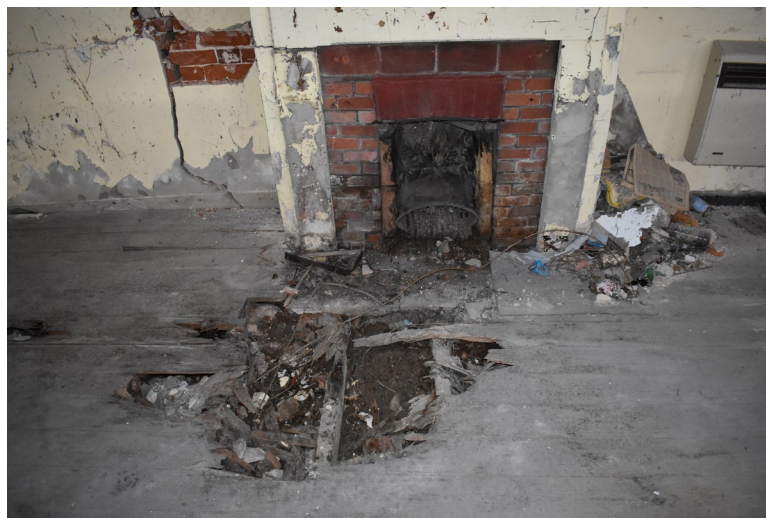
Photograph 17 Detail of inserted fireplace in western chimney-breast of southern room. Damaged section of floor visible in front. Photograph taken facing north-west.
