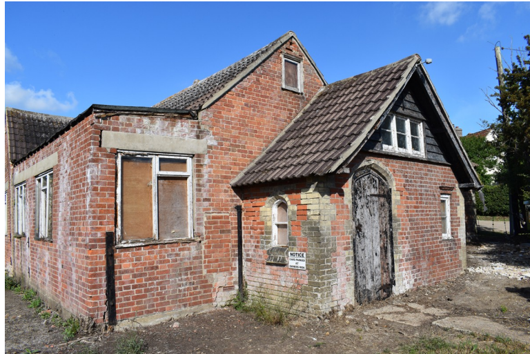
Photograph 11 North-east and south-east elevation of building. Note postbox visible in earlier photographs has been removed. Photograph taken facing west.
