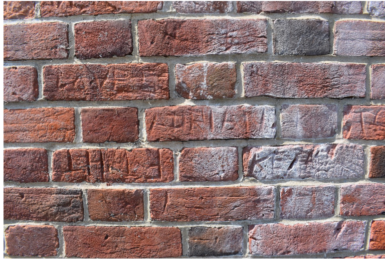
Photograph 9 Example of graffiti on south-east elevation of building. Photograph taken facing north-west.
