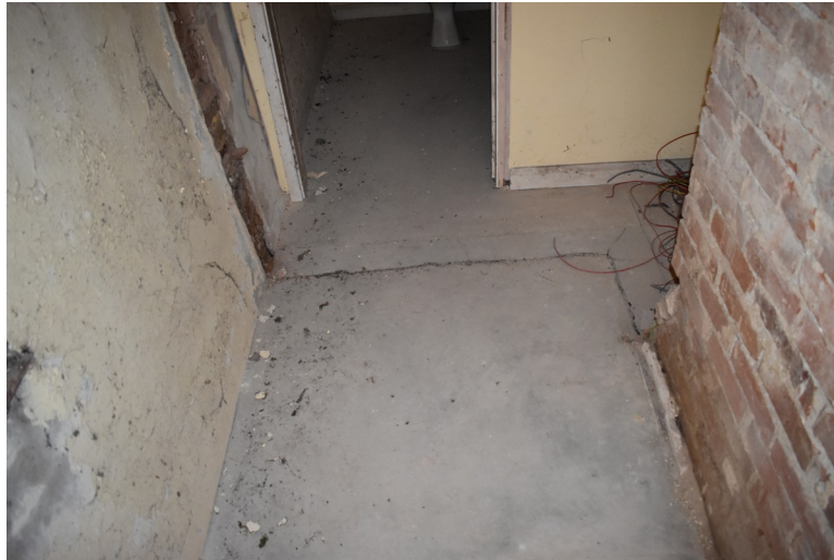
Photograph 23 Detail of scarring on floor of north room, showing location of original brick wall forming end of corridor. Location of original entrance into building to the left. Photograph taken facing north-west.
