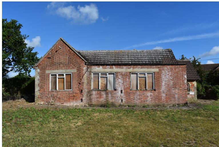
Photograph 8 South-east elevation of building. Note structural damage and modern windows with substantial concrete lintels. Photograph taken facing north-west.
