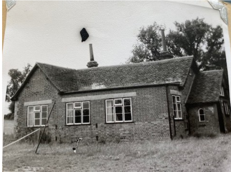
Photograph 5 South-east elevation of the building, taken sometime between 1950-1975. Photograph taken facing north-west. ERO D/DU 1464/42.
