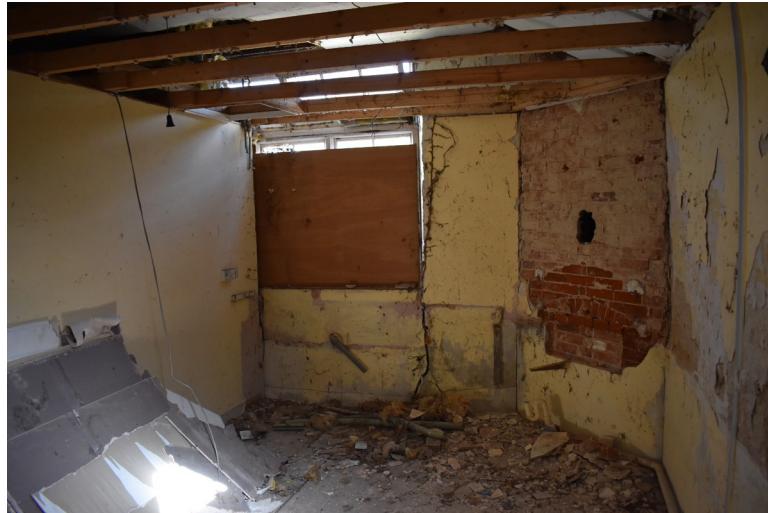
Photograph 25 Northern room of building, showing structural damage evident to room's north-west elevation. Photograph taken facing north-west.
