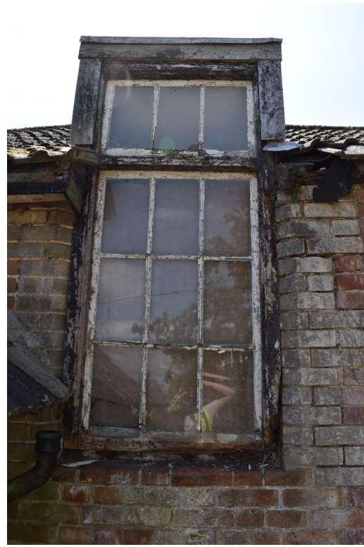
Photograph 13 Detail of dormer window on north-east elevation of original range. Photograph taken facing south-west.
