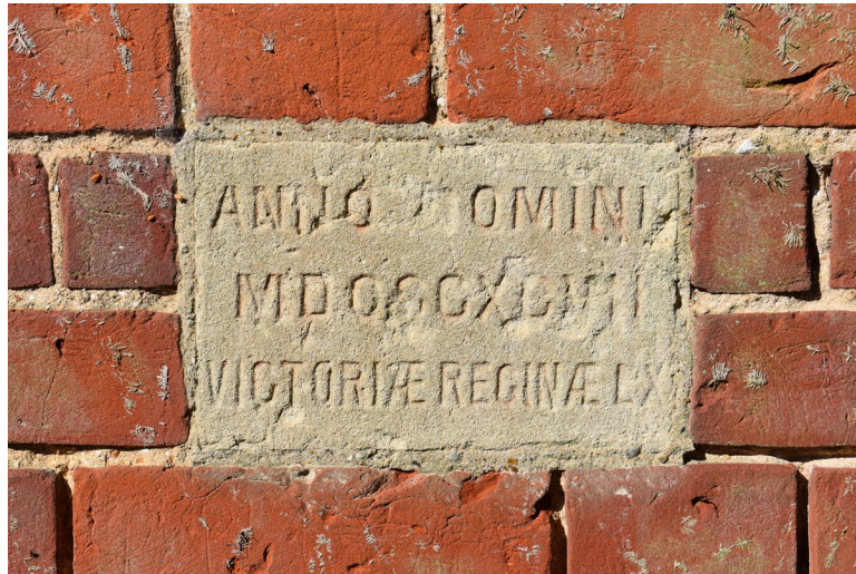
Photograph 14 Detail of tablet stone on north-east elevation of main range, commemorating Queen Victoria's Diamond jubilee. Photograph taken facing south-west.
