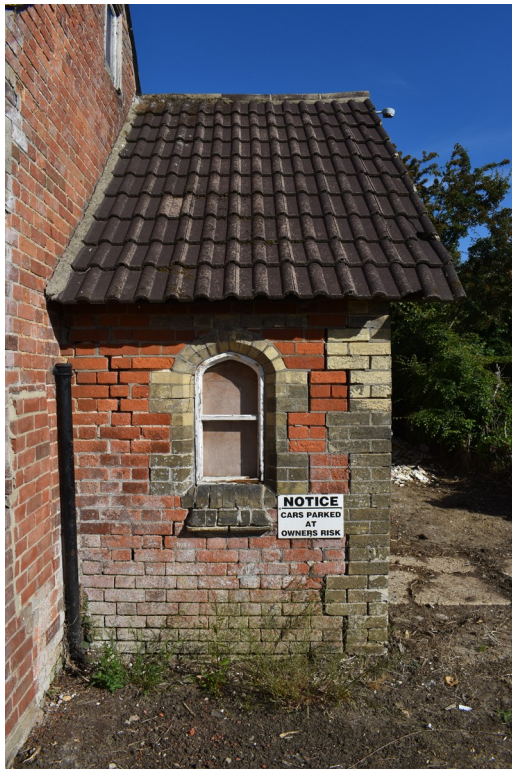
Photograph 10 South-east elevation of porch extension, showing small fixed window. Photograph taken facing north-west.
