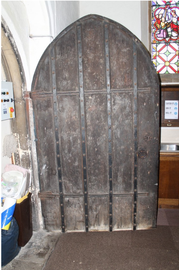
Photograph 9 Front of door between southern aisle of church and porch. Photograph taken facing west.
