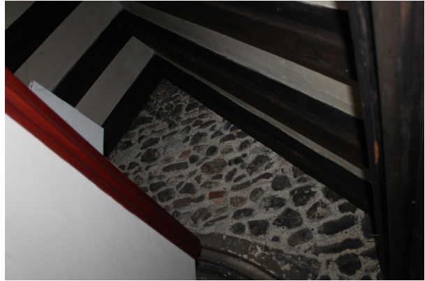
Photograph 7 Interior of porch, showing south wall of church, as well as rafters of porch. Photograph taken facing north-west.
