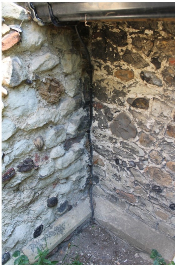
Photograph 4 Detail of join between western elevation of porch (to right) and wall of southern aisle (to left). Photograph taken facing north-east.
