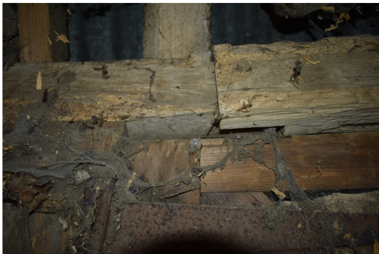
Photograph 14 Detail of face-halved scarf in bay 2, above double-doors on north-east elevation. Photograph taken facing north-east.
