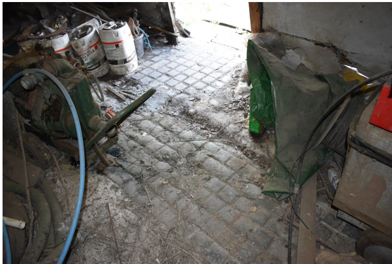
Photograph 13 Detail of surviving cobbled floor and drainage run in bay 2. Photograph taken facing south.
