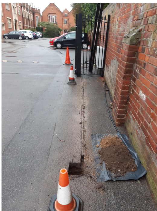
Photograph 1 An excavated hole by Gate 8 (leading onto Creffield Road), showing new gateposts in background. Photograph taken facing south.
