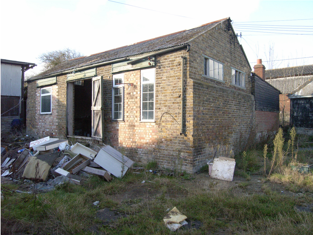
A2.8 Workshop. Exterior from south-east, showing blocked tall windows to right and left of central entrance.
