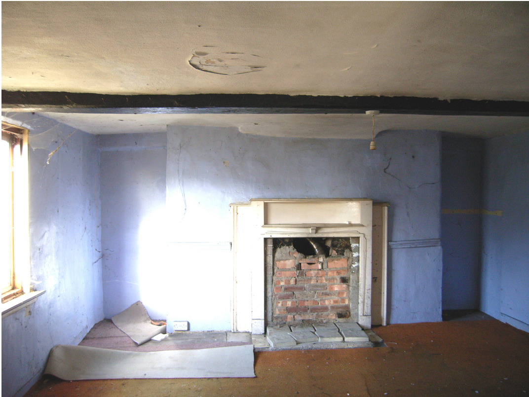
A2.3 Farmhouse. Internal northern gable, showing altered 18th-century fireplace on ground floor.
