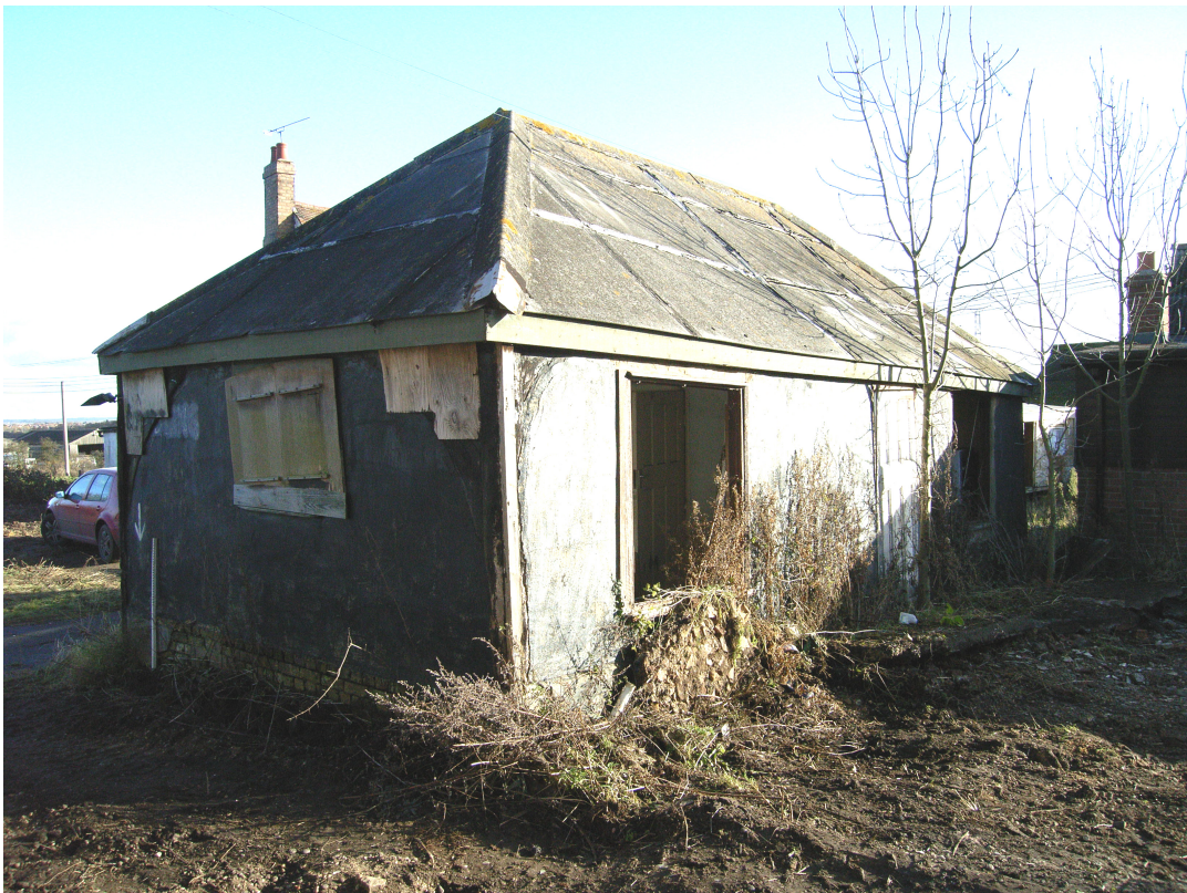
A2.4 Cart lodge. Exterior from north-west, showing massive brackets to western elevation and (left) to northern gable.
