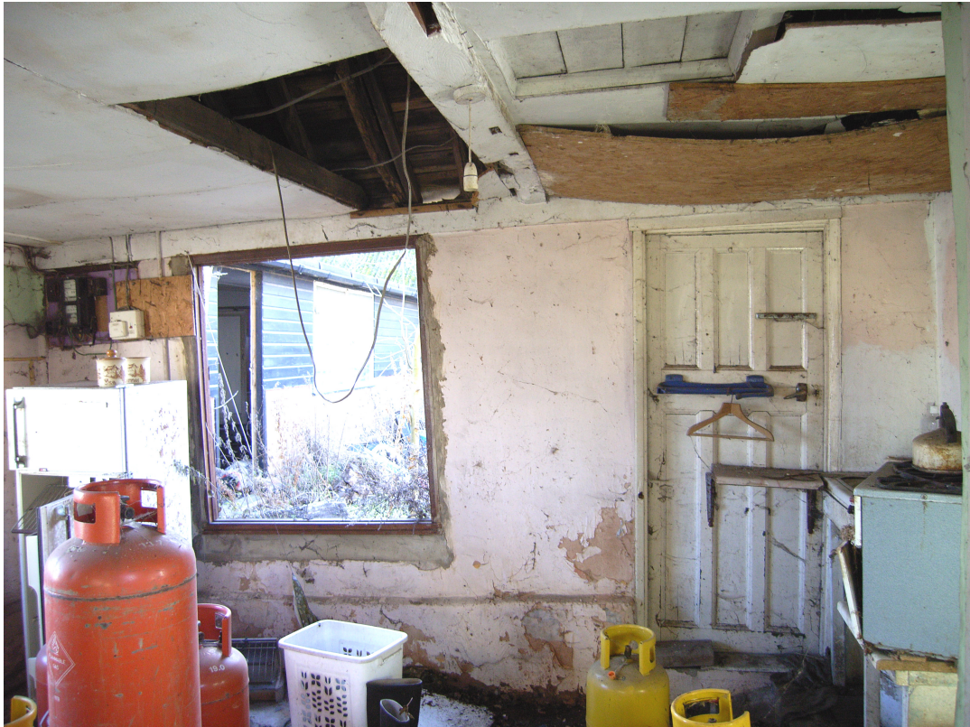
A2.5 Cart lodge. Interior of southern room, showing western elevation with empty partition mortises in tie-beam above.
