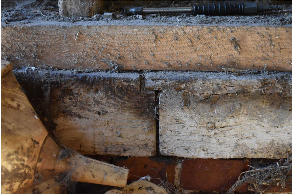
Photograph 10 Scarf joint in sill-beam on southern elevation in bay 5. Photograph taken facing south.
