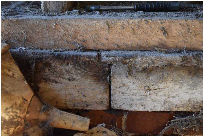
HSCF21_Phograph_081Scarf joint in sill-beam on southern elevation in bay 5...
