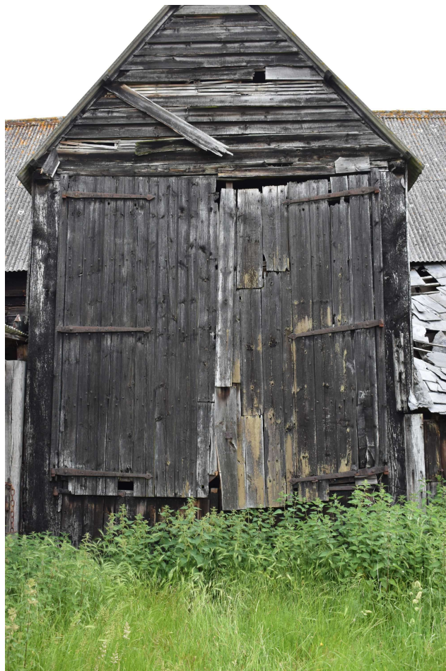
Photograph 3 Detail of mistrey doors on southern elevation of threshing barn. Photograph taken facing north.
