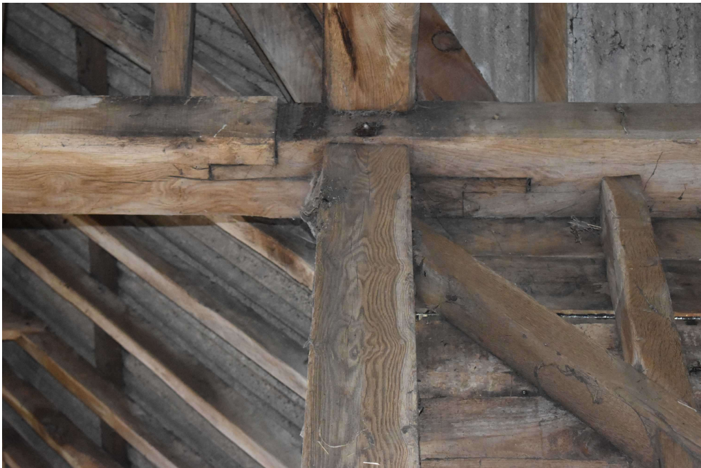
Photograph 11 Scarf joint in southern wall-plate between bays 2 and 3. Photograph taken facing south.
