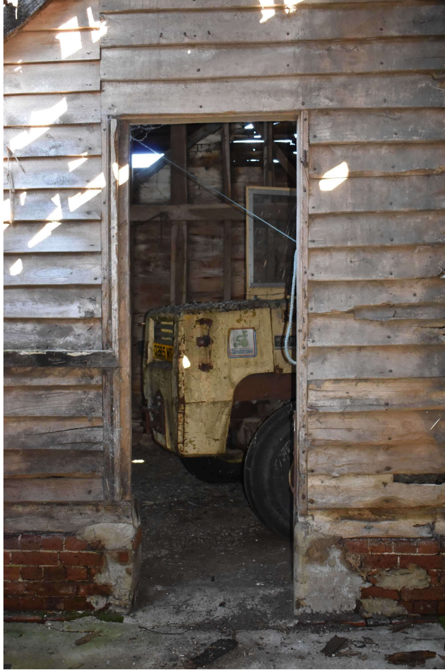
Photograph 17 Detail of doorway on eastern elevation of mistrey. Photograph taken facing west.
