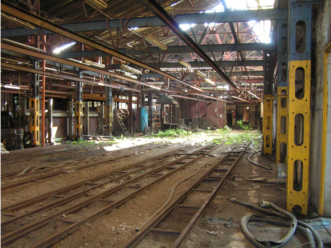
A1.18 Main foundry casting floor with overhead monorail metal-handling system, view south-east.
