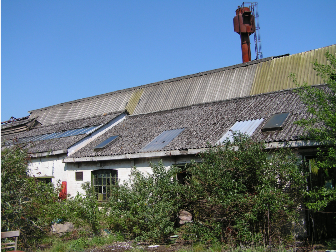
A1.3 Exterior of the pattern shop with main foundry in the background, view north-east.
