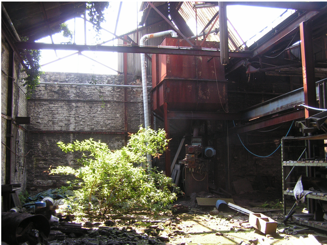
A1.10 The moulding floor with the moulding sand hopper to the right, view south-west.
