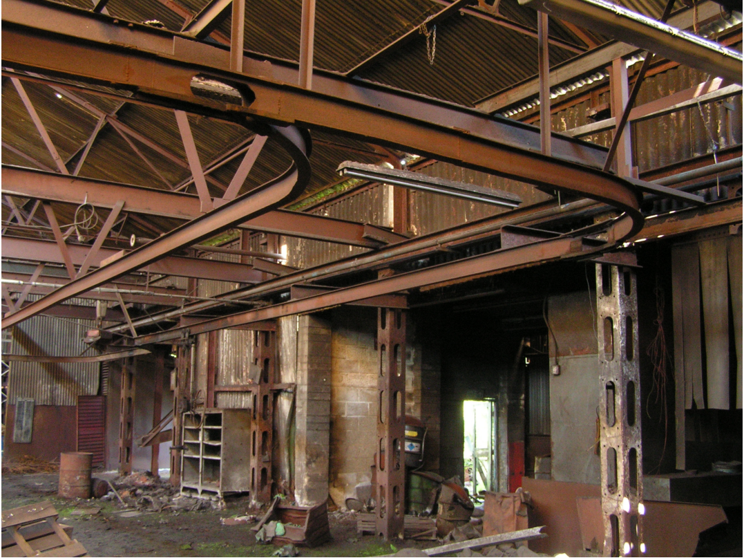
A1.15 The overhead monorail metal-handling system, view north-east.
