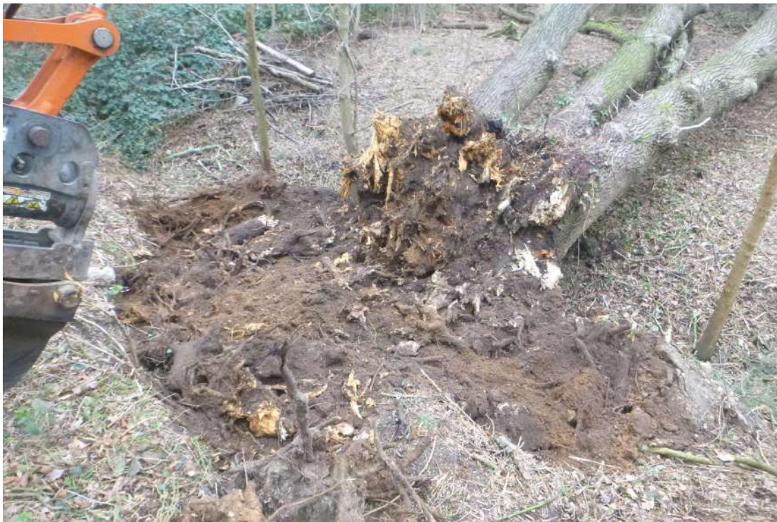
Photograph 4 Breaking up the tree roots to backfill within the tree throw, looking north-east
