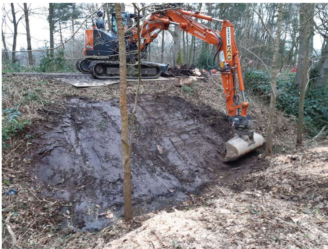
Photograph 7 Smoothing down the backfilled tree throw and reinstatement of the Berechurch Dyke, looking north-west
