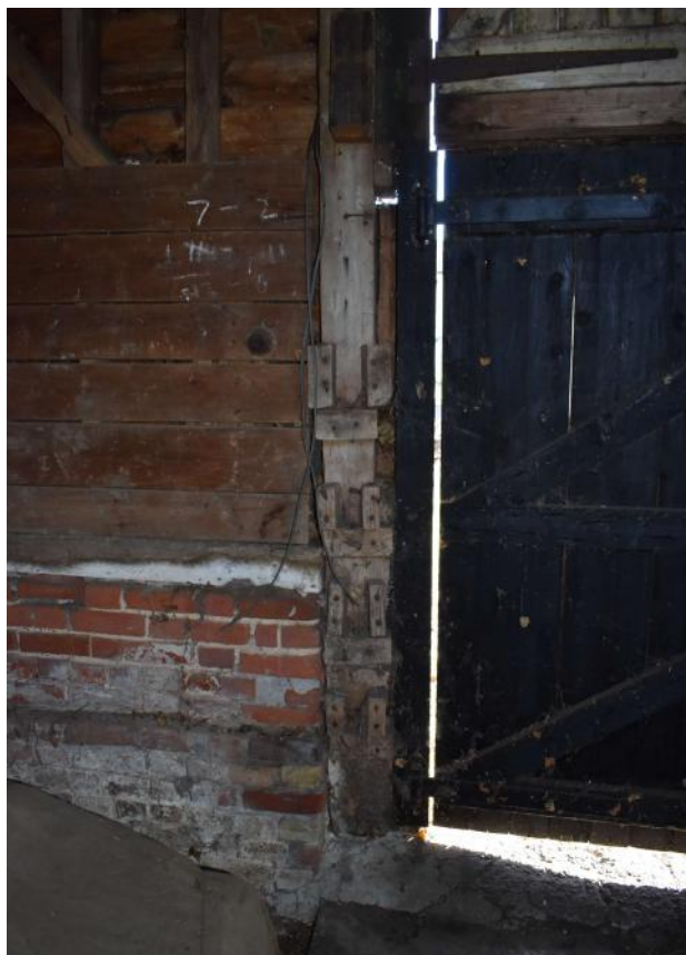
Photograph 16 Detail of wooden blocks adjacent to barn door on eastern wall. Photograph taken facing north-east.
