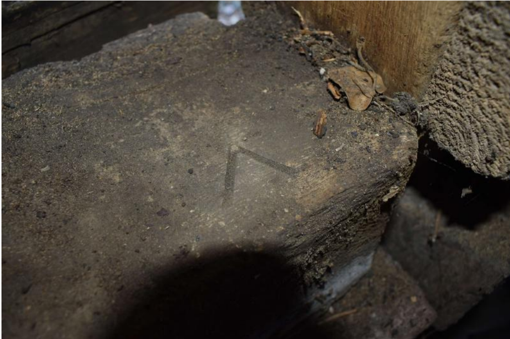
Photograph 14 Detail of carpenters' mark 'V' on sill-beam on western wall of bay 2 in barn. Photograph taken facing north.
