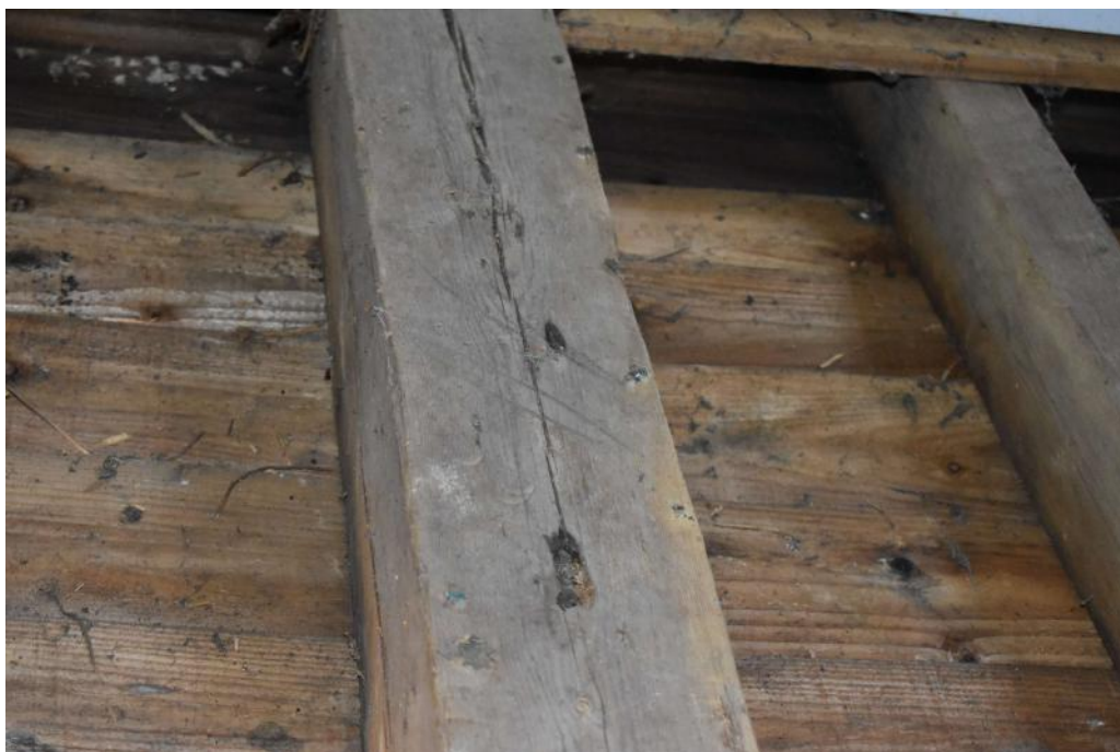
Photograph 19 Detail of Baltic timber mark on post of eastern wall between bays 4 and 5. Photograph taken facing south-east.
