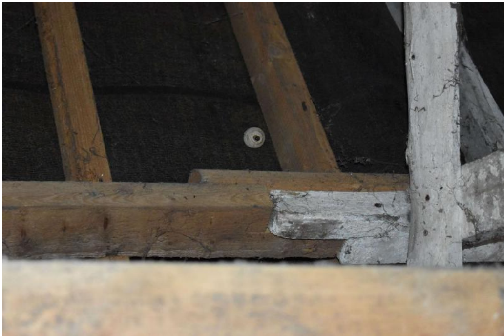
Photograph 21 Detail of scarf-joint in purlin on the northern pitch of the roof of the store 5. Photograph taken facing north.
