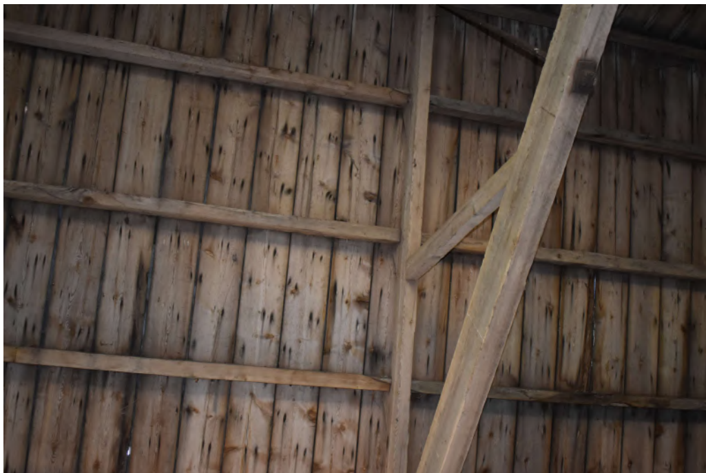
Photograph 10 Detail of scarf-joints in purlin in eastern roof pitch between bays 2 and 3 of the barn. Photograph taken facing south-east.
