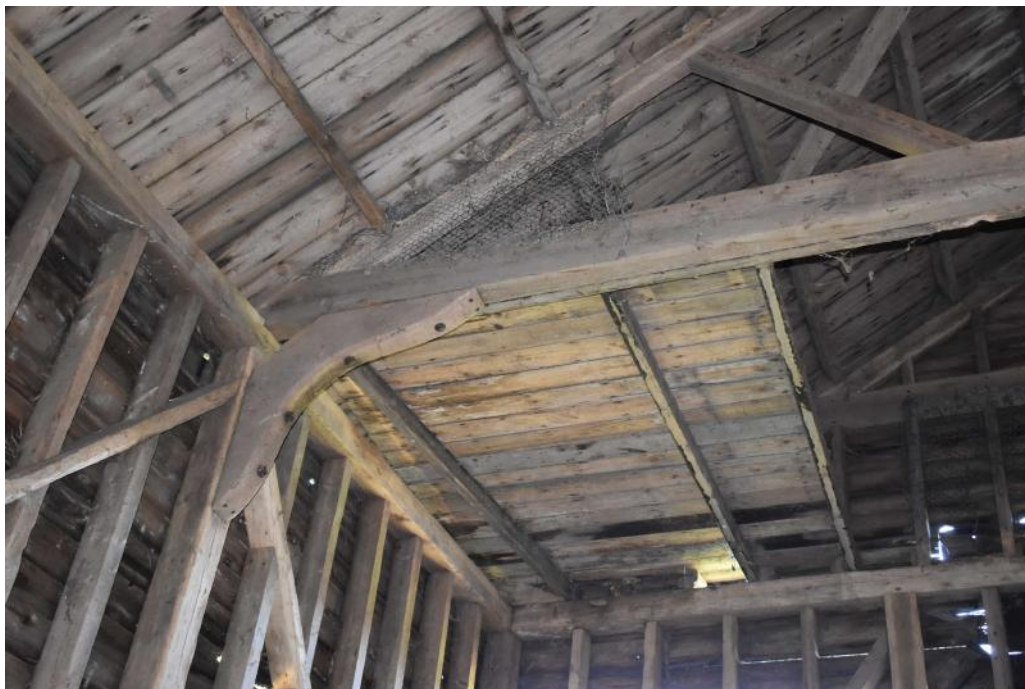
Photograph 17 Detail of inserted loft level in bay 5 of barn. Photograph taken facing north.
