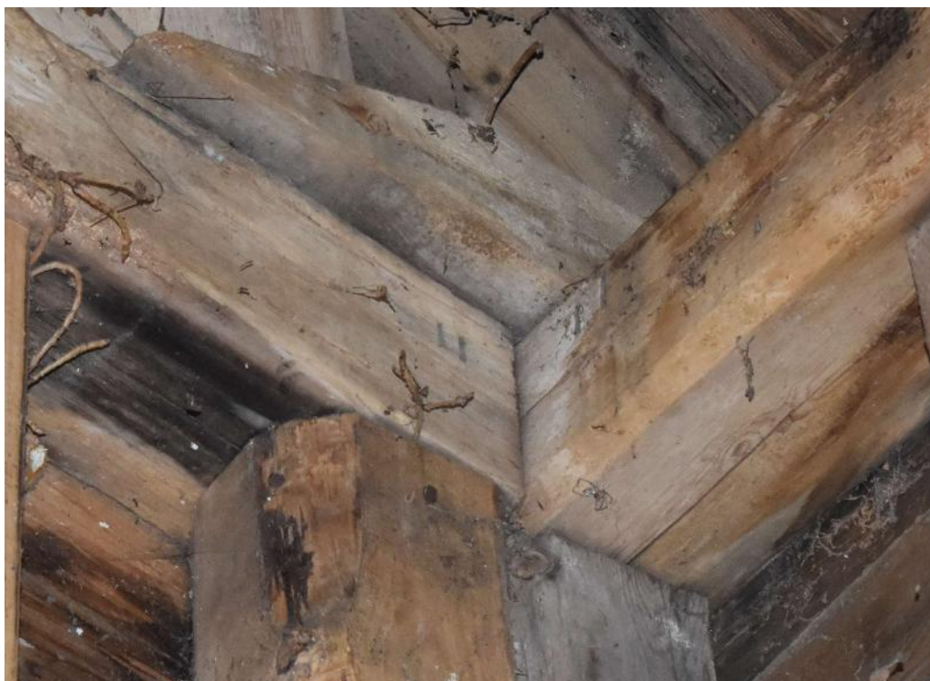
Photograph 13 Detail of carpenters' mark 'II' on gable-tie and wall-plate in north-west corner of bay 1 in barn. Photograph taken facing north.
