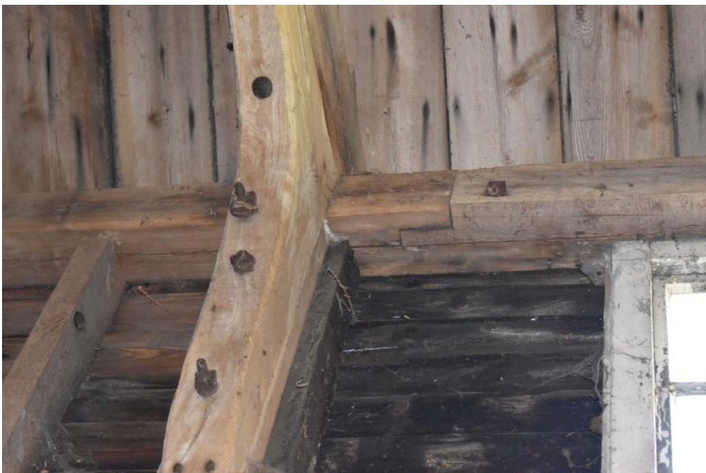
Photograph 15 Detail of scarf-joint in wall-plate of western wall of bay 3 of barn. Photograph taken facing south-west.
