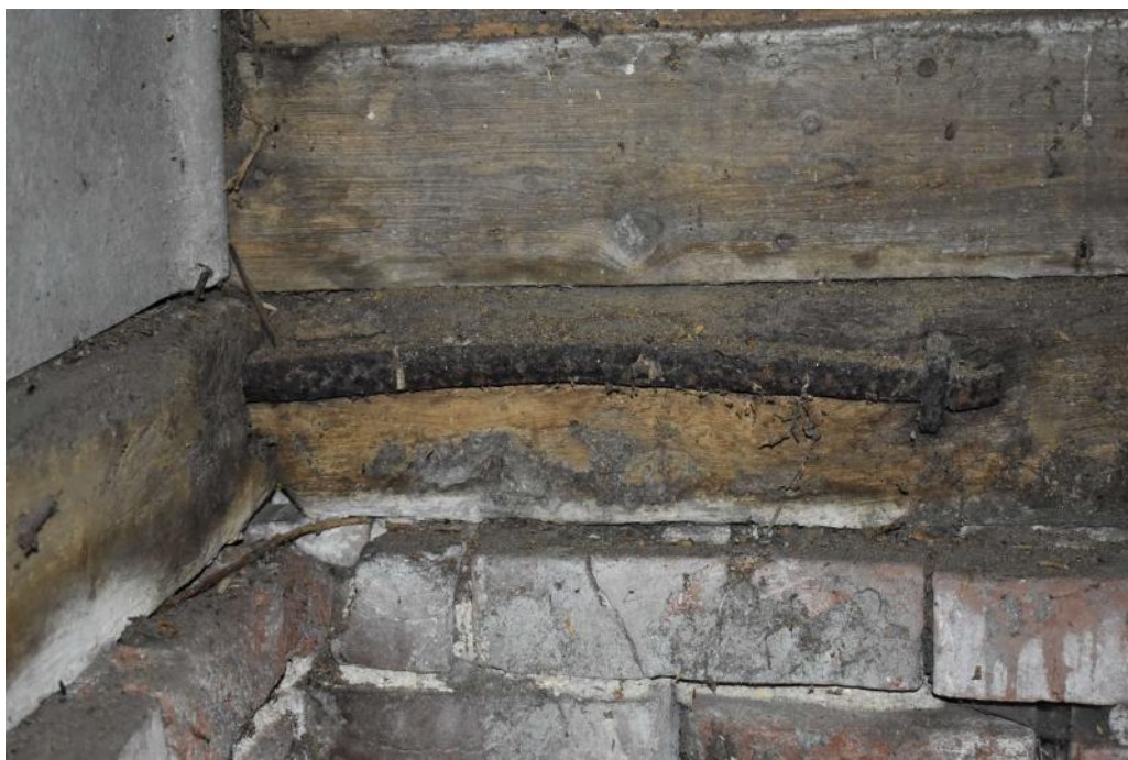
Photograph 18 Detail of iron strap on sill-beam of northern wall of bay 5 of barn. Photograph taken facing north.
