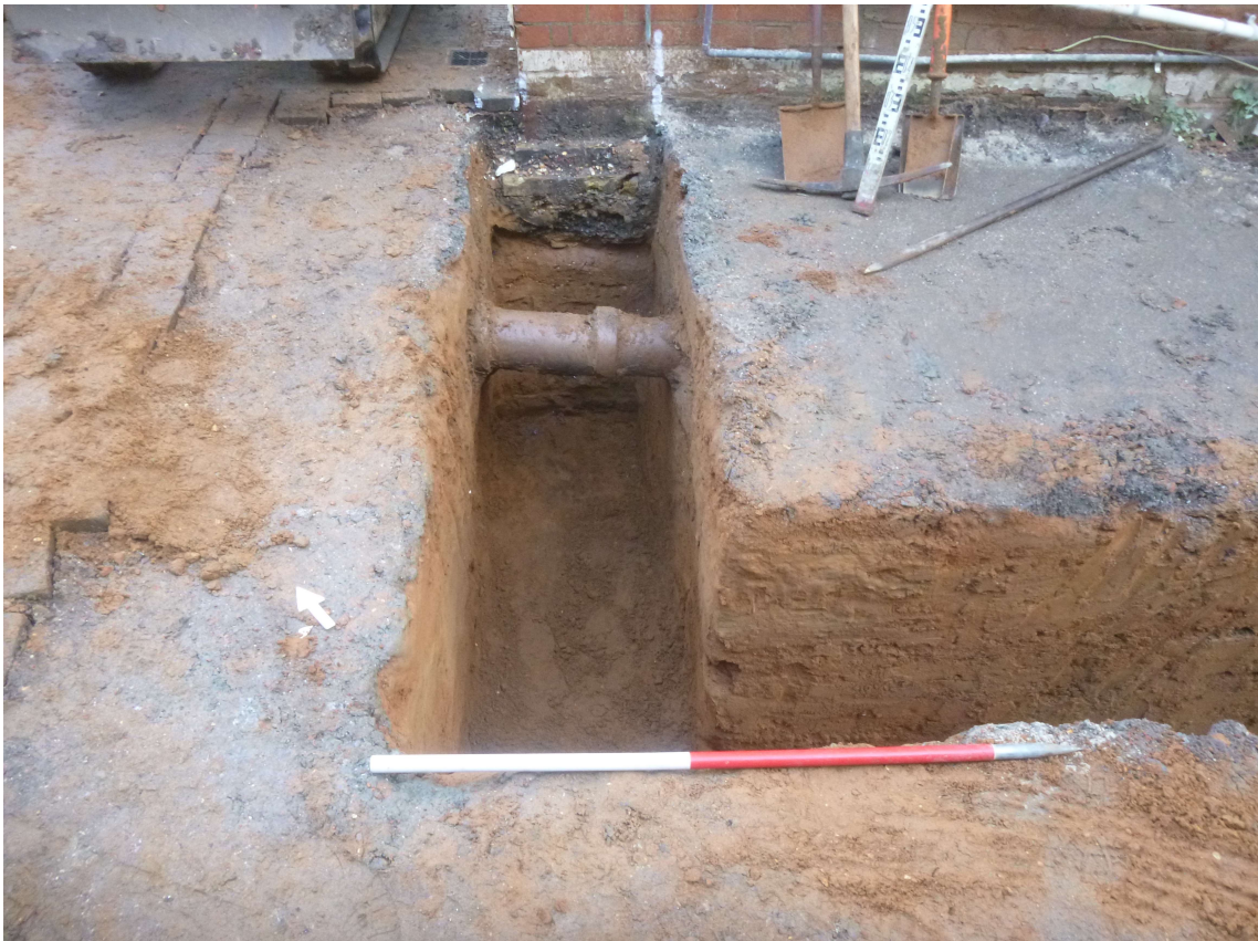
Photograph 1 Foundation trench, view north-east. Note patio tiles laying directly onto L1 to the left.
