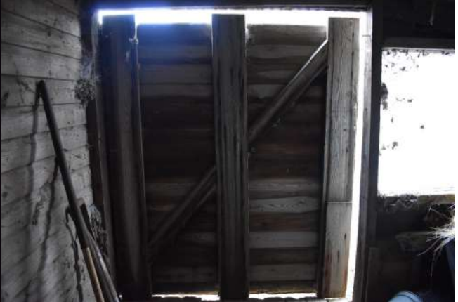
GEAGE23_PhotoGraph_062.JPG Detail of window in northern wall of extension 1. Photograph taken facing north-west.
