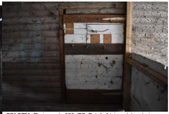
GEAGE23_PhotoGraph_056.JPG Detail of internal door betw een sectional timber hut and extension 1. Photograph taken facing south-w est.
