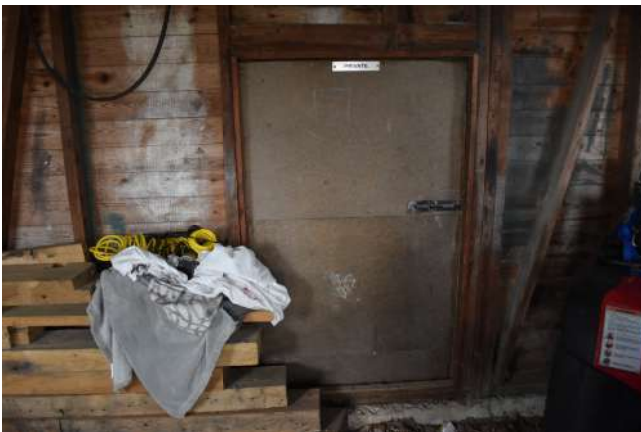
GEAGE23_Photograph_047.JPG Detail of internal door in eastern wall of sectional timber hut. Photograph taken facing north-east.
