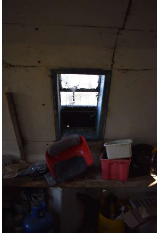
GEAGE23_PhotoGraph_014.JPG Detail of window on northern wall of the handcraft hut. Photograph taken facing north-w est.
