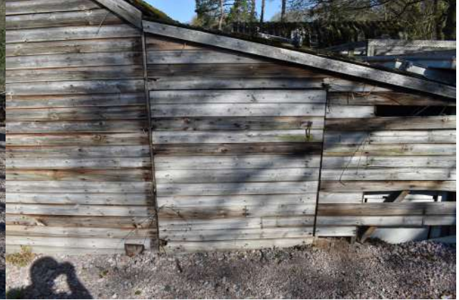
GEAGE23_Phograph_034.JPG Detail of doorway on southern elevation of modern extension of sectional timber hut. Photograph taken facing north-w est.
