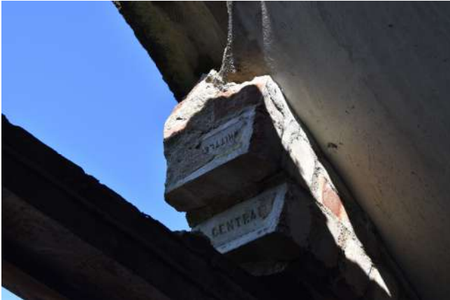
GEAGE23_Photo graph_021.JPG Detail of bricks above door of western wall of the handcraft hut. Photo graph taken facing west.
