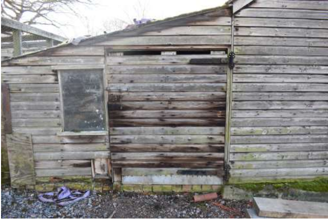
GEAGE23_PhotoGraph_037.JPG Detail of doorway on northern elevation of modern extension of sectional timber hut. Photograph taken facing south-east.
