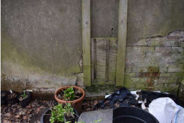
GEAGE23_PhotoGraph_065.JPG Detail of poultry door betw een extension 1 and 3. Photograph taken facing south-w est.
