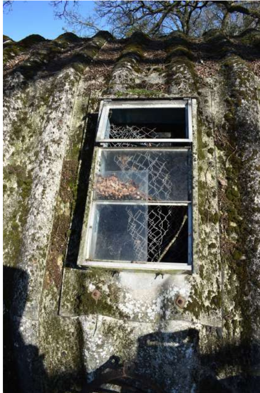
Photograph 7 Detail of window on southern elevation of the handcraft hut. Photograph taken facing north-west.
