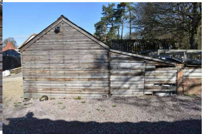
GEAGE23_Photograph_032.JPG Southern elevation of the sectional timber hut. Photograph taken facing north-west.
