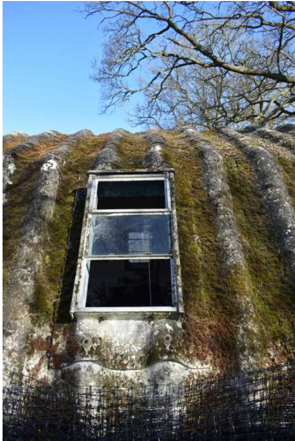
GEAGE23_Phograph_011.JPG Detail of window on southern elevation of the handcraft hut. Photograph taken facing north-west.
