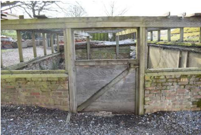
GEAGE23_PhotoGraph_039.JPG Detail of doorway on northern elevation of modern extension to sectional timber hut. Photograph taken facing south-east.
