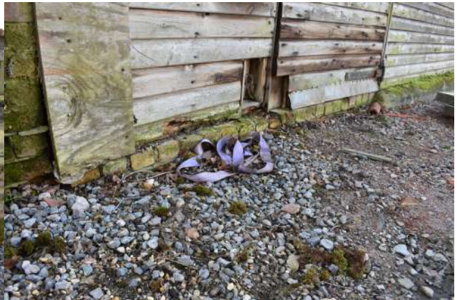
GEAGE23_PhotoGraph_040.JPG Detail of brick plinth on northern elevation of modern extension of sectional timber hut. Photograph taken facing south.
