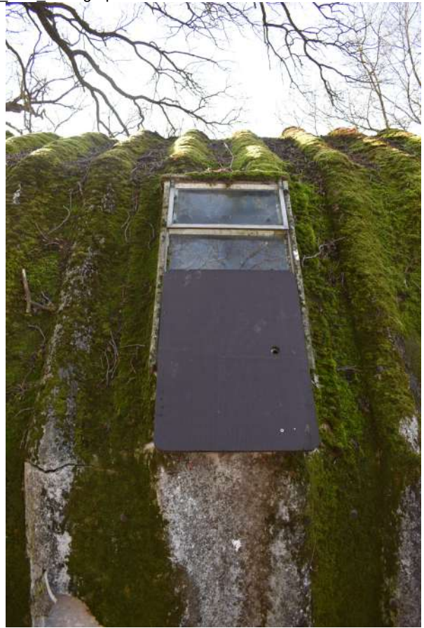
GEAGE23_Photograph_006.JPG Detail of window on northern elevation of the handcraft hut. Photograph taken facing south-east.
