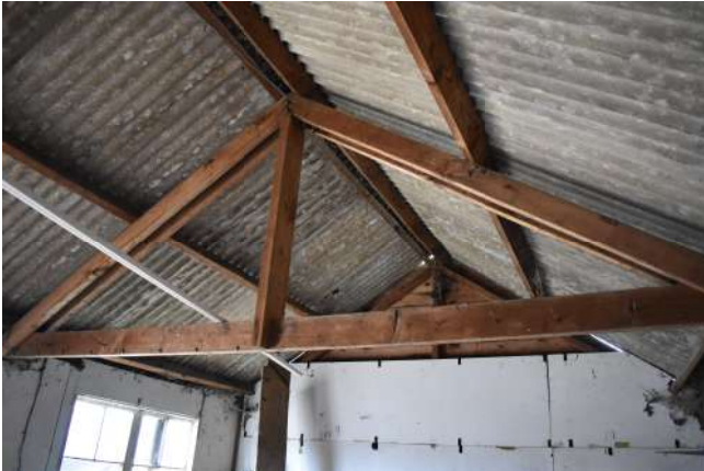
GEAGE23_PhotoGraph_049.JPG Detail of truss in sectional timber hut. Photograph taken facing north-w est.
