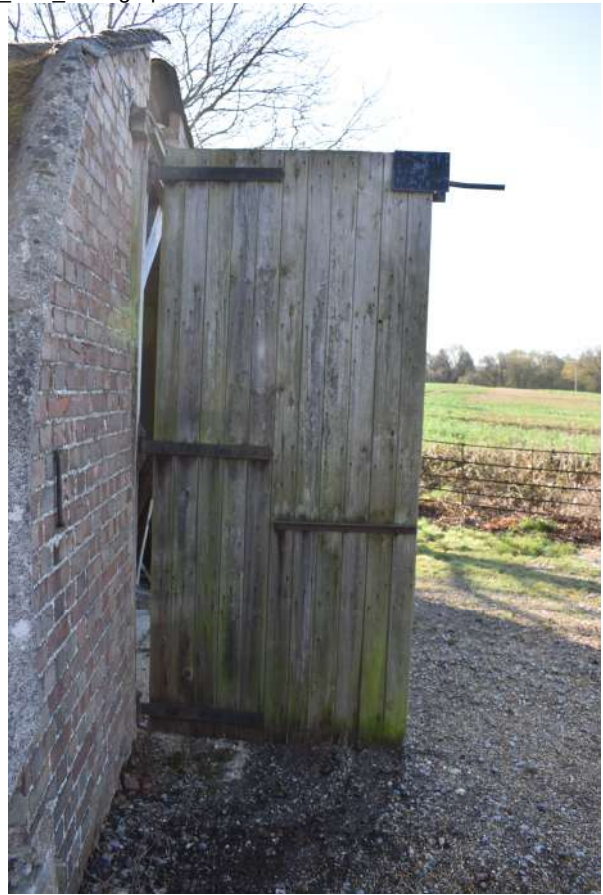
GEAGE23_PhotoGraph_002.JPG Detail of door on western elevation of the handcraft hut. Photograph taken facing south-east.
