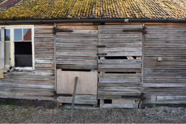
GEAGE23_Photograph_029.JPG Detail of doorway on western elevation of the sectional timber hut. Photograph taken facing north-east.
