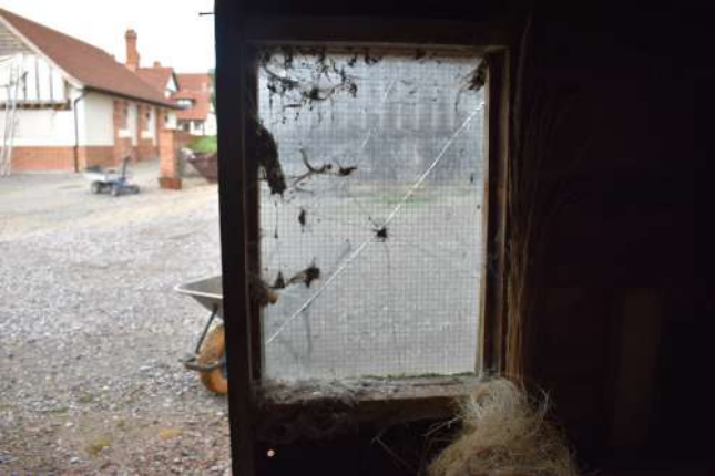
GEAGE23_PhotoGraph_061.JPG Detail of window of northern wall of extension 1. Photograph taken facing north-west.
