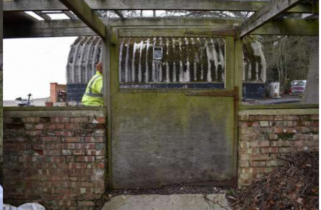
GEAGE23_PhotoGraph_066.JPG Detail of door in northern wall of extension 3. Photograph taken facing north-w est.
