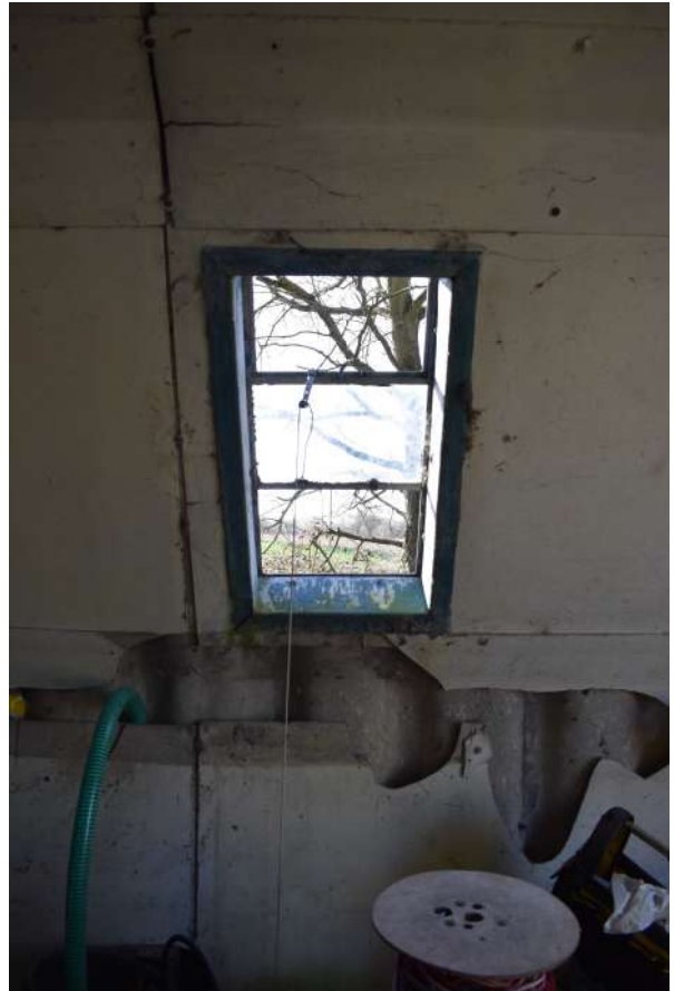
GEAGE23_PhotoGraph_016.JPG Detail of window on southern wall of the handcraft hut. Photograph taken facing south-east.
