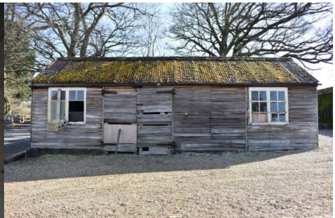
GEAGE23_PhotoGraph_028.JPG Western elevation of the sectional timber hut. Photograph taken facing north-east.
