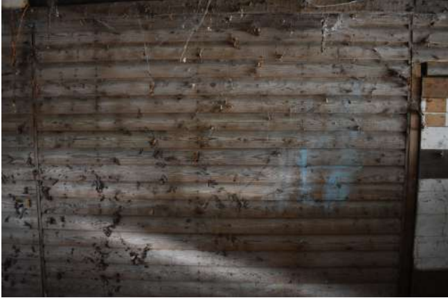
GEAGE23_PhotoGraph_057.JPG Detail of original exterior w all of sectional timber hut w ithin extension 1. Photograph taken facing south-w est.
