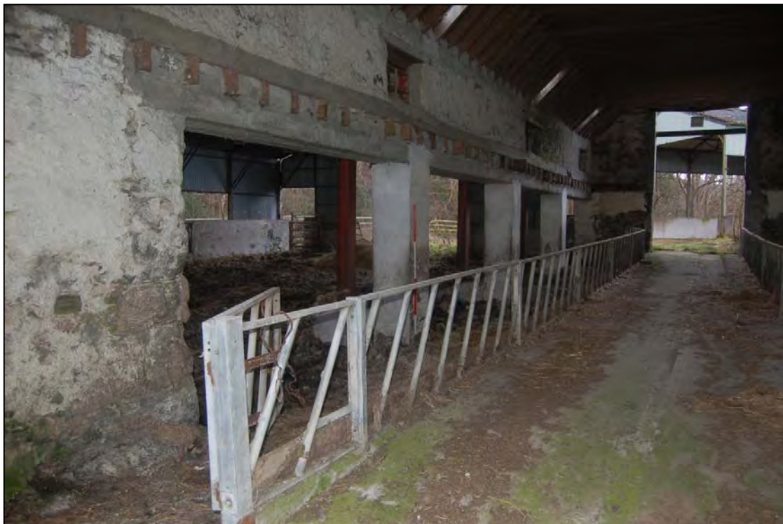
Plate 17 House 7, interior E elevation, showing replacement concrete pillars to carry upper wall and roof
