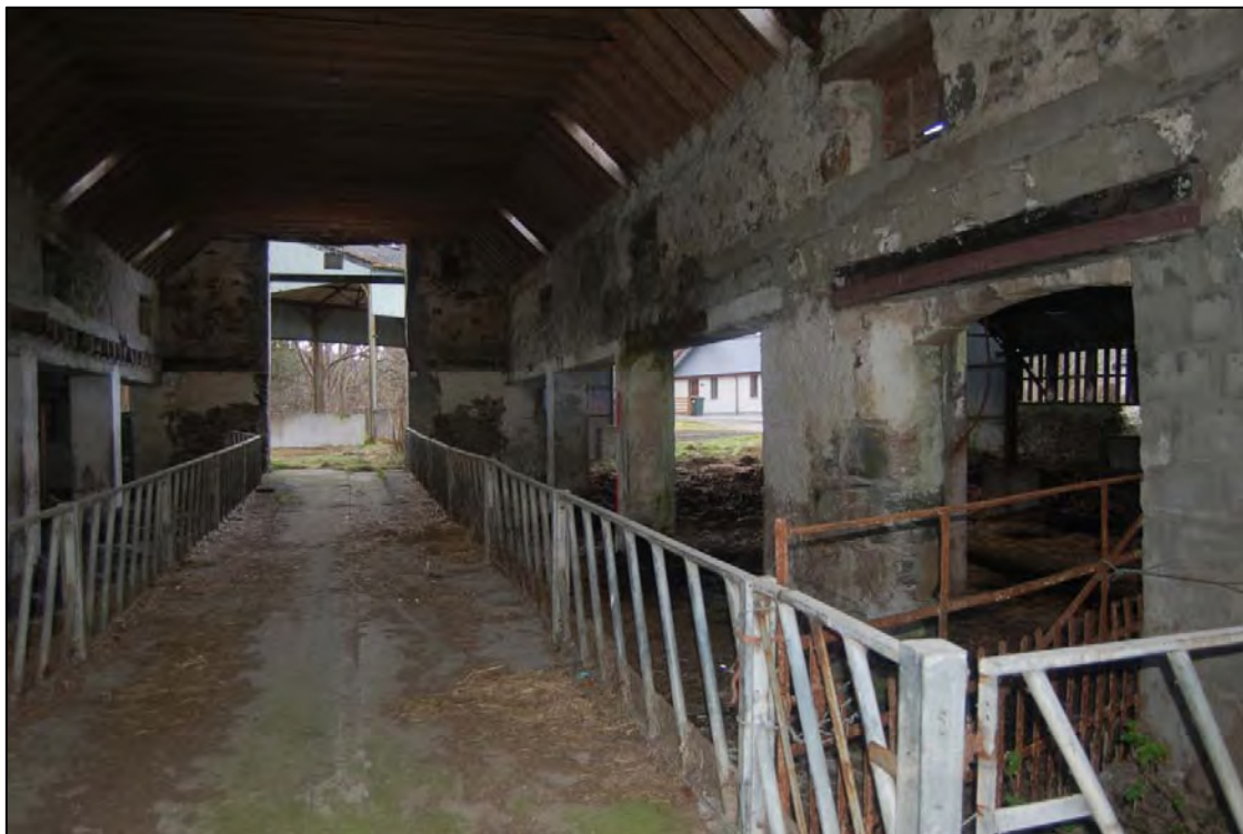
Plate 18 House 7, internal view of W elevation, showing replacement concrete lintels over openings
