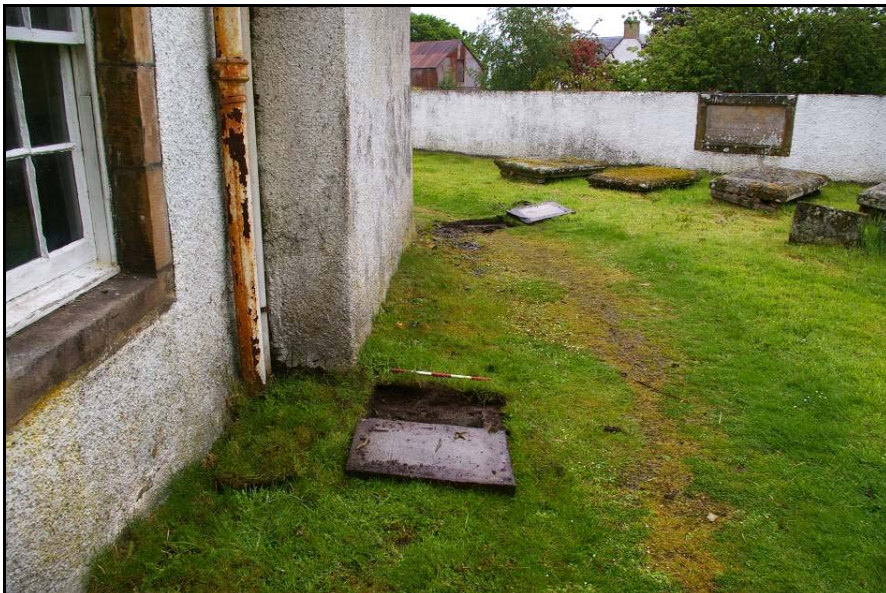
Figure 15 Drain covers lifted outside E wall of church.
