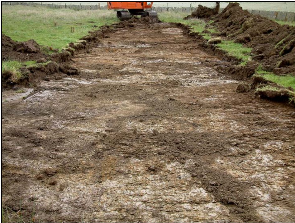
12: Stripping for septic tank and soakaway (Photo 8) Location and direction shown as No. 8 on site plan above
