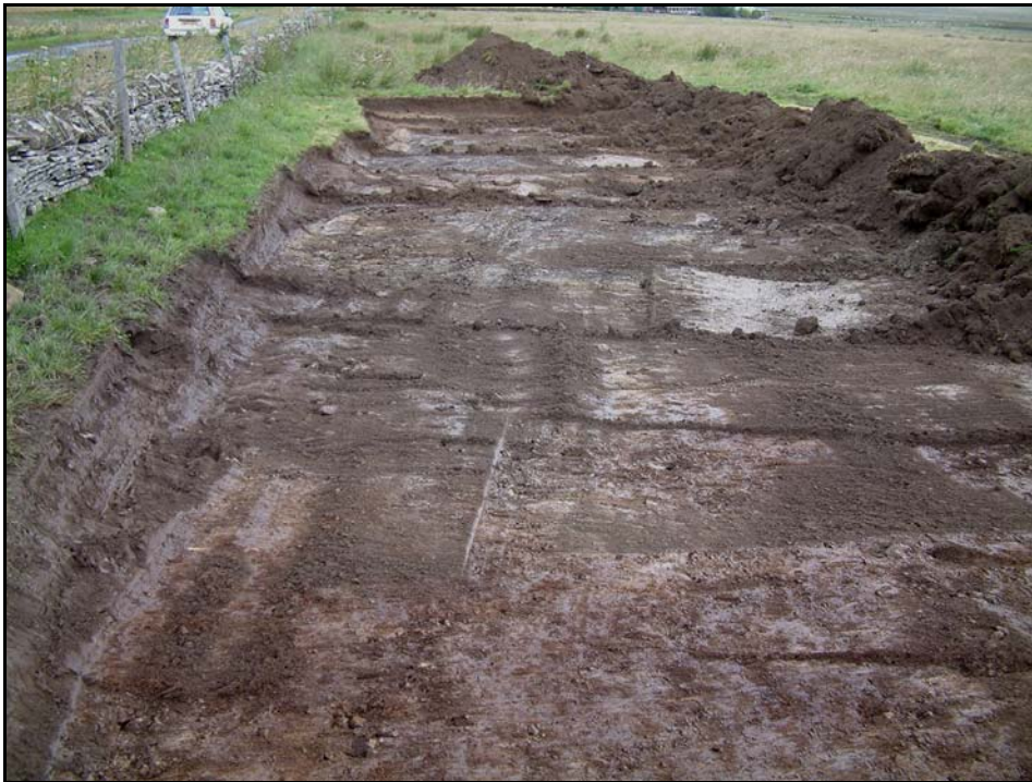
8: Site stripping in progress: hard standing and shed area (Photo 4) Location and direction shown as No. 4 on site plan above
