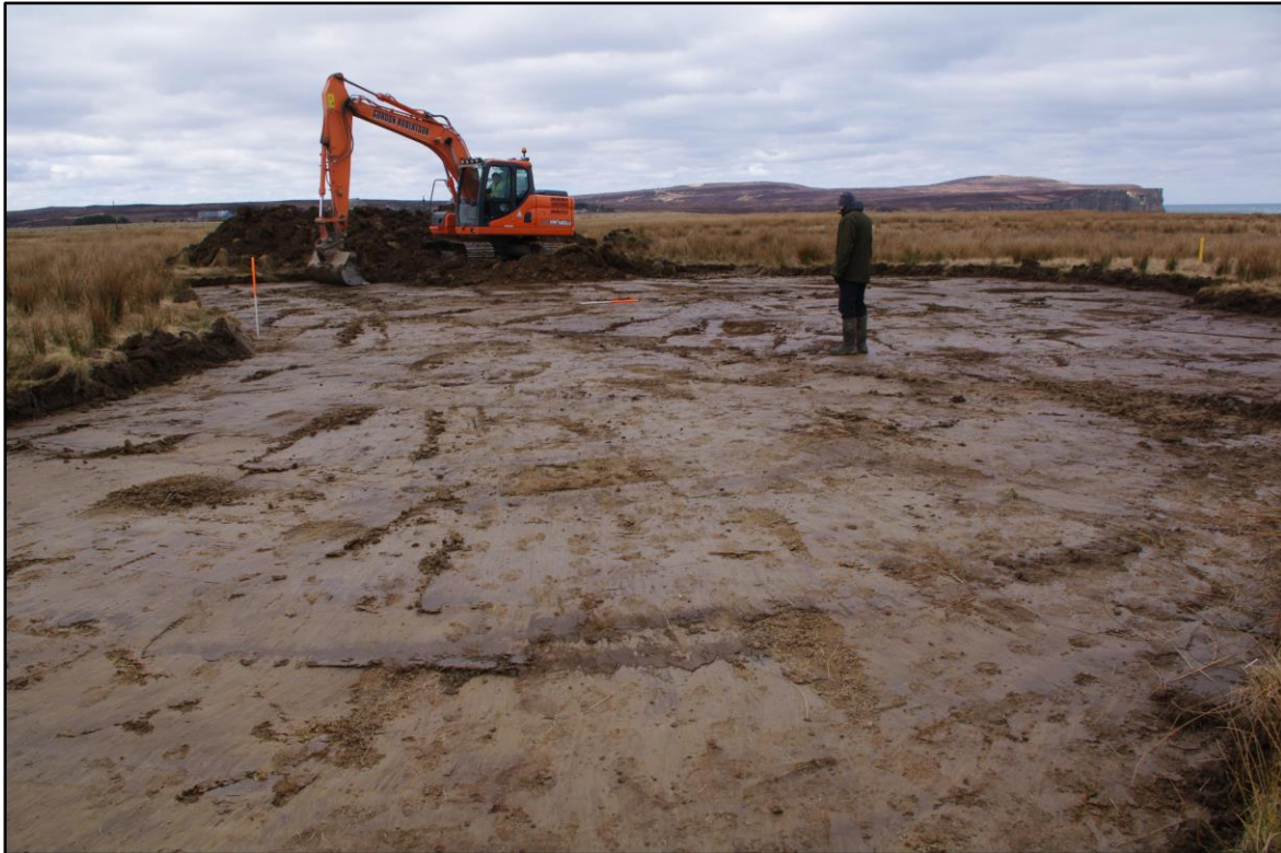
Figure 7: The topsoil stripping area nearing completion. Facing NW from CP2. Scales 1m
