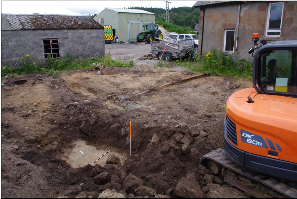
Figure 11 – Cutting in Soakaway Deposit (106) also showing modern waste pipes. Facing S. Scales 1m
