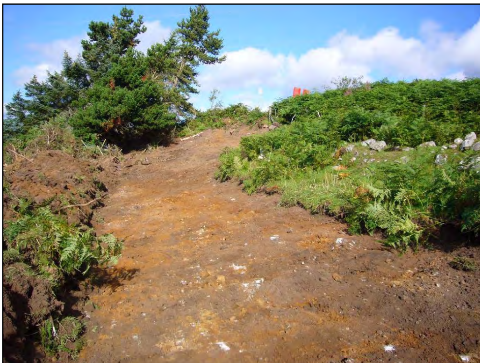
Plate 3 Ground clearance for the new access road into the site. Remains of the stone boundary dyke can be seen to the top right of the picture
