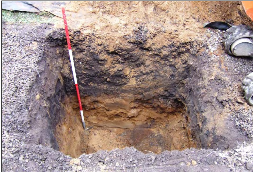
Plate 3 Soakaway in churchyard
