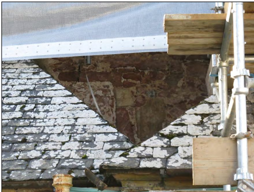
Plate 10 Evidence of blocked 16 th c. window in E gable, largely hidden by E porch and vestry
