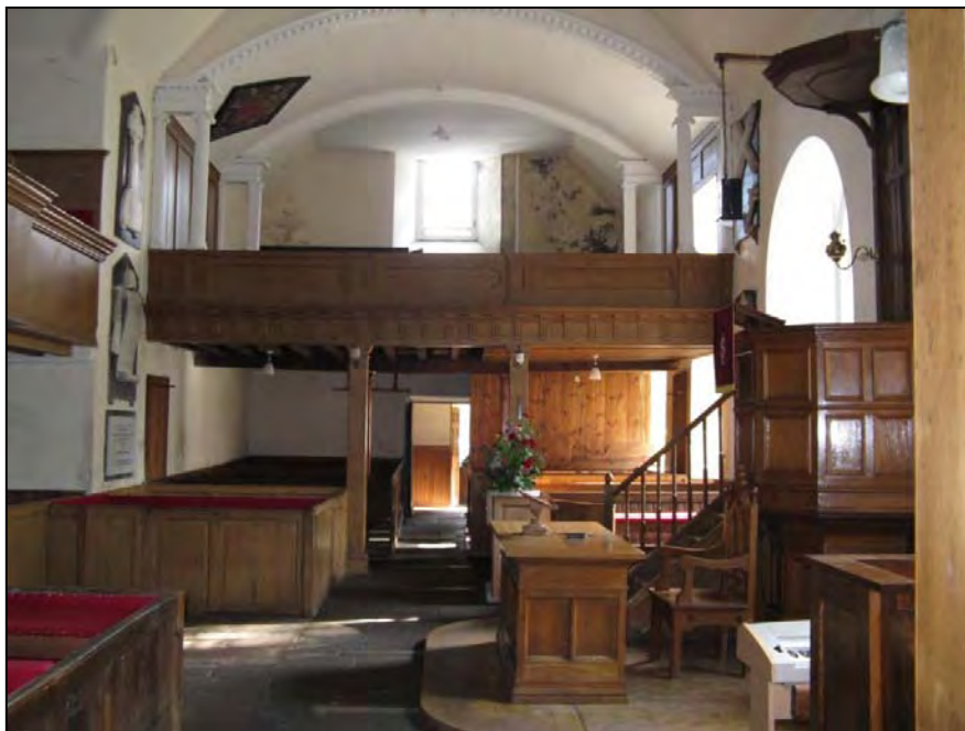
Plate 2 Interior before project started: damp in east gable
