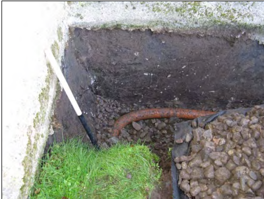
Plate 1 Corner of E wall and E porch, by door, showing bitumen, cement harl and perforated pipe drainage as found
