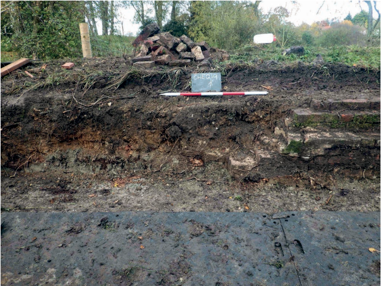
Plate 5: Missing section at western end of dam wall
