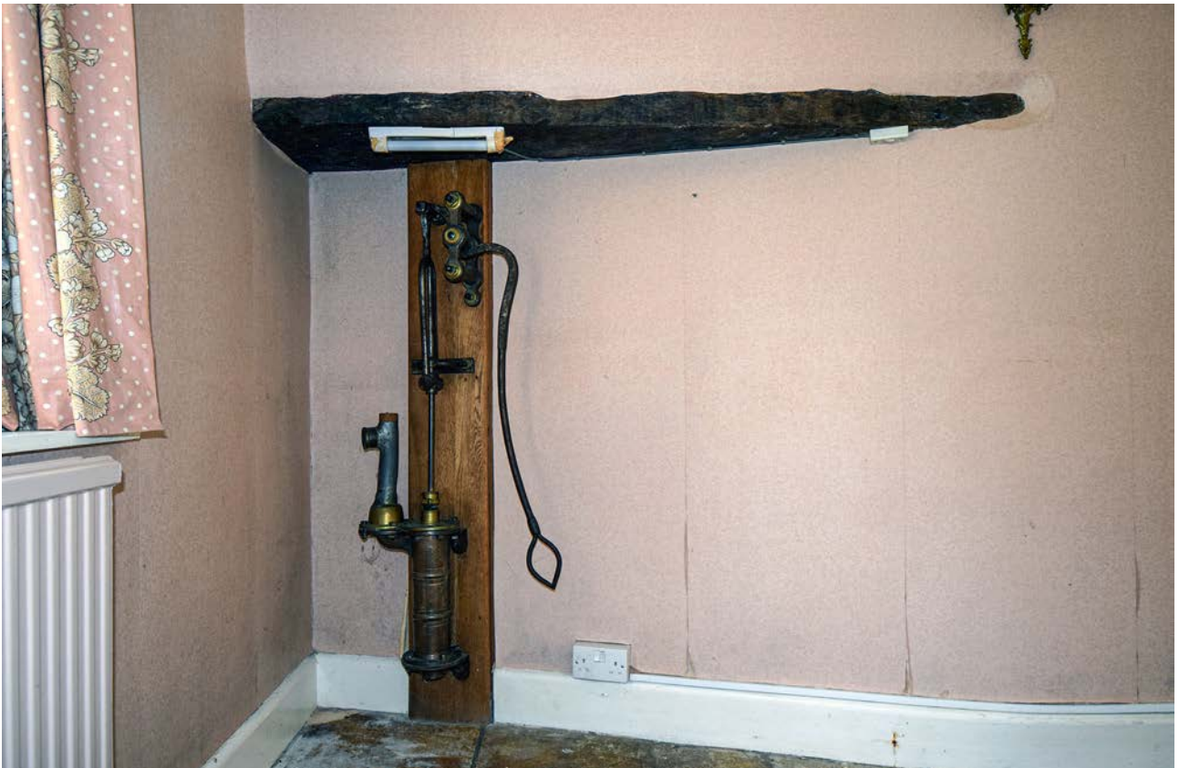
Plate 19: The water pump in the north-east corner of the dining room, looking north-east
