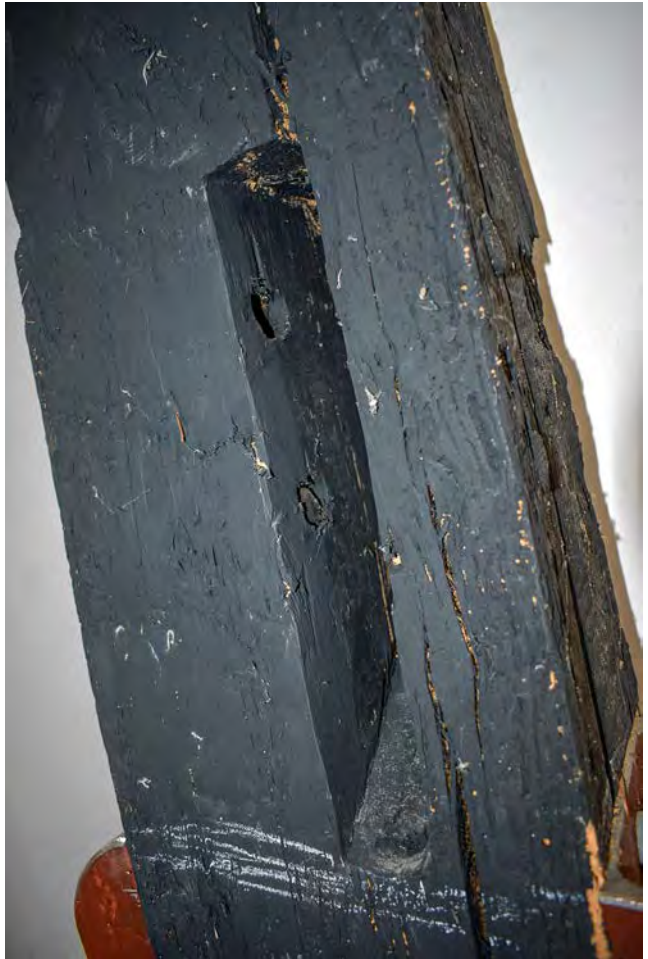
Plate 39: Empty mortise in the truss in the attic corridor, looking south-west
