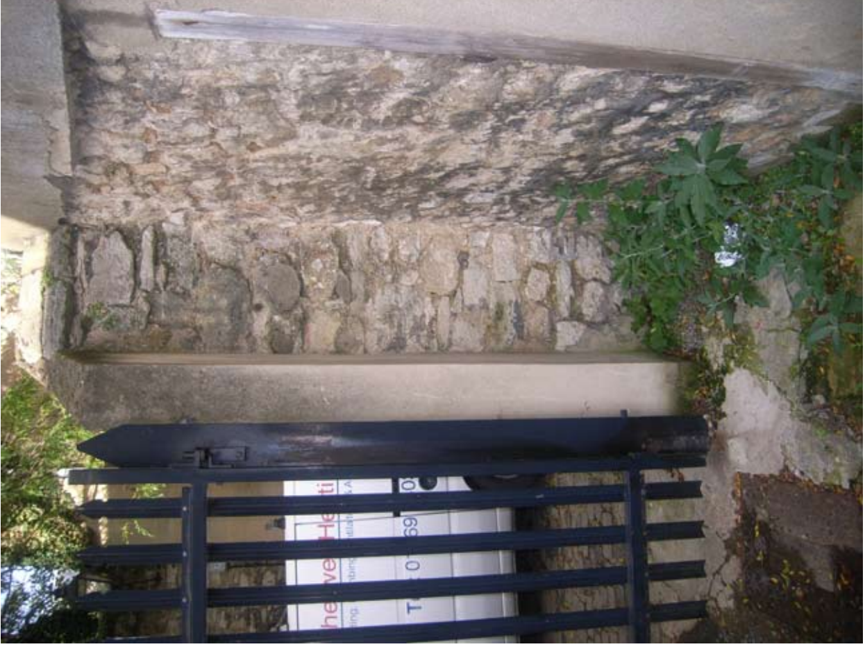
Plate 24: South face of nib of wall to east of 6 Brewer Street
