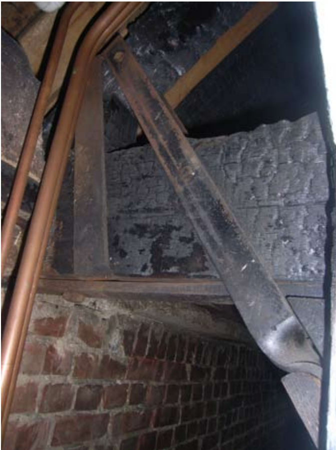
Plate 15: Charred north end of tie-beam in 6 Brewer Street.
